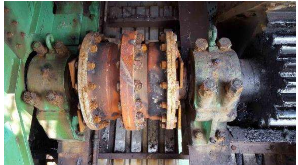
Bascule span coupler
