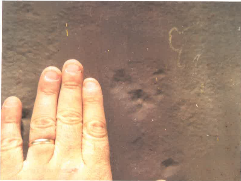
Photograph 26 -- Previous Pitting on the Lift Span Girder Web
