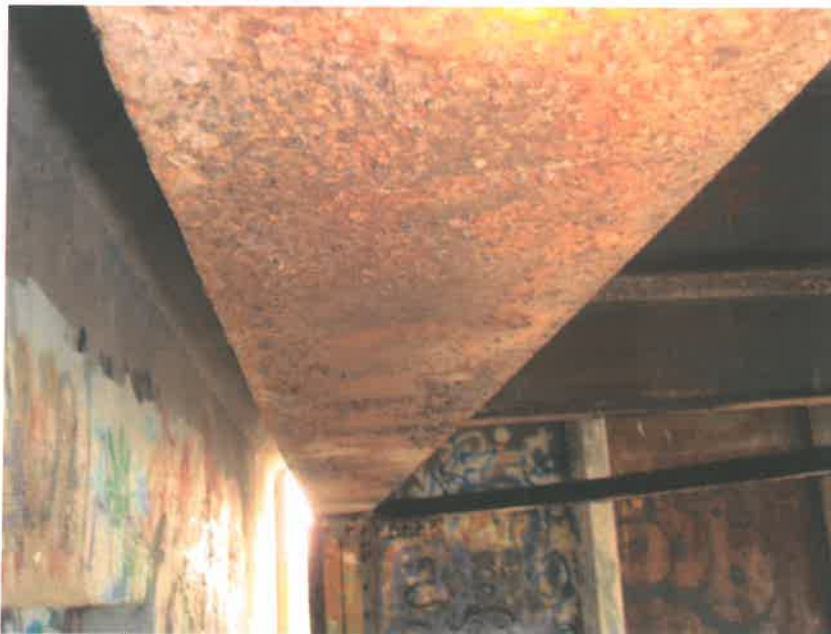
Photograph 8 – Corrosion on the Underside of the Bottom Flange of End Floorbeam
