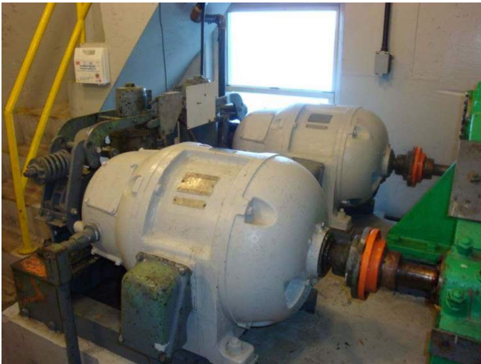
Photo M-02, The steel mounting brackets for the motors and brakes have scattered areas of paint loss and light corrosion. View of motor room looking north.
