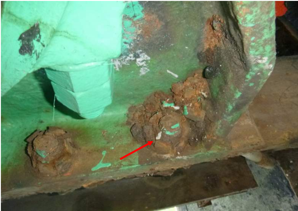
Photo M-05: The open gear housing and bearing fasteners are corroded with varying degrees of section loss.
