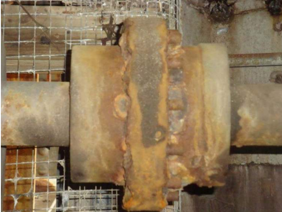
Photo M-13, The emergency drive output coupling has complete paint loss and corrosion. Fasteners are corroded and the lubrication appears dry.
