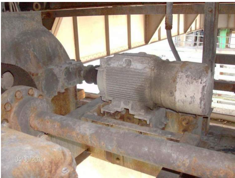
Photo M-18, The span lock motor grease fittings appeared dry and the motor frame and had complete paint loss and light corrosion.
