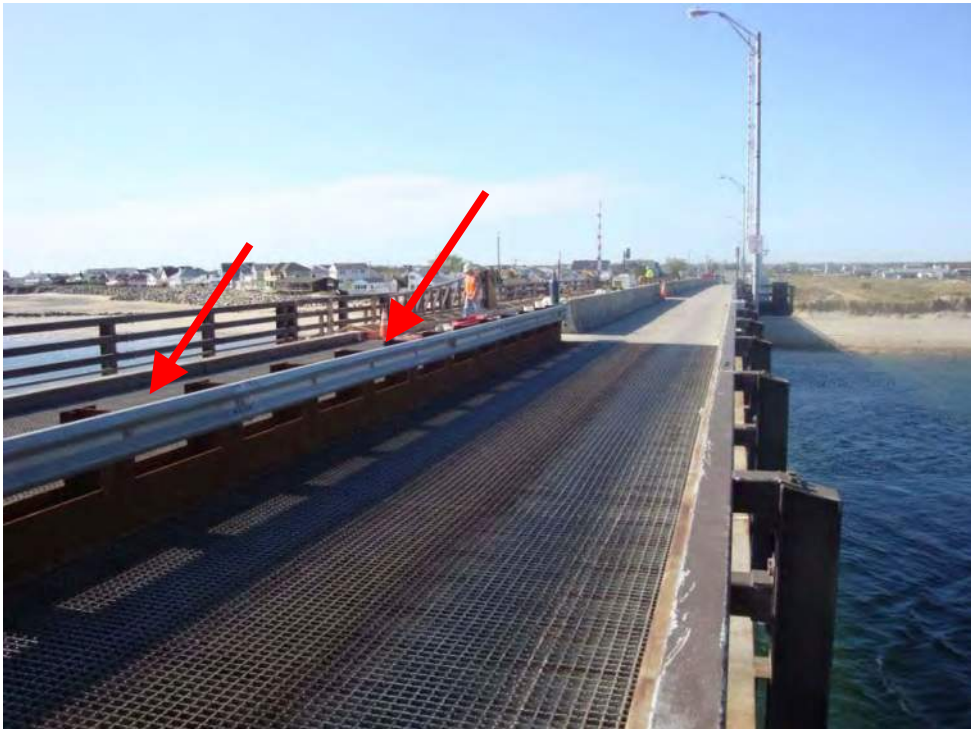
Photo M-24, A steel center divider has been added to the movable span since the previous inspection.
