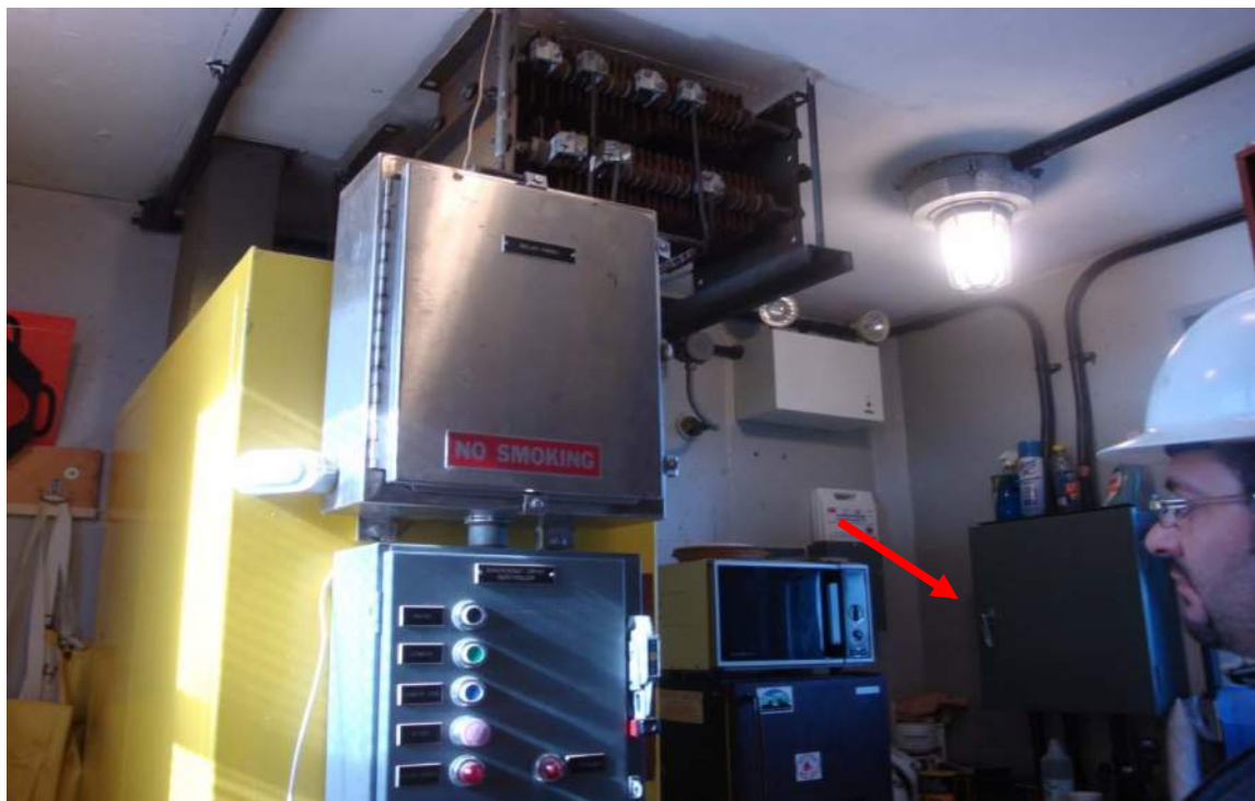
Photo E-18, 120/240 volts, 40 amp lighting panel.
