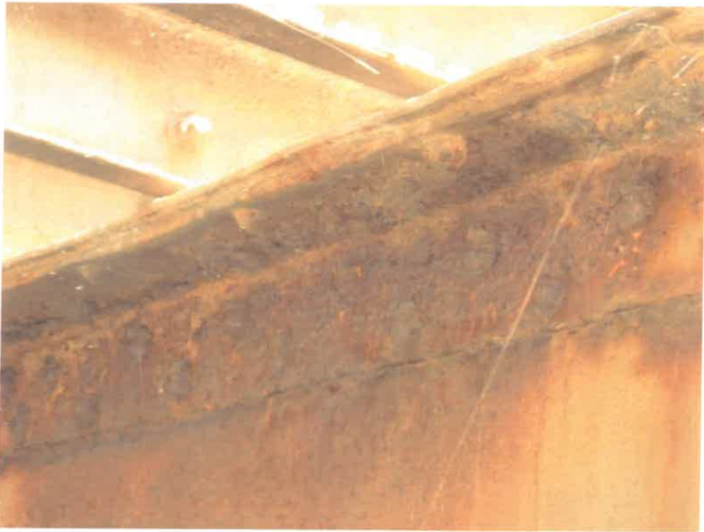
Photograph 22 – Corrosion at Girder Top Flange
