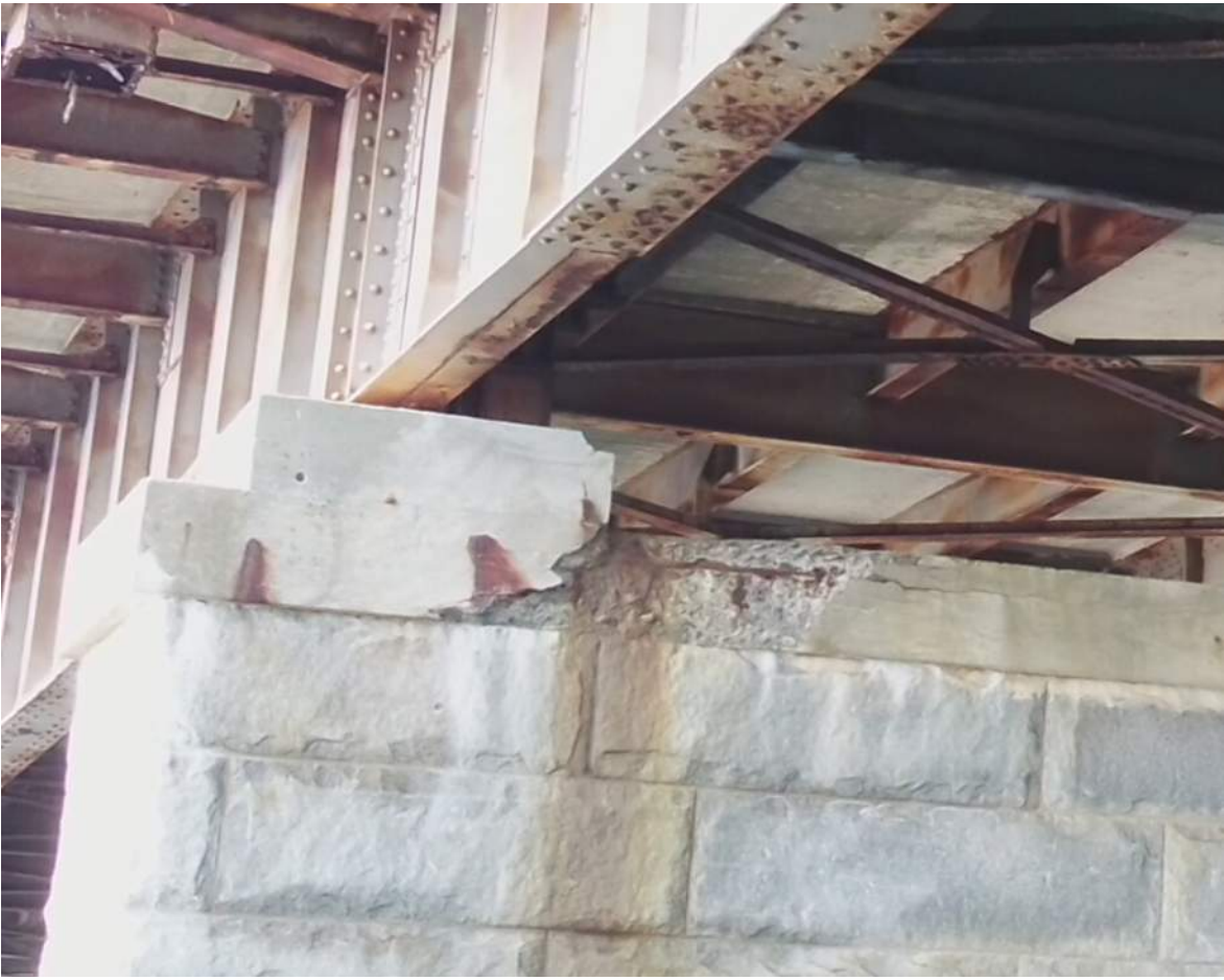
Photo S-23: Deteriorated pier cap at Pier 4N.
