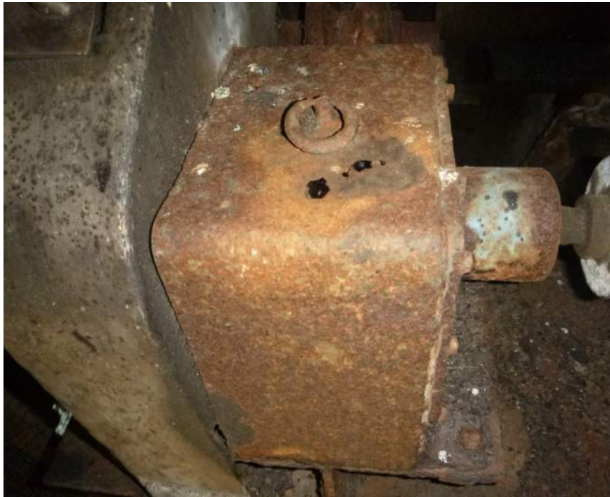
Photo M-07: The outside of the enclosed reducer is corroded and the mount is in poor condition.
