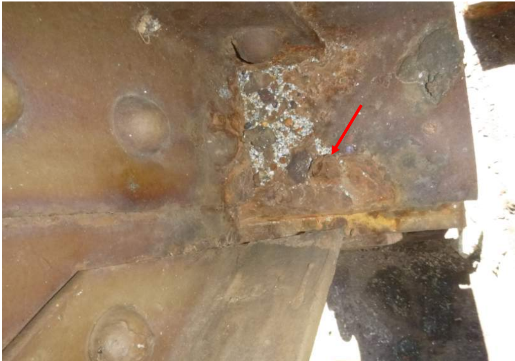
Photo M-18: The live load shoe rivets exhibit severe corrosion and section loss.
