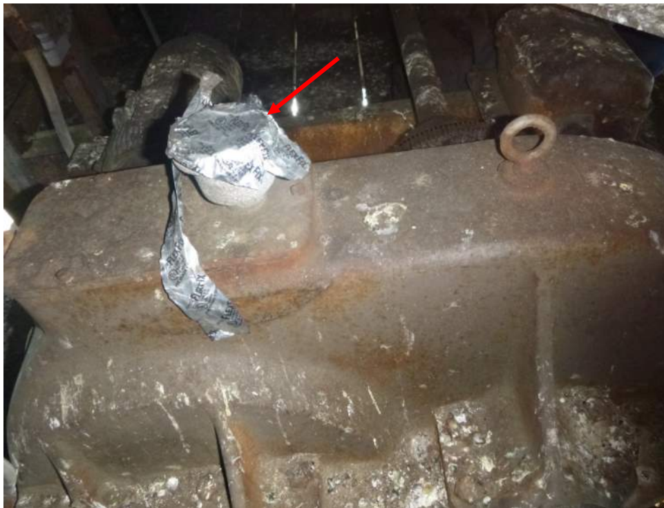
Photo M-10: The breather on the span lock reducer is clogged and covered with tape.
