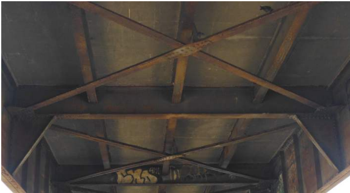
Photo S-12: Approach span floor beam and cross bracing typical condition.
