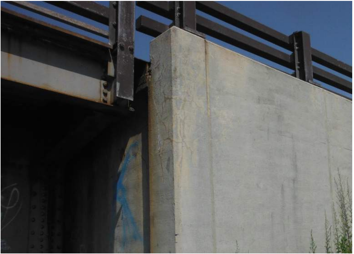
Photo S-19: Cracks and efflorescence at northeast wingwall.
