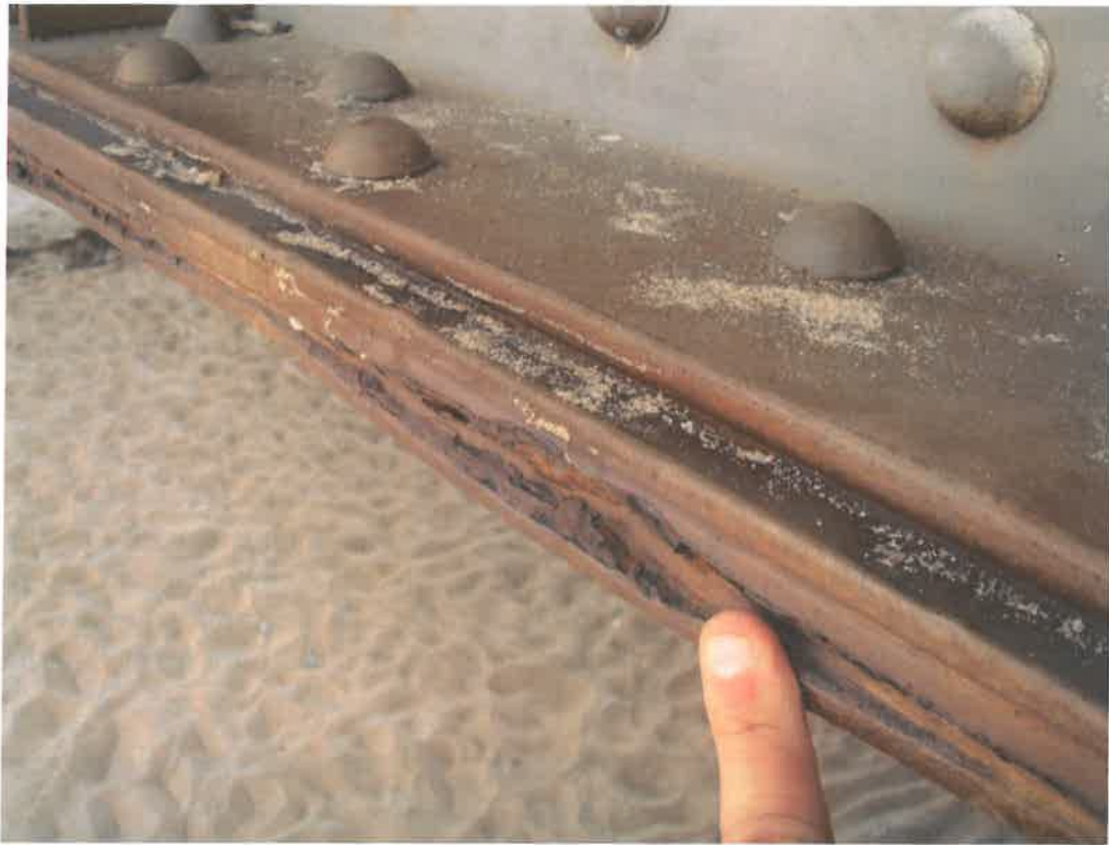
Photograph 5 – Area of Pack Rust at Girder Bottom Flange
