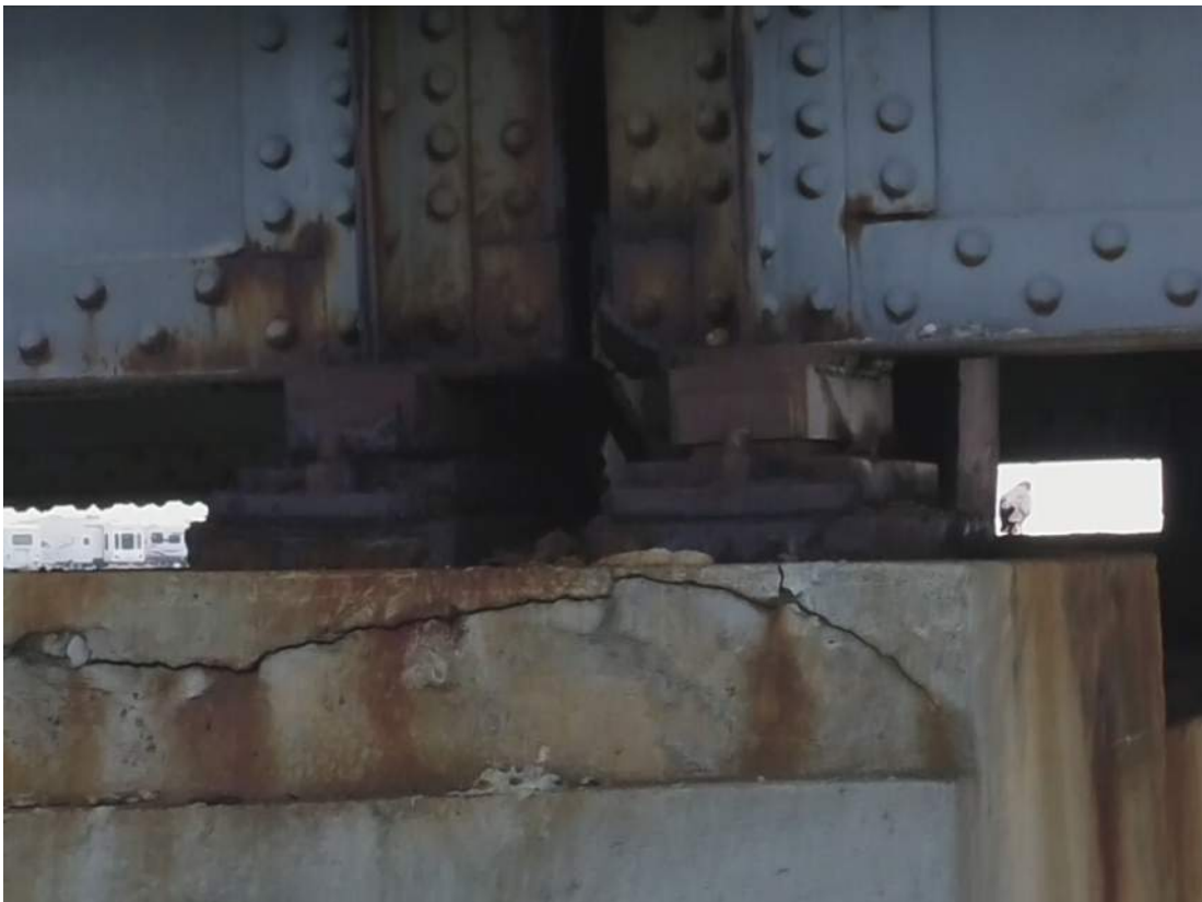
Photo S-14: Severely corroded bearings at Pier 4N.
