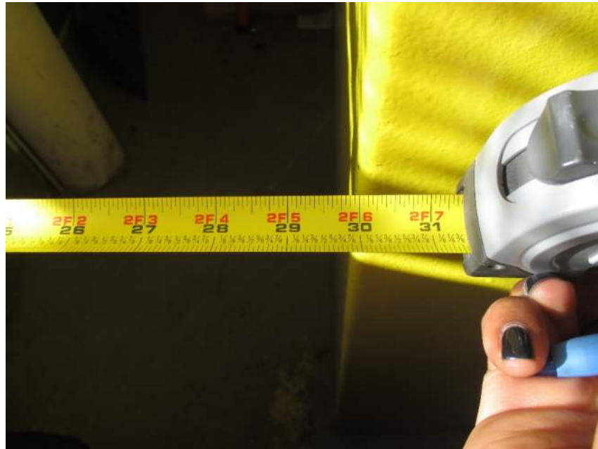
Photo E-03: MCC Insufficient Working Clearance from East Wall
