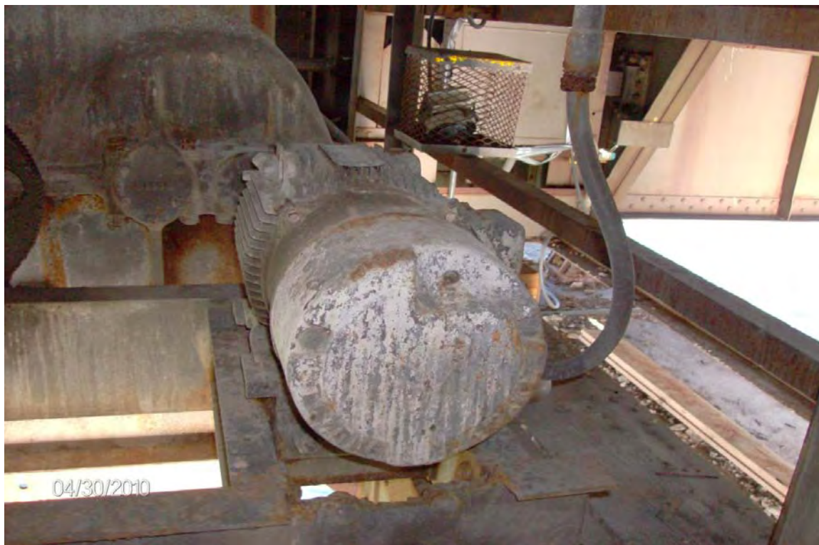
Photo E-14, Span lock motor signs of corrosions.
