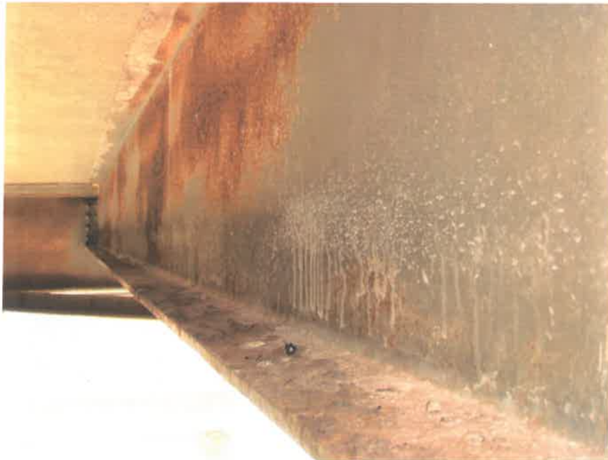
Photograph 10 – Typical Rusting on Stringer Webs
