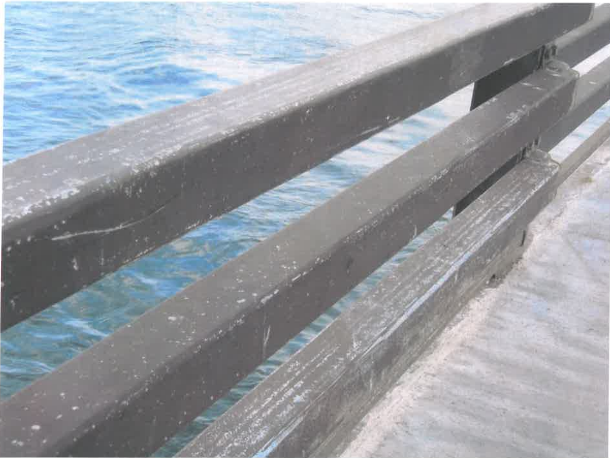
Photograph 15 – Typical Wear of the Topcoat on the Bridge Handrail
