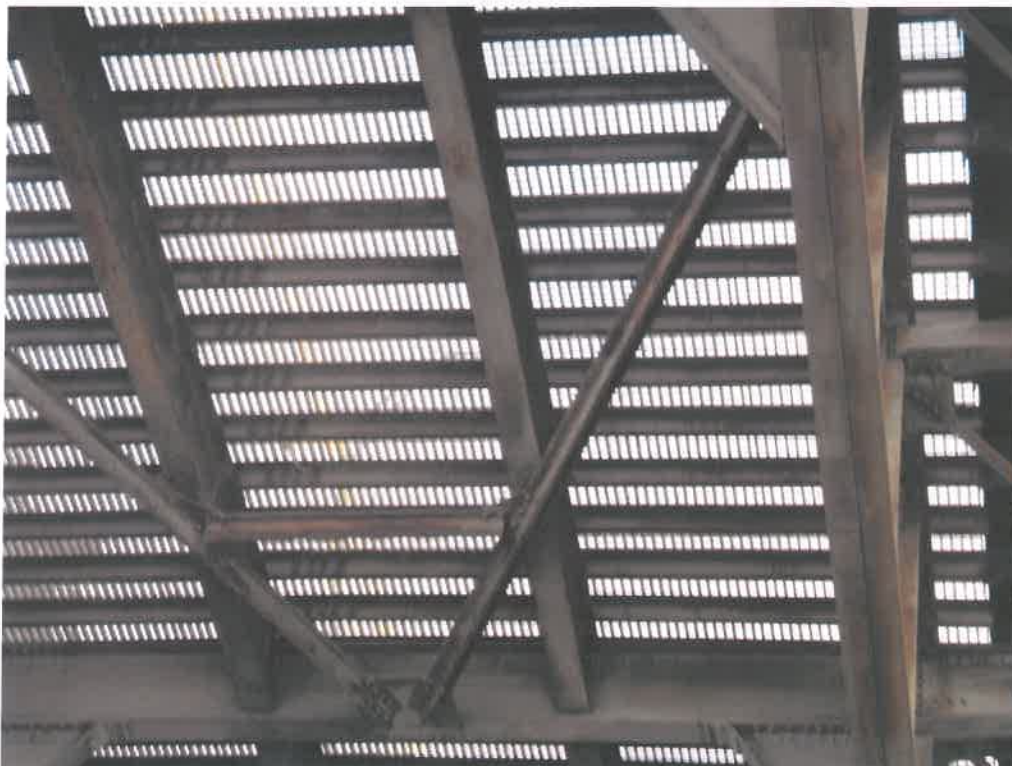
Photograph 17 – Pinpoint Rust on Lift Span Girder, Stringers, and Lateral Bracing
