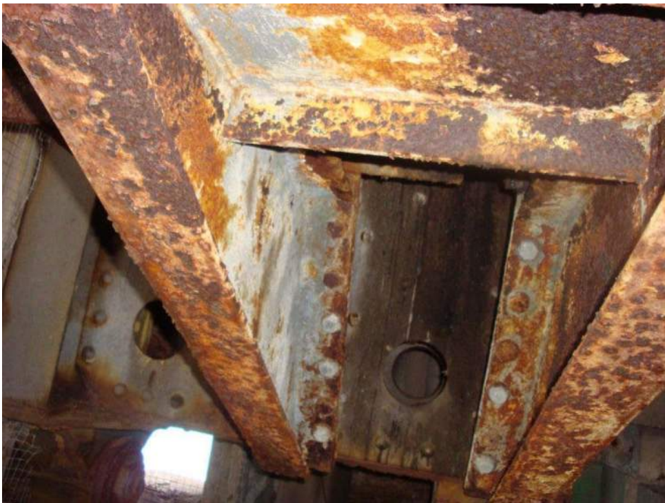
Photo M-10, The emergency drive front machinery support has paint loss and light corrosion.
