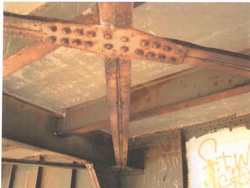
Photograph 12 – Typical Rust on the Underside of the Lateral Bracing
