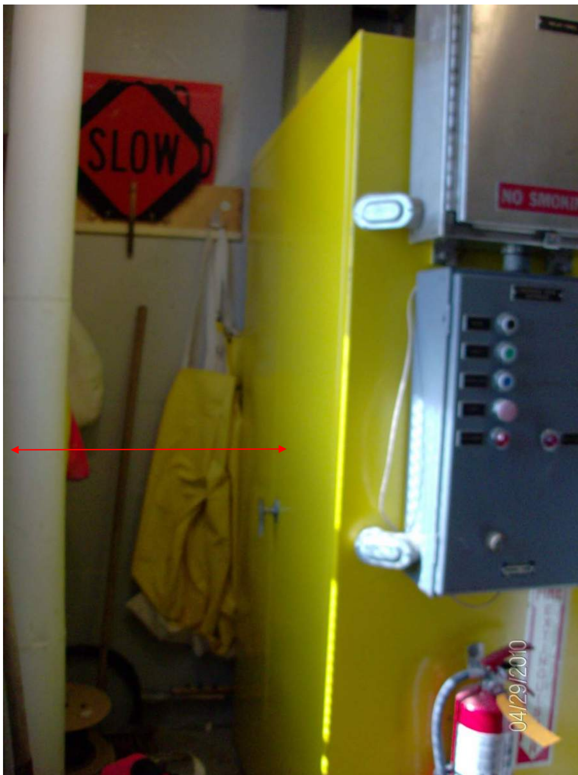
Photo E-04, The rear side of the MCC distance from the wall is less than the NEC requirement for working clearances.
