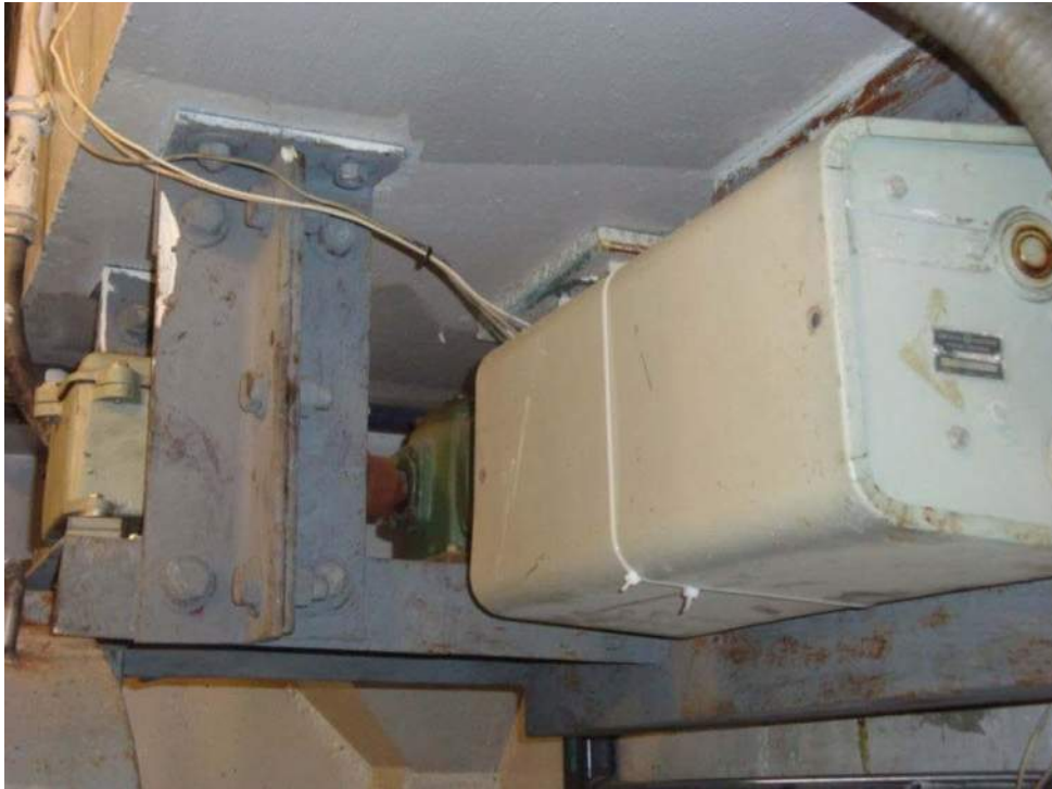
Photo M-17, General Electric rotary cam limit switch and Henschel Corp position transmitter.
