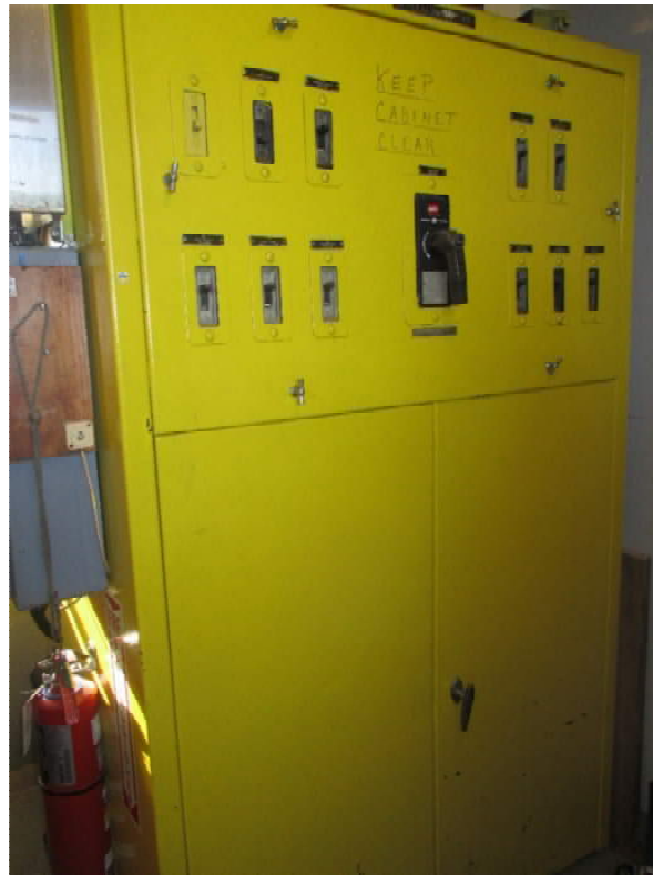
Photo E-01: Motor Control Center (MCC)
