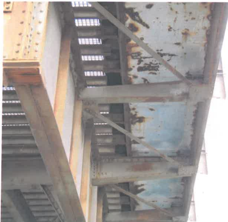
Photograph 19 – Corrosion on Ocean Side Sidewalk Support and Deck Pans
