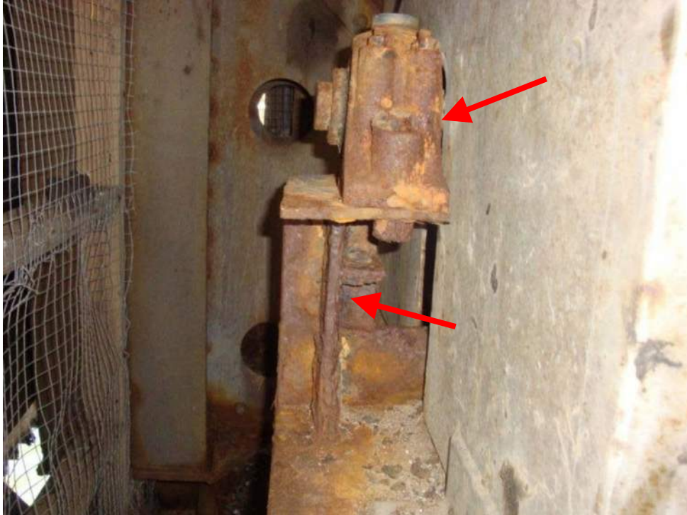
Photo M-15, Bearing block fasteners have near complete head loss due to corrosion. The pillow block bearing pedestals have complete paint loss and sectional loss.
