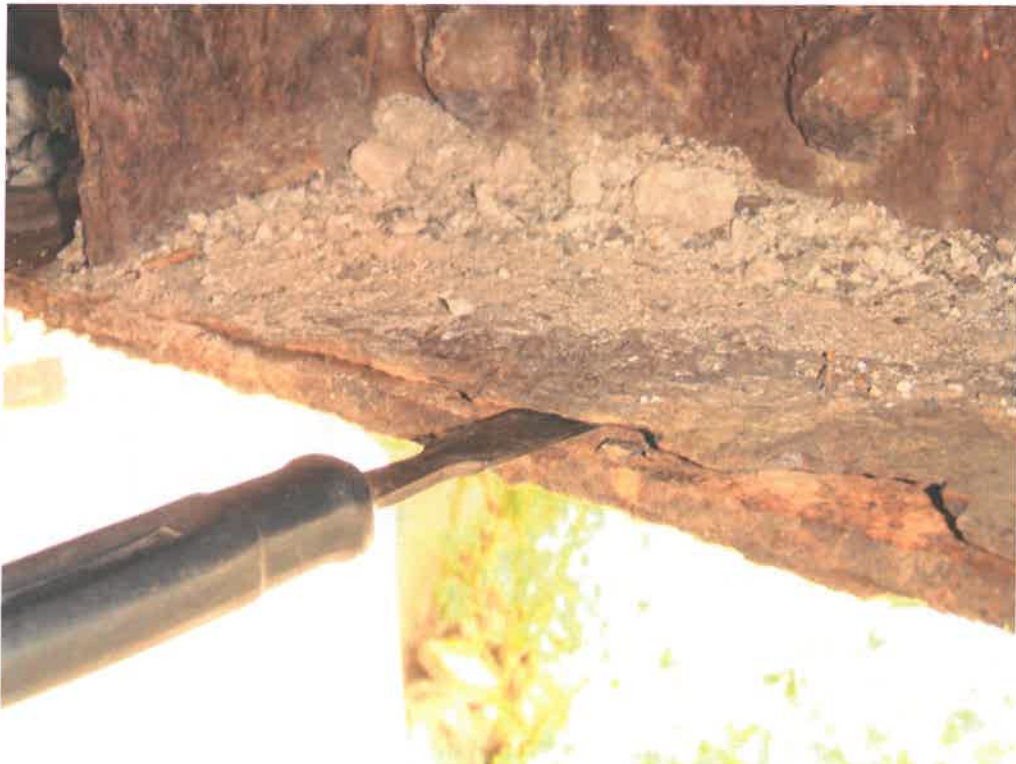
Photograph 6 – Corrosion and Metal Loss on Girder Bottom Flange in Span 6N
