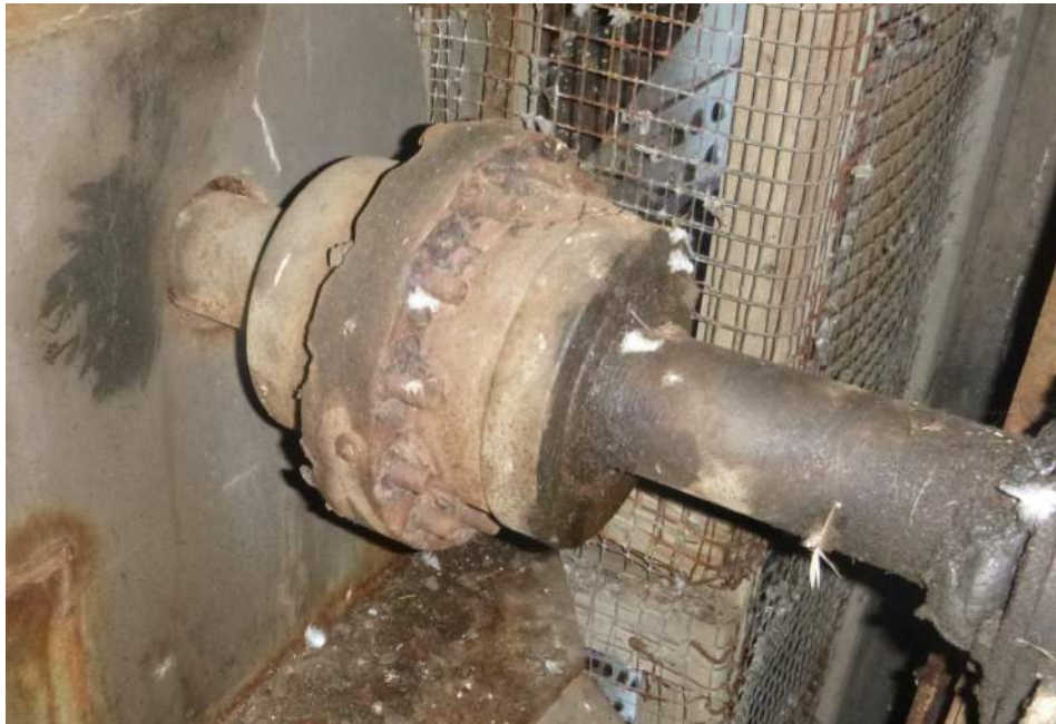
Photo M-08: The auxiliary machinery coupling exhibits corrosion and section loss around the fasteners on the connection flanges.
