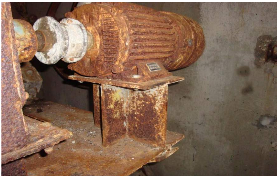
Photo E-09a, Emergency motor exhibited corrosion.
