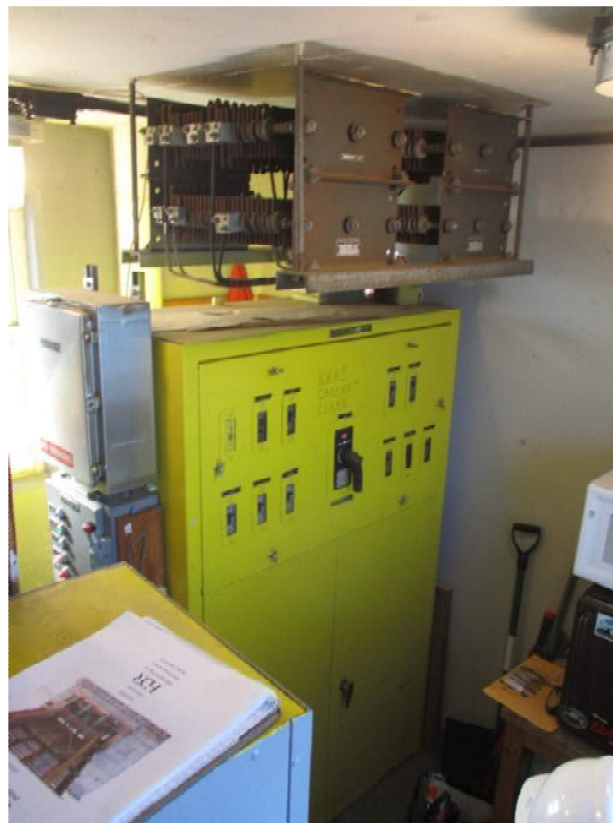
Photo E-12: Secondary Resistors (located above the MCC)
