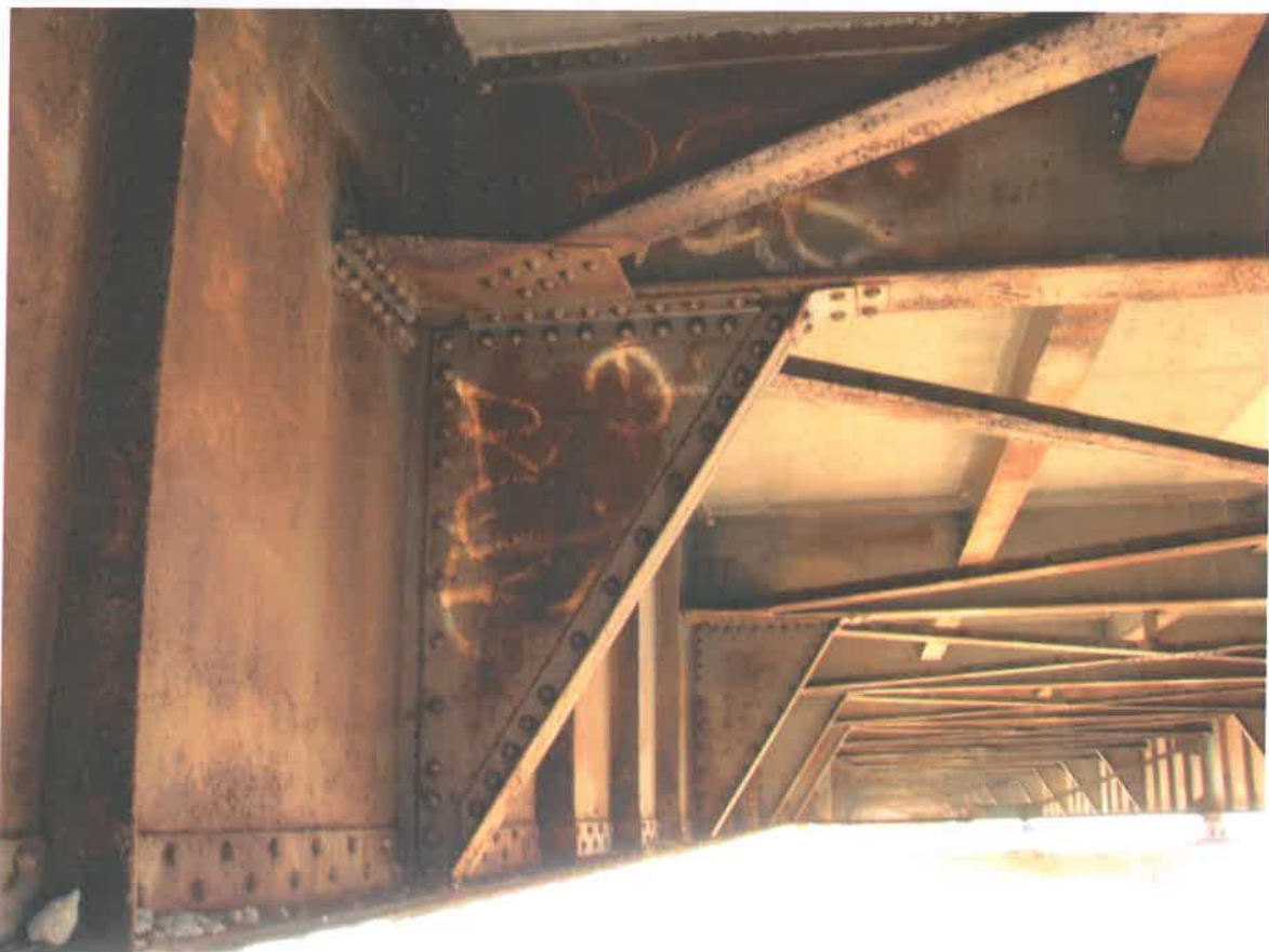
Photograph 4 – Typical Condition of Interior Face of Girder Webs Note Pinpoint Rust on Web and Stiffeners
