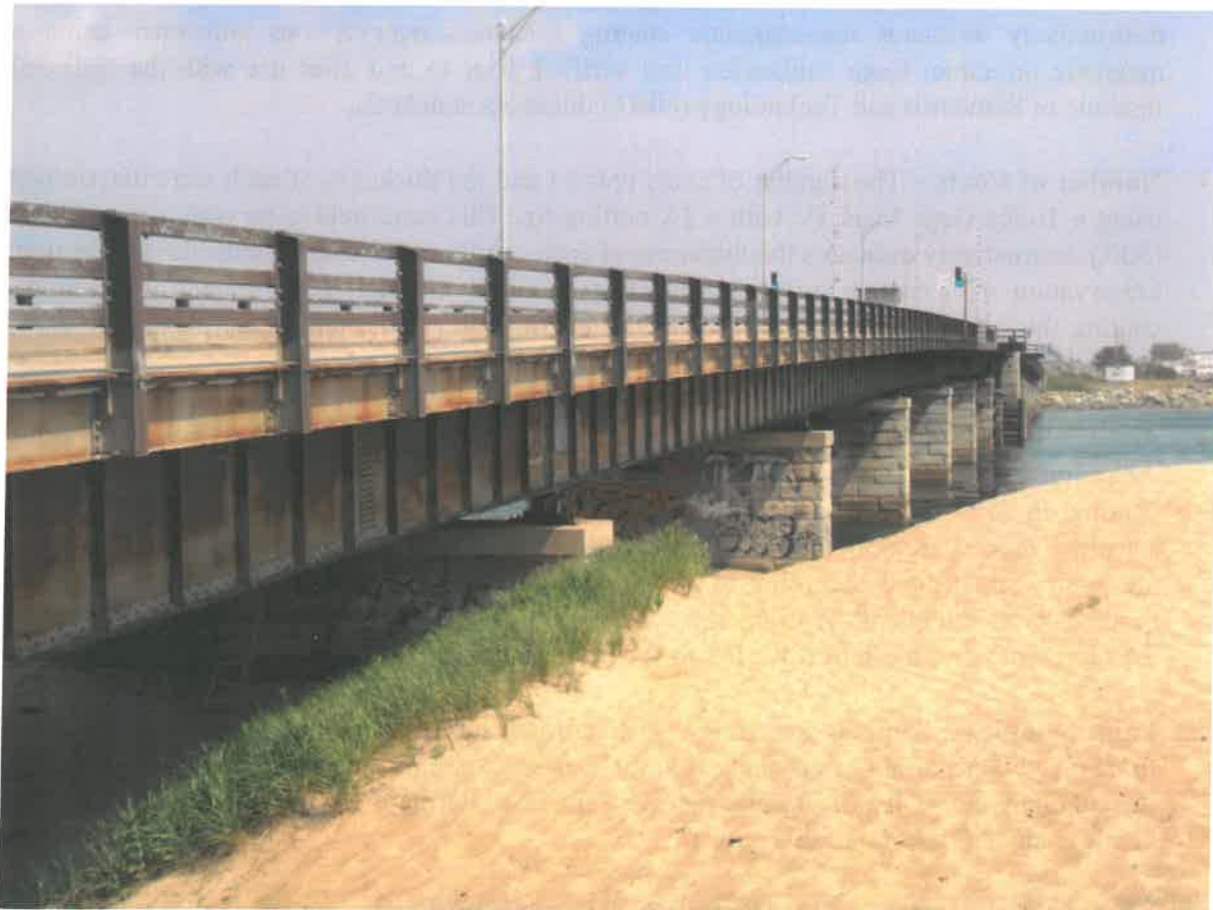
Photograph 3 -- View of Pinpoint Rust on Ocean Side Girder Webs and Sidewalk Stringers
