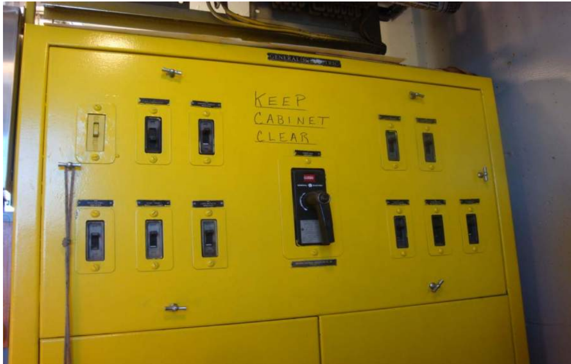
Photo E-01, Top-front portion of the MCC.
