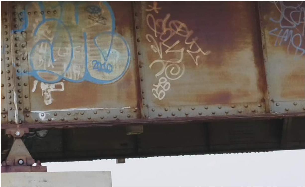
Photo S-09: Pack rust causing prying of cover plates over Pier 6S.
