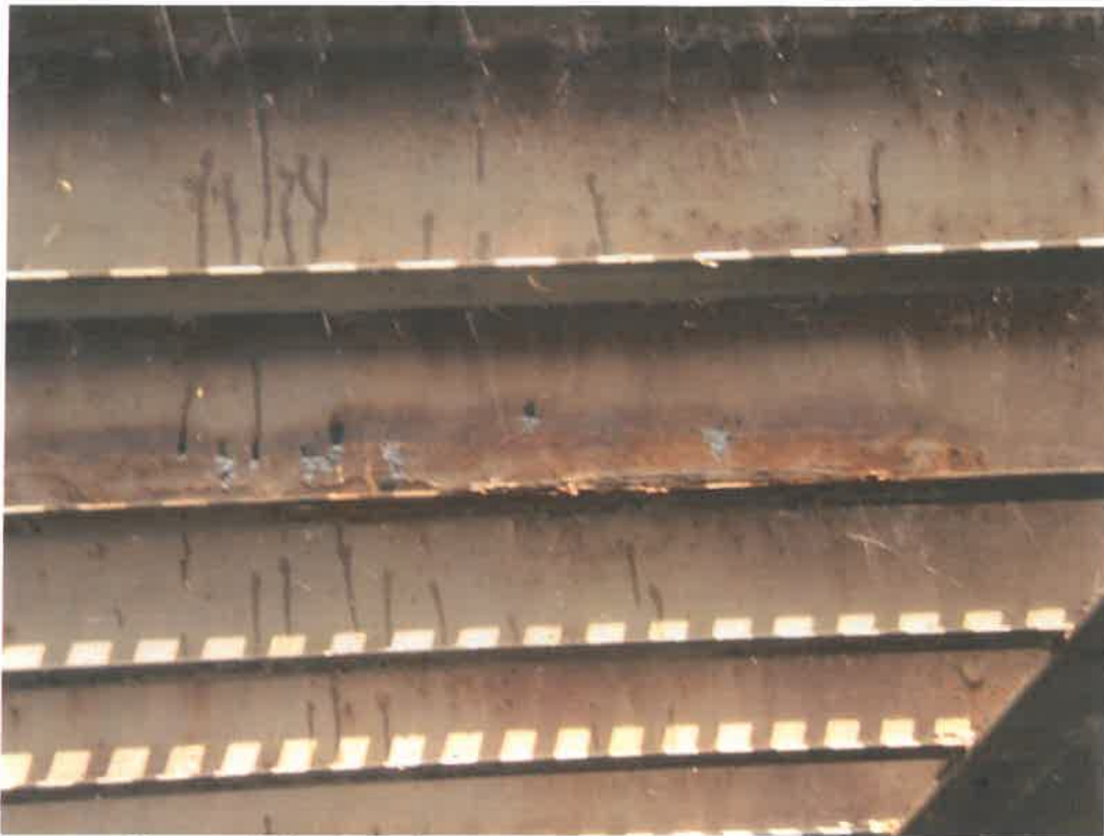
Photograph 20 – Corrosion on Flange of Channel Stringers in Lift Span
