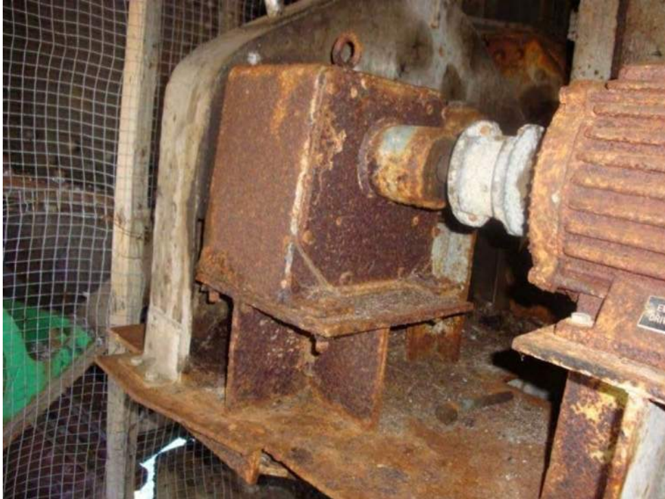
Photo M-11, Emergency drive primary reducer and machinery supports have paint loss and moderate corrosion.
