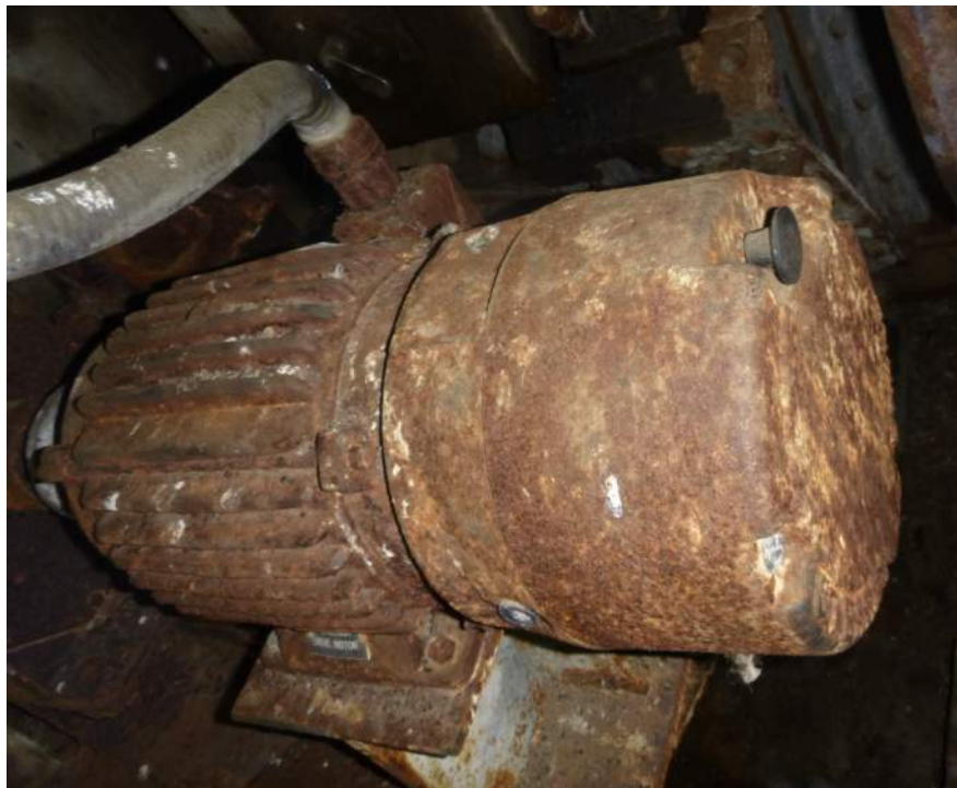
Photo M-06: The auxiliary motor and brake exhibit moderate to severe corrosion and have not been operated in several years.
