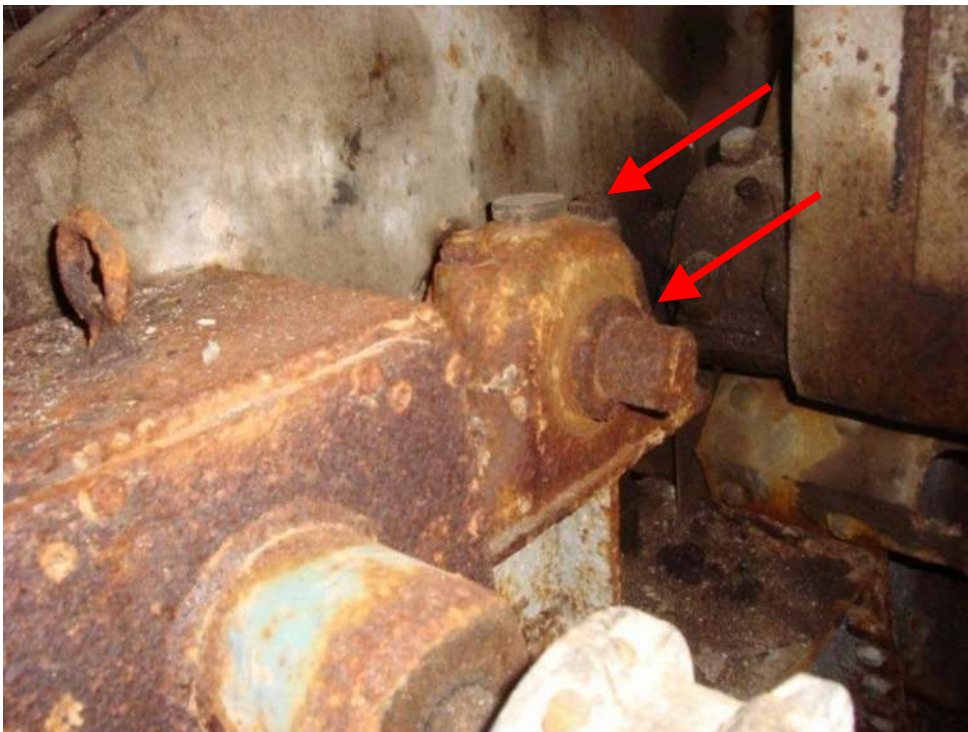
Photo M-14, The emergency drive open gear pillow block bearings and fasteners have complete paint loss and corrosion. Pillow block bearing lubrication appears dry.
