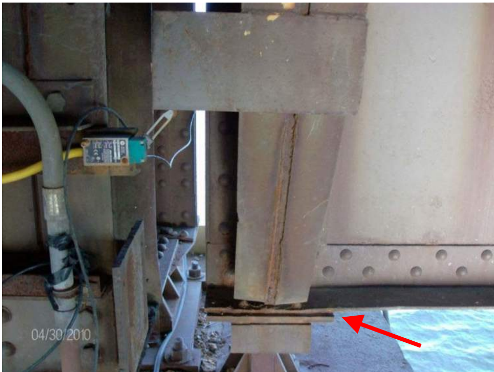
Photo M-22, The live load bearings were found to have some scattered areas of paint failure and corrosion, with no visible, significant wear. Please note the span seated limit switch which is being replaced as part of the electrical scope of work.
