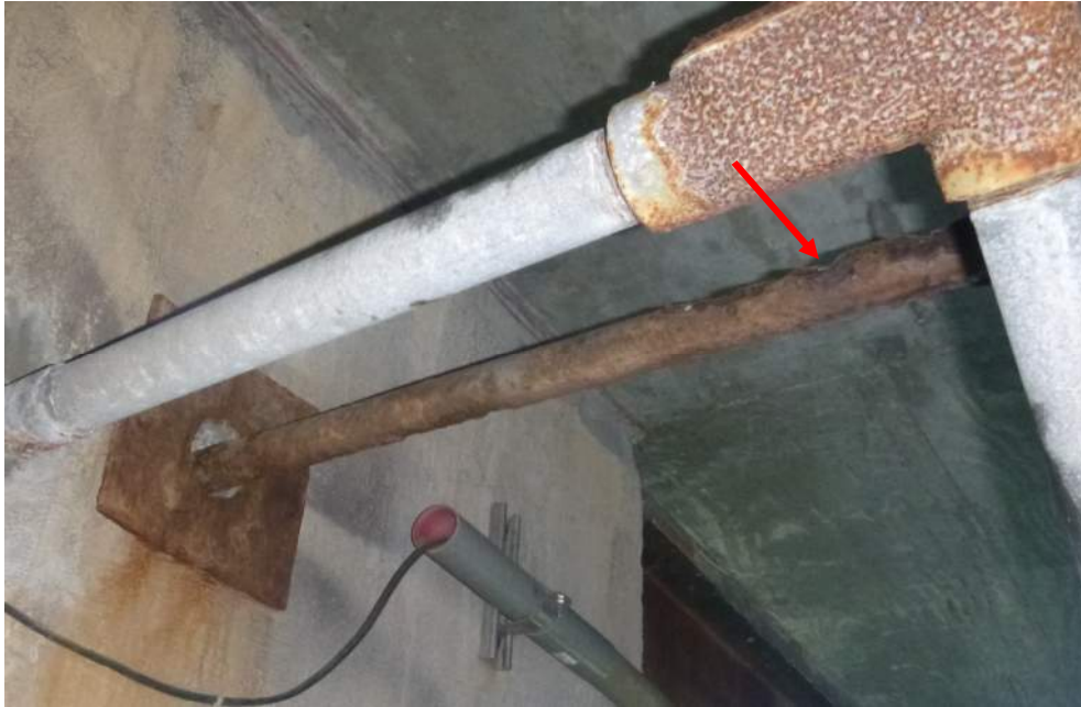
Photo M-15: The span drive instrumentation shaft is corroding and exhibits section loss.
