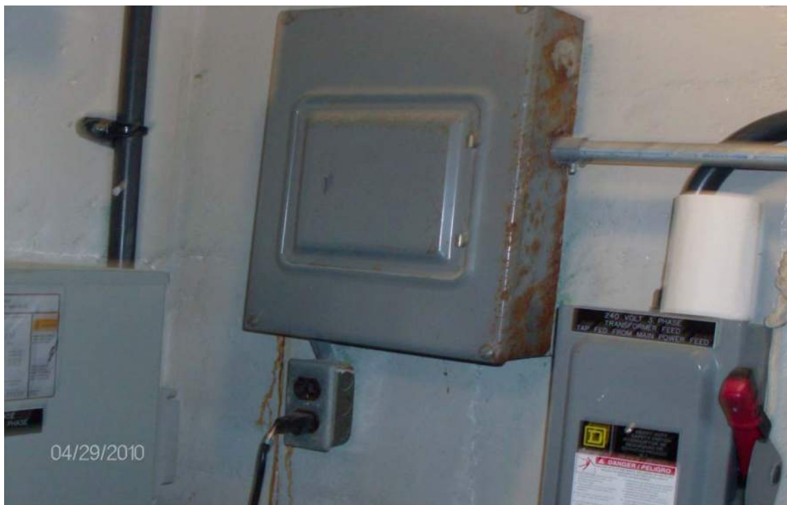
Photo E-22, 120/240 volts, lighting panel for air compressor and other EDG room receptacles.
