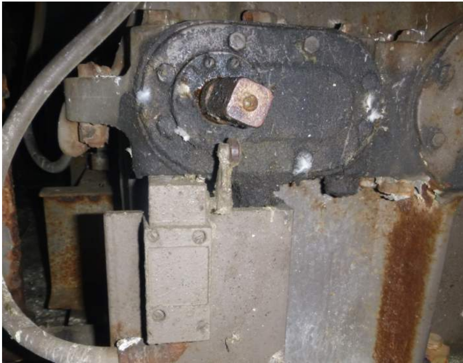
Photo M-11: The hand wheel shaft and limit switch are corroded and the limit switch lever arm has seized in place due to dirt and debris.
