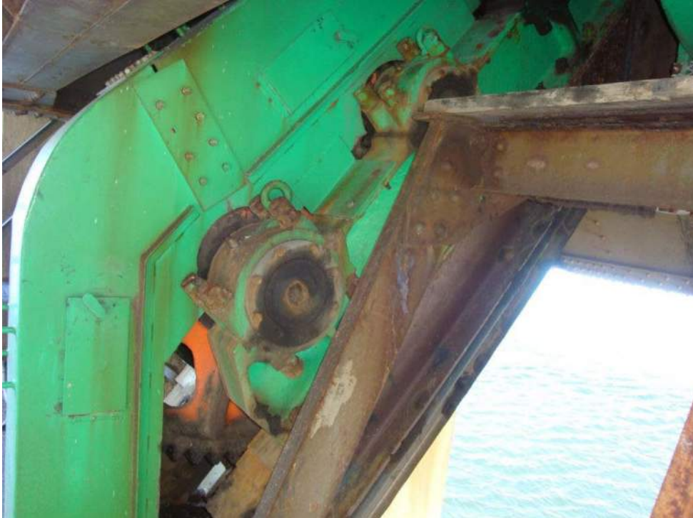
Photo M-07, The operating machinery bearings for the main drive appear in good condition. Some paint loss and corrosion is present and the lubrication appears dry.
