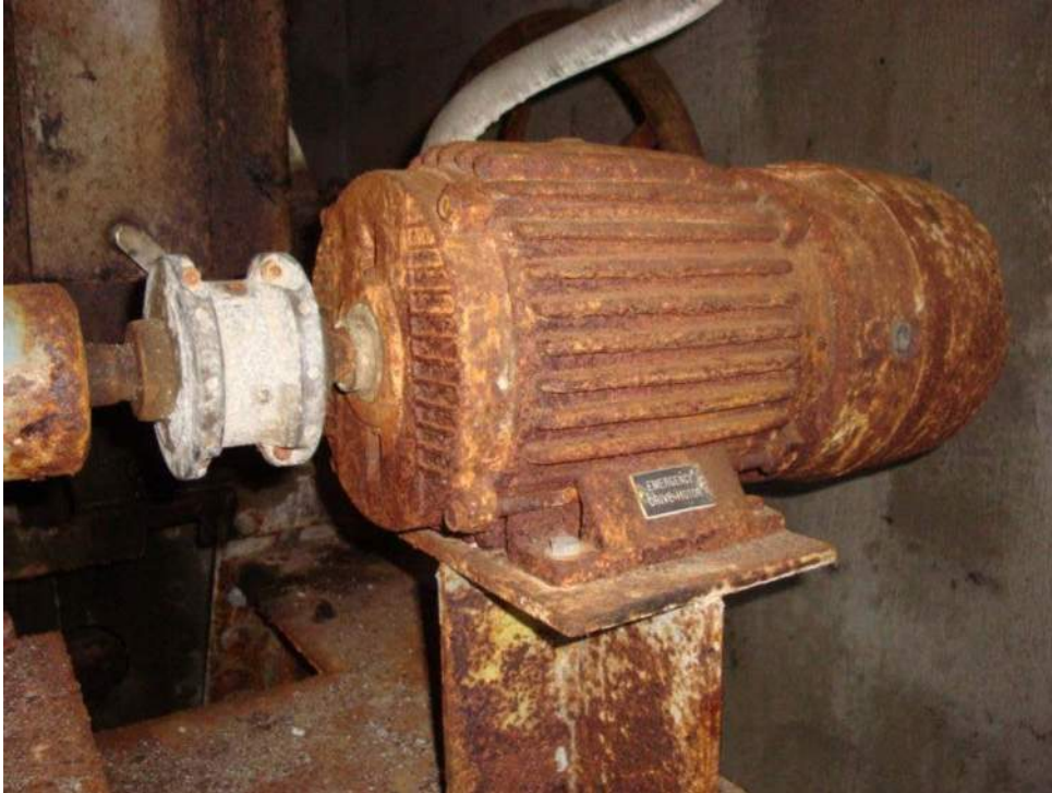
Photo M-09, The emergency drive motor, motor brake and pedestal have substantial paint loss and corrosion.
