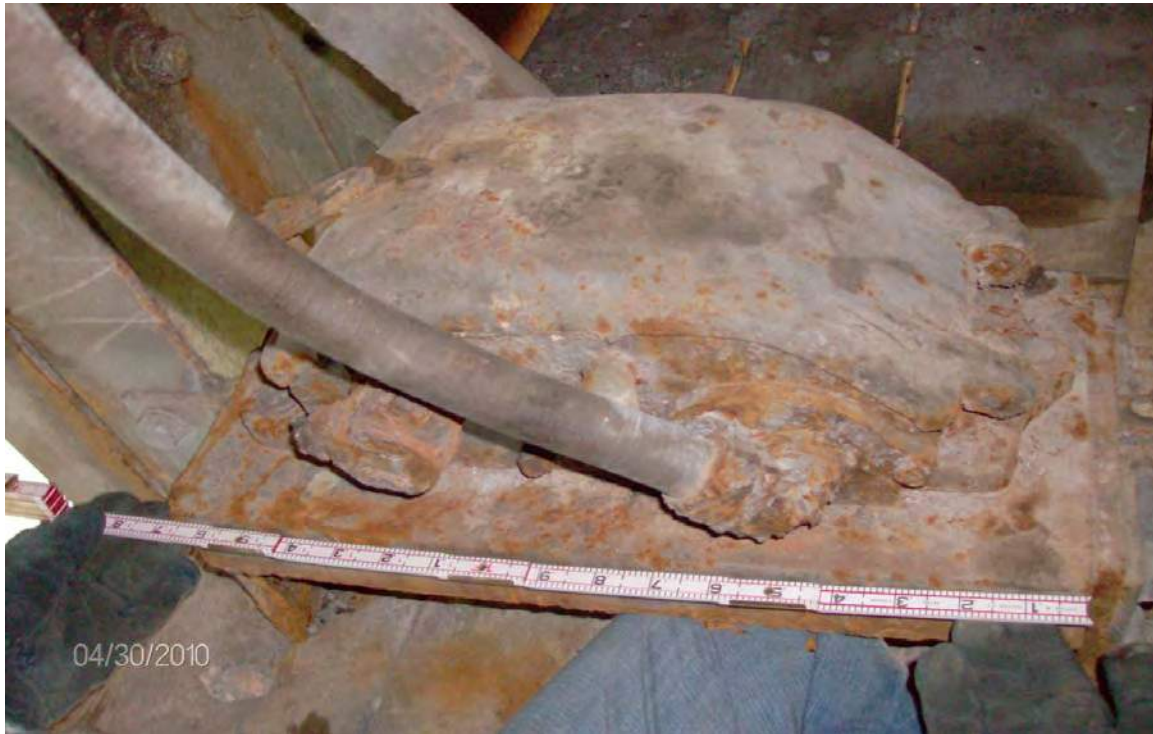
Photo E-16, Span lock position switch signs of corrosion.
