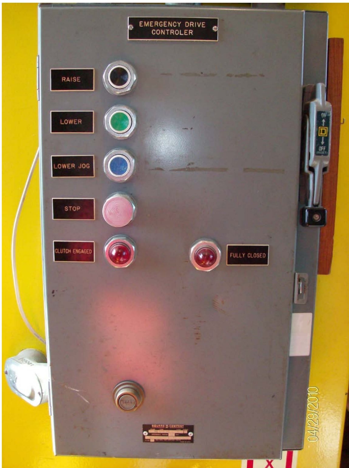
Photo E-09b, Emergency drive controller.
