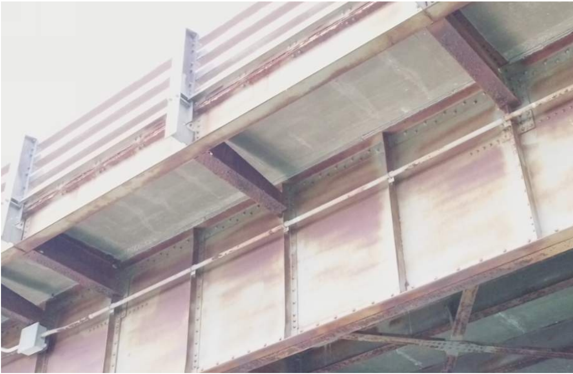
Photo S-01: Typical approach span deck overhang condition.
