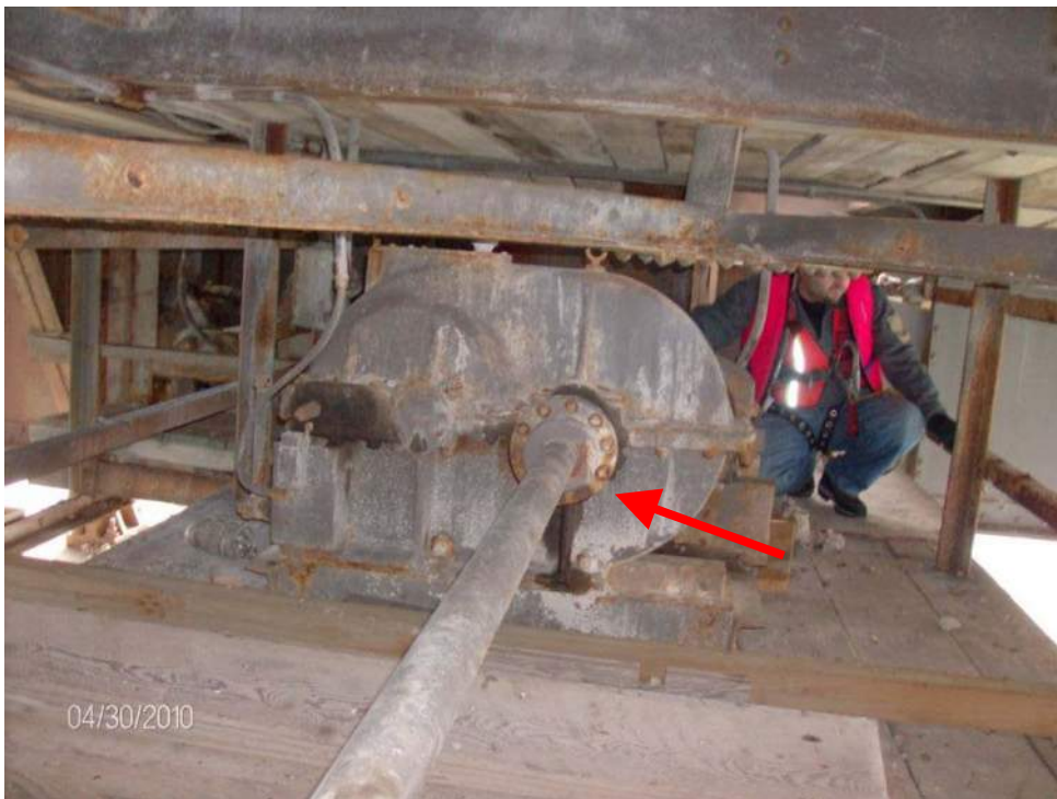
Photo M-20, The span lock shafts and couplings have scattered areas of paint loss and corrosion. The coupling lubrication appears dry.
