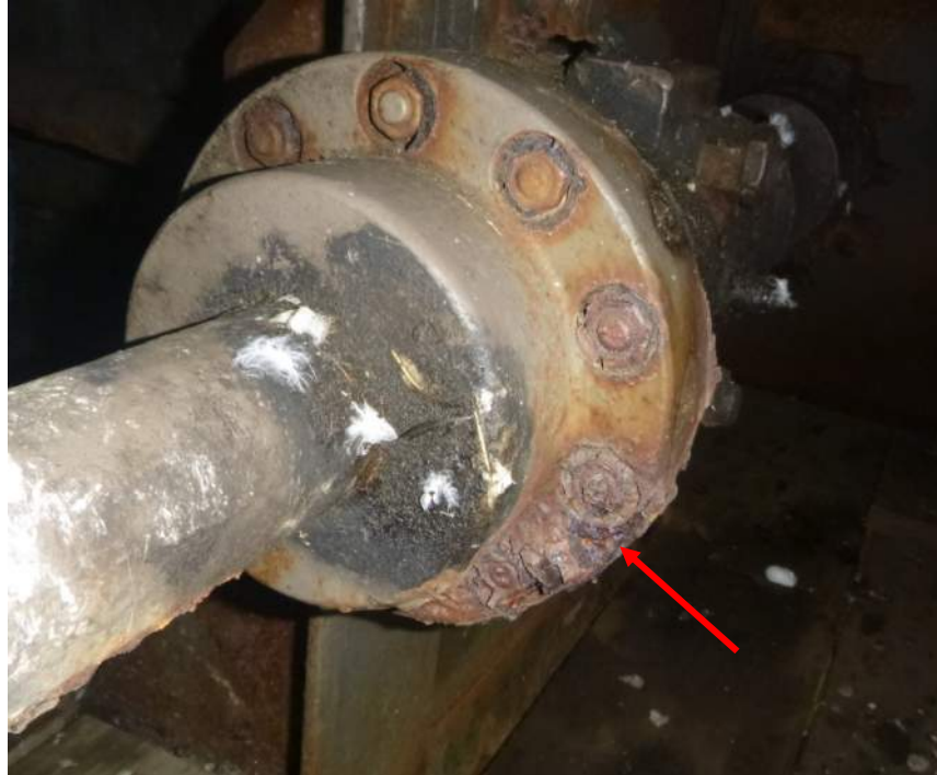
Photo M-12: The span lock machinery couplings exhibit corrosion and section loss on the flanges around the fasteners.
