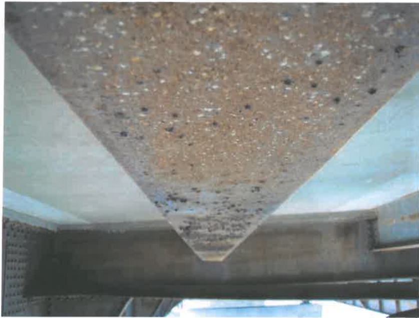
Photograph 11 – Typical Coating Deterioration and Corrosion on Stringer Bottom Flanges
