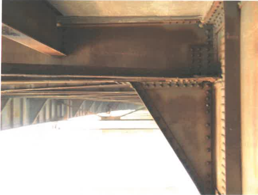
Photograph 7 – Typical Pinpoint Rust on Floorbeams and Floorbeam Haunch
