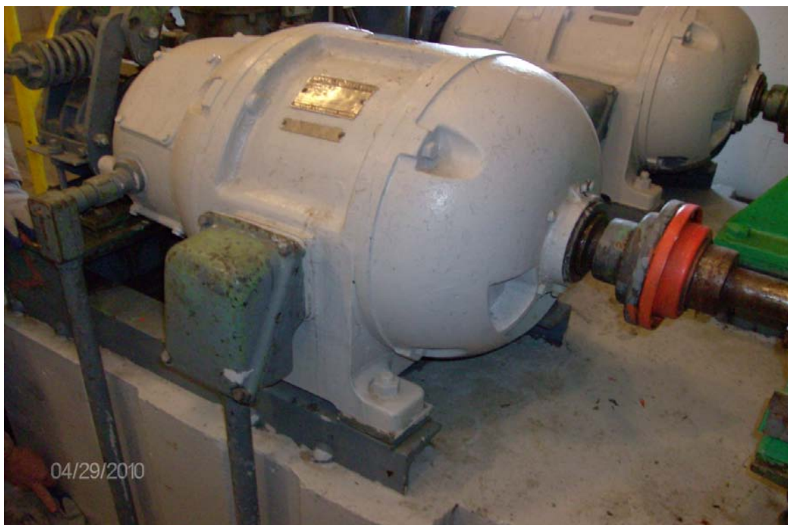
Photo E-05, Main motors.
