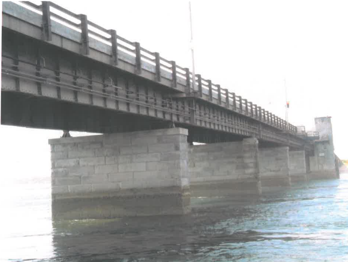
Photograph 1 – View of Harbor Side Fascia and Bridge Rail
