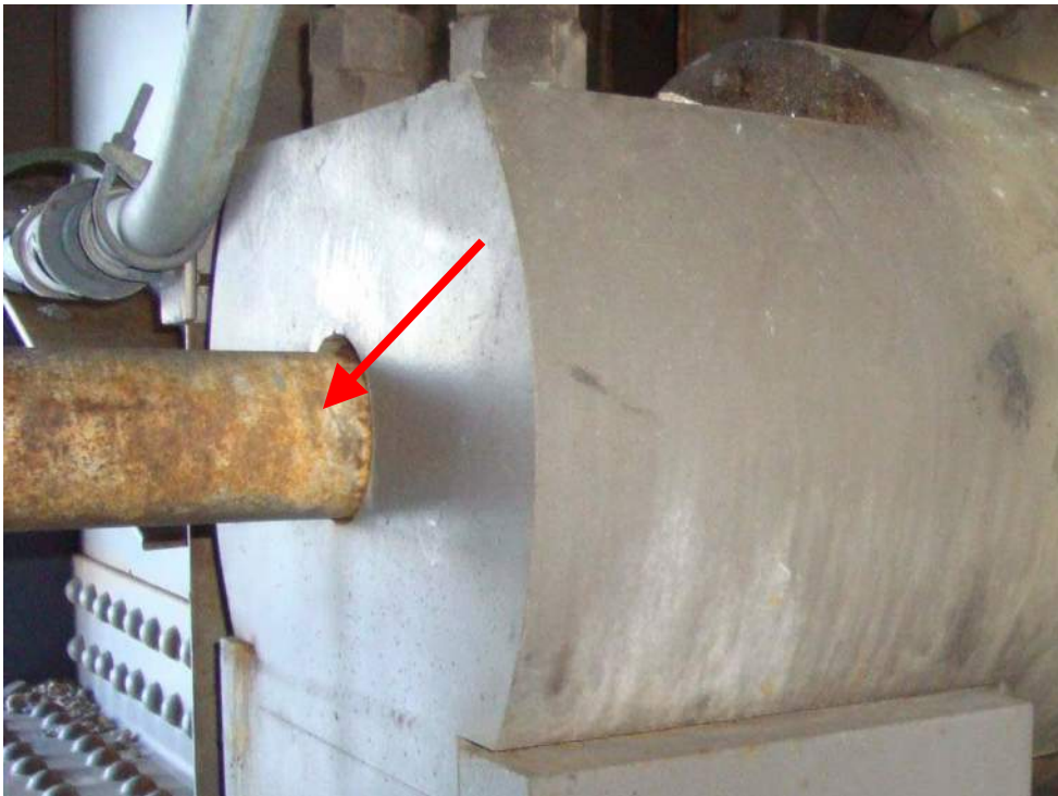
Photo M-06, The operating machinery shafts have scattered areas of paint loss and corrosion.
