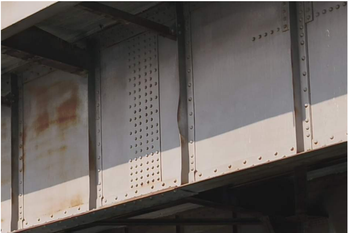
Photo S-08: Bent stiffener plate in Span 1N on the outboard side of the east girder, north of the northern girder splice.
