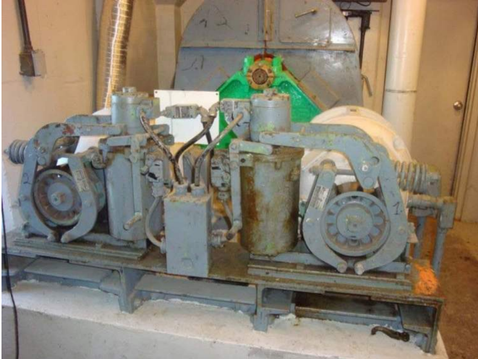
Photo M-01, General Electric 8 inch thruster brakes mounted on auxiliary side of 15 HP main span drive induction motors. View of motor room looking east.
