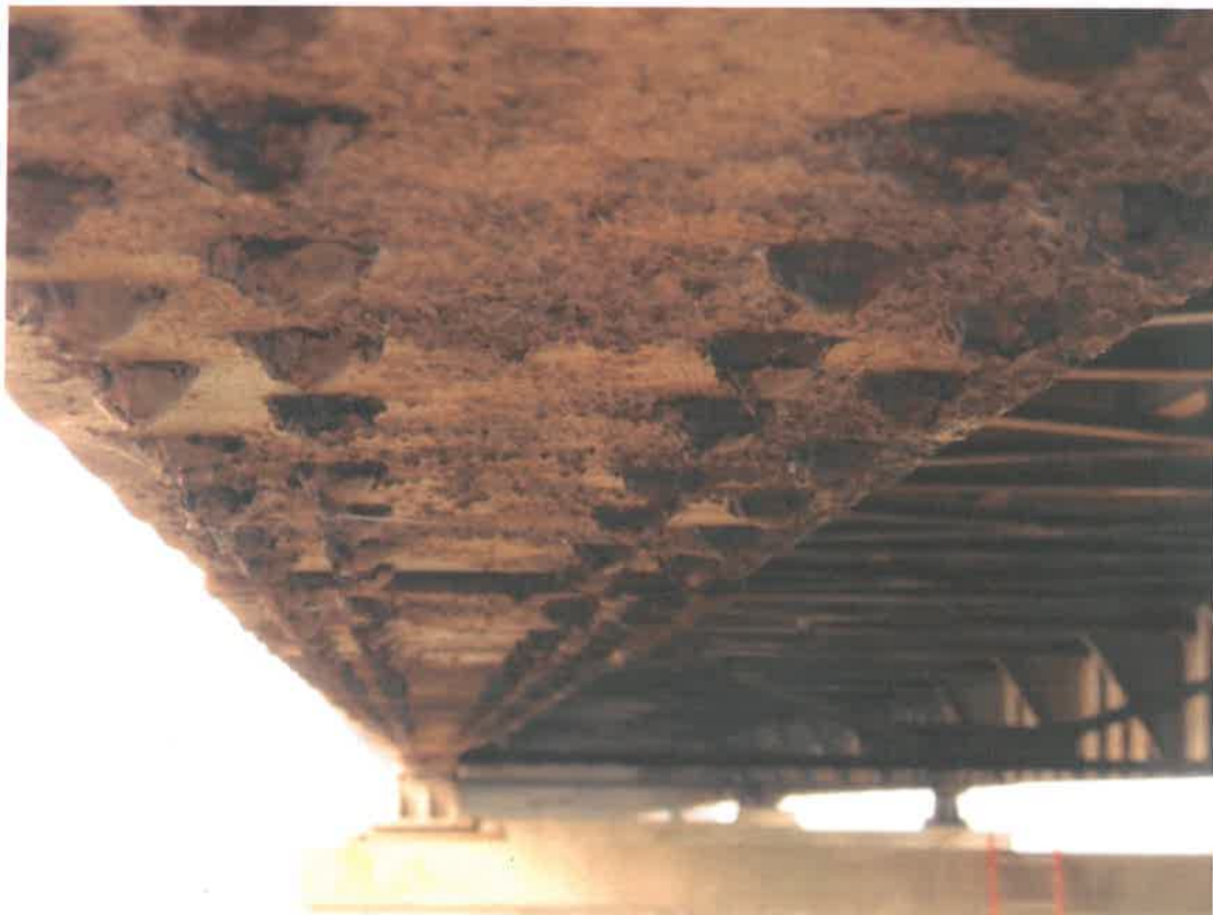
Photograph 2 – Typical Coating Deterioration and Corrosion on Girder Bottom Flanges in Span 6N
