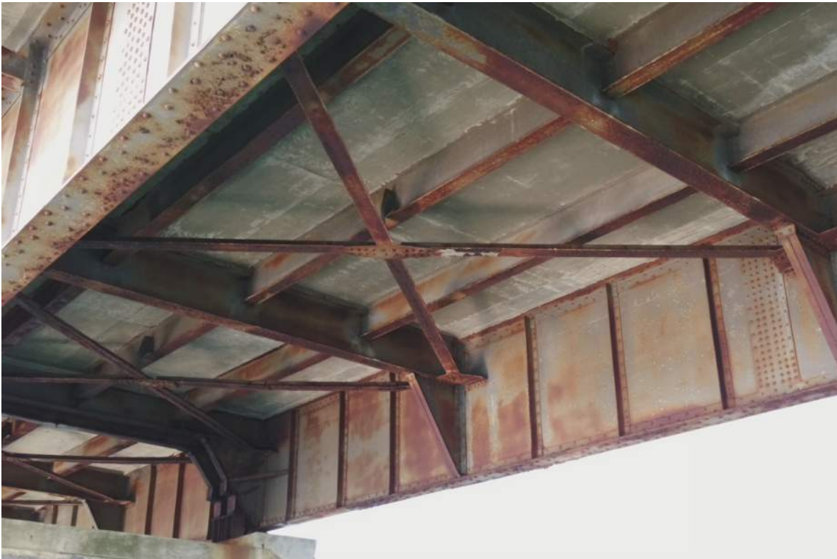
Photo S-02: Typical approach span deck condition.
