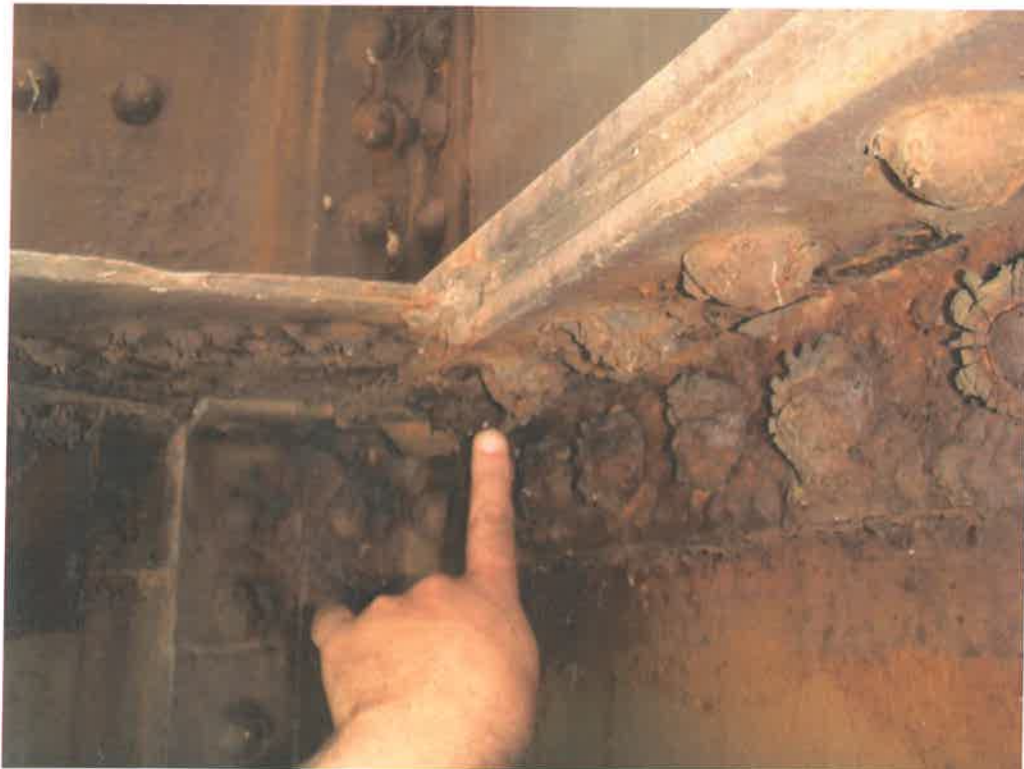
Photograph 23 – Heavy Corrosion Rivets in Lift Span
