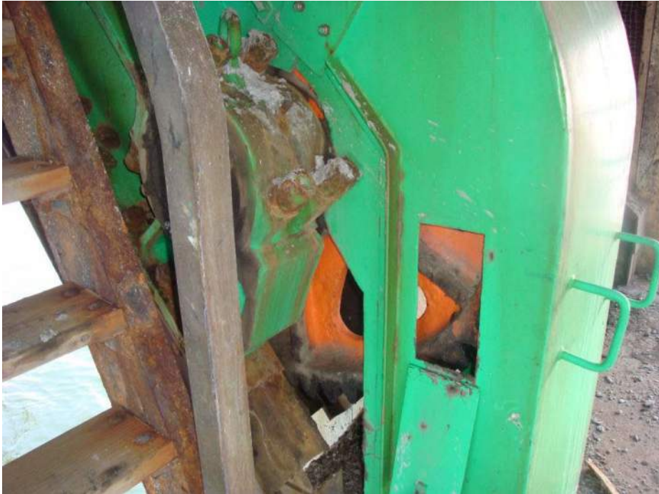
Photo M-05, The centrally located differential and secondary open gearing were concealed by a heavy steel cover. Inspection windows provide a limited view of the gear teeth. The lubrication appears dry and contaminated.
