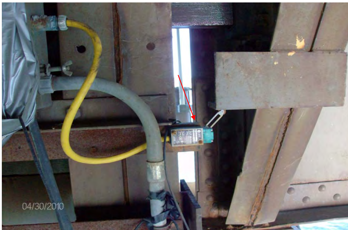
Photo E-13, Span seated lever arm limit switch (only one is used for seating indication).
