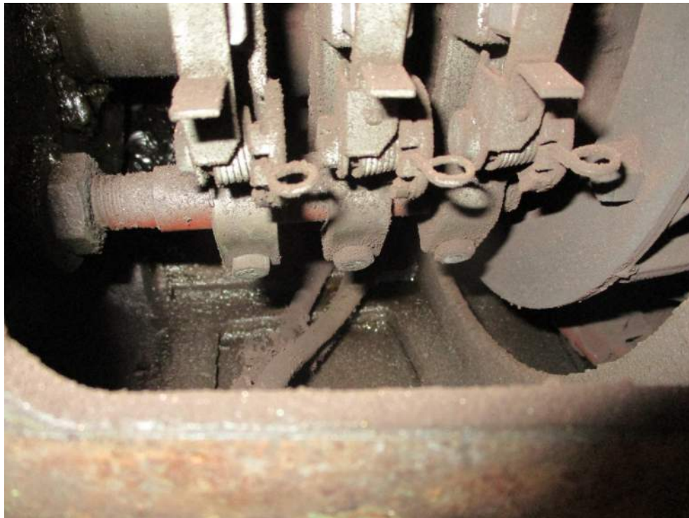
Photo E-06: Inside View of Main Span Motor 2 Showing Dirt/Dust Build Up
