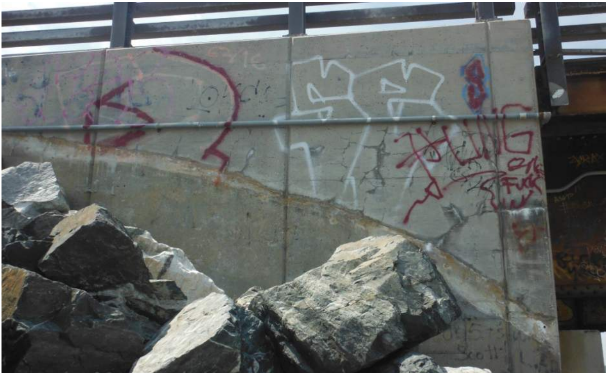
Photo S-20: Cracks and efflorescence at southeast wingwall.
