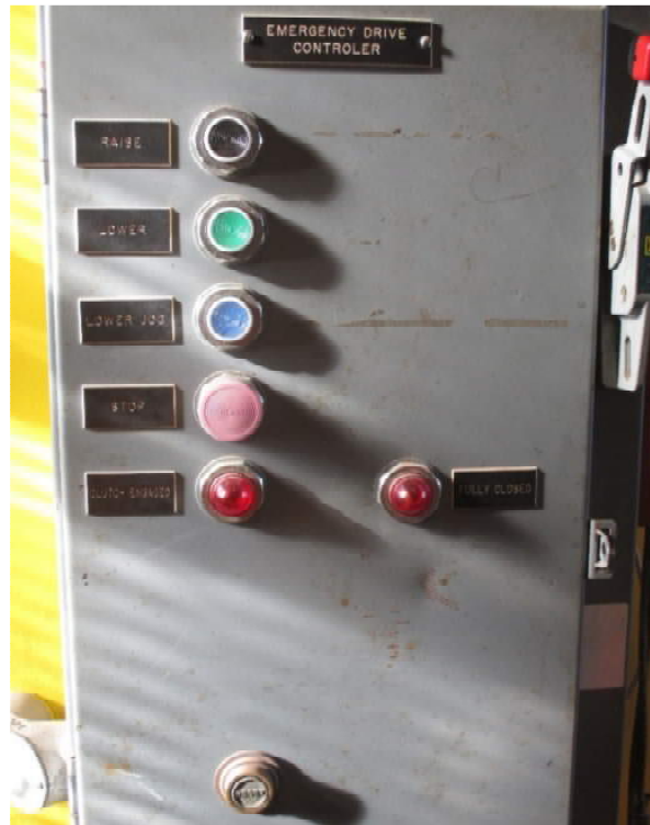
Photo E-08: Emergency Motor Control Panel
