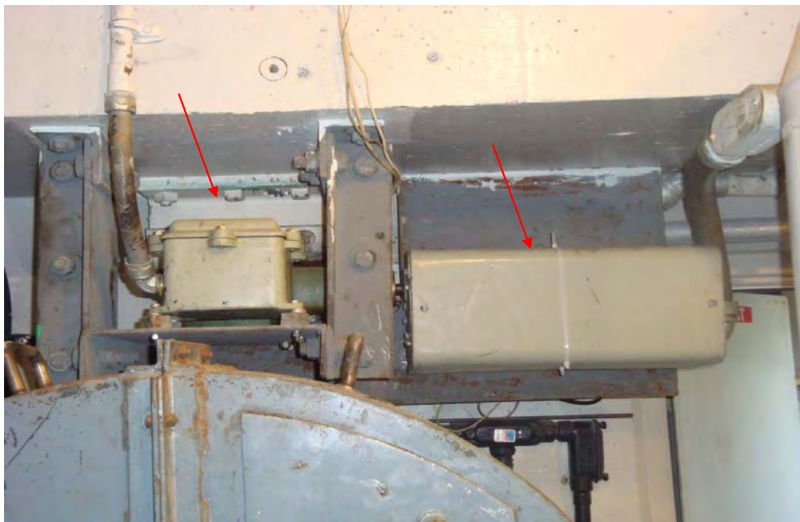
Photo E-12, Location of rotary cam limit switch & height transmitter.
