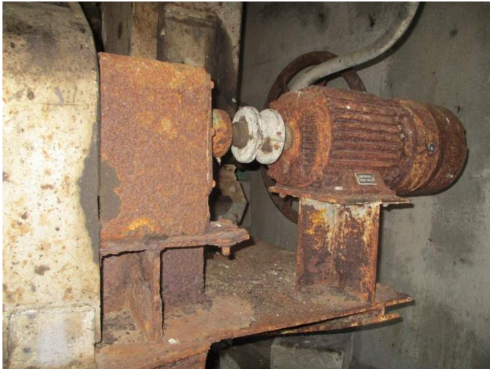
Photo E-07: Emergency Motor Exhibiting Corrosion & Rust
