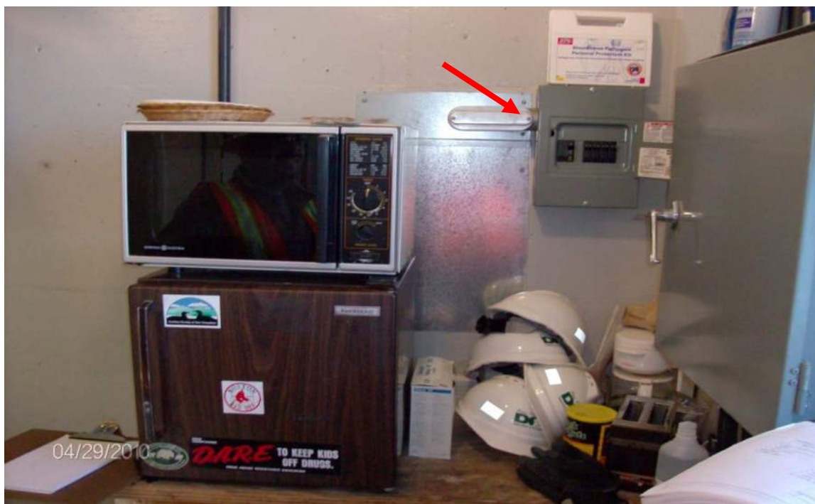
Photo E-19, 120/240 volts, 100 amp lighting panel.
