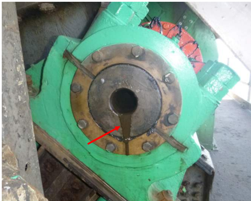
Photo M-04: The main pinion shaft coupling grease is leaking through the connecting shafts.
