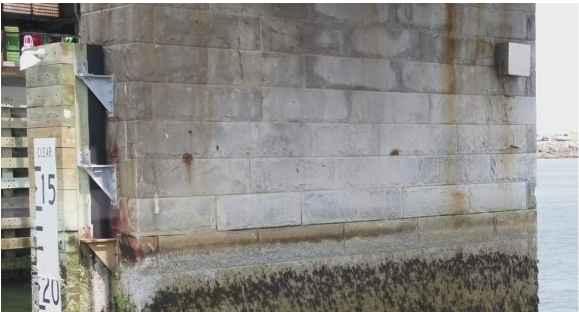
Photo S-22: Typical pier condition with cracked granite stones and deteriorated mortar at the water line.
