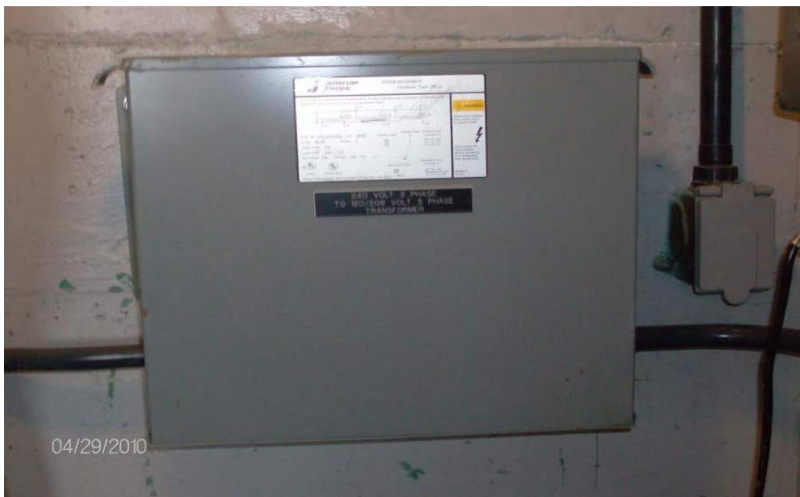
Photo E-21, 120/240-120/208 volts, step down transformer for barrier gates lighting panel.
