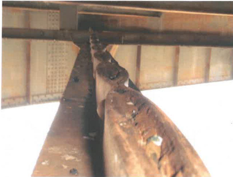
Photograph 13 -- Significant Pack Rust between Lateral Bracing Back-to-Back Angles
