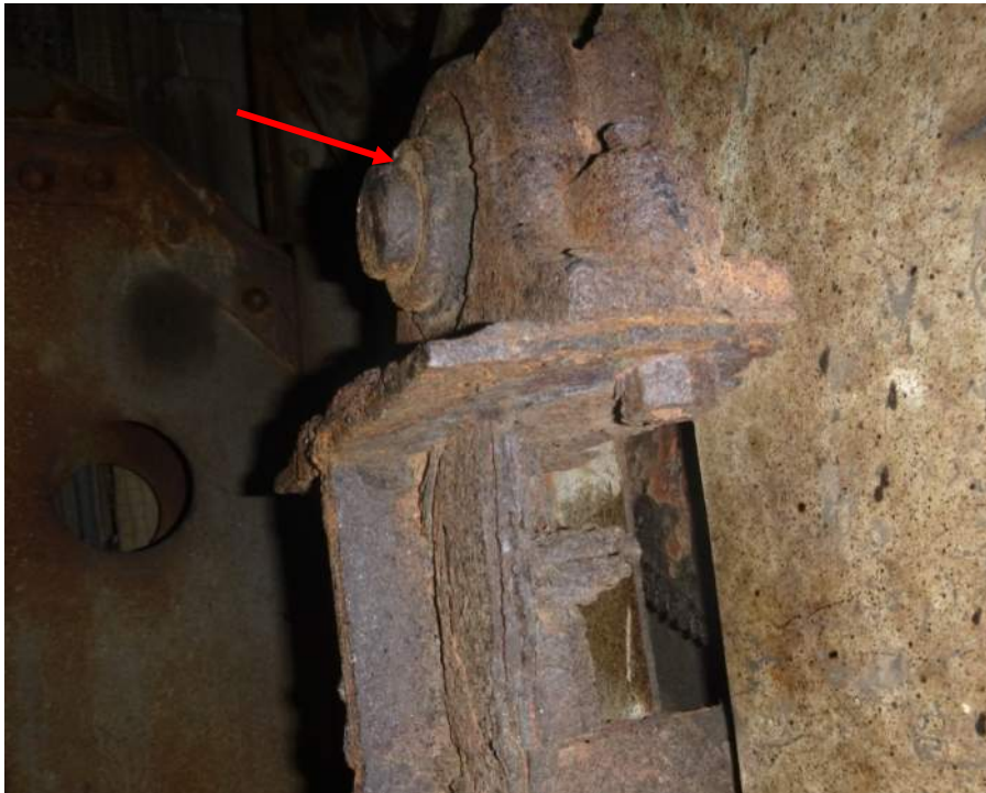
Photo M-09: The bearings and mounts for the primary open gear set of the auxiliary machinery are severely corroded and may have seized with the shaft.
