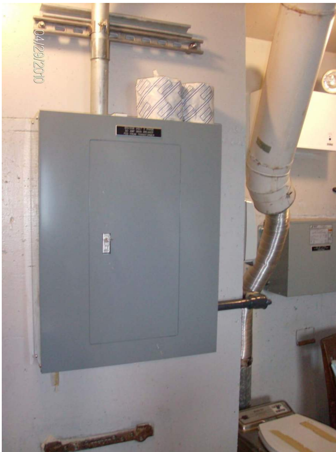
Photo E-20, 120/208 volts, 50 amp barrier gates lighting panel.
