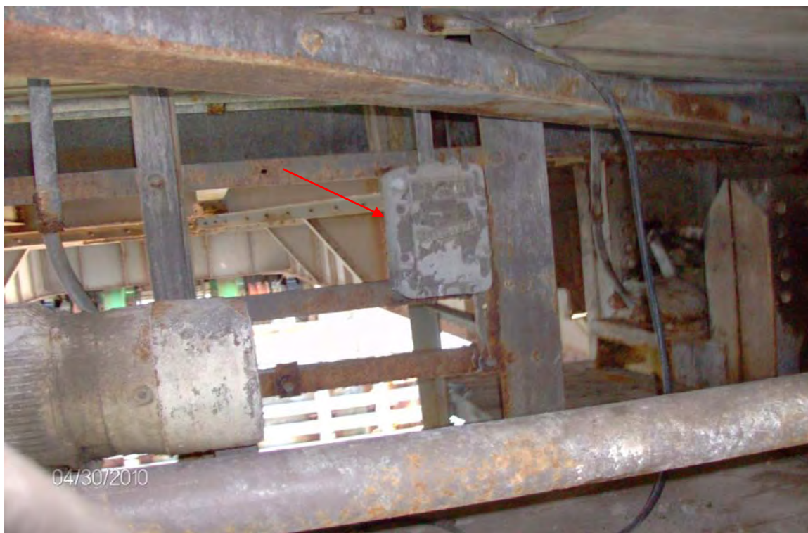
Photo E-15, Span lock motor local disconnect switch.
