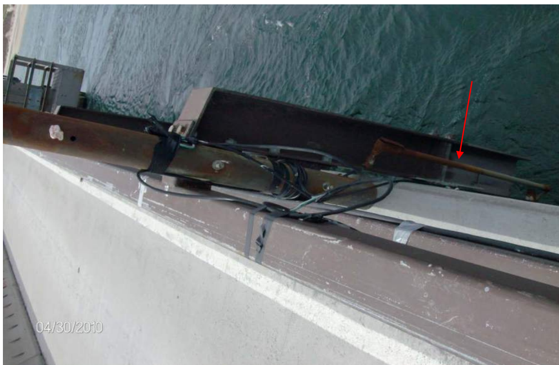
Photo E-25, Showing the old conduit system at the north approach traffic lights.
