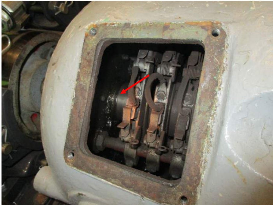
Photo E-05: Inside View of Main Span Motor 1 Showing Grease Build Up
