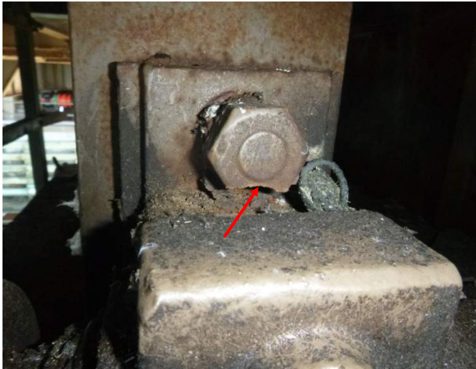
Photo M-13: The fasteners on the crank arm bearings are severely corroded with over 50% section loss.
