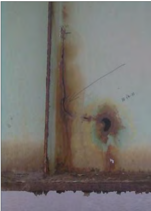
Figure BR8: Hole and Crack in Web at Transverse Stiffener
