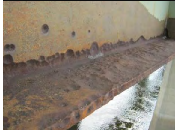
Figure BR7: Bottom Flange Pitting
