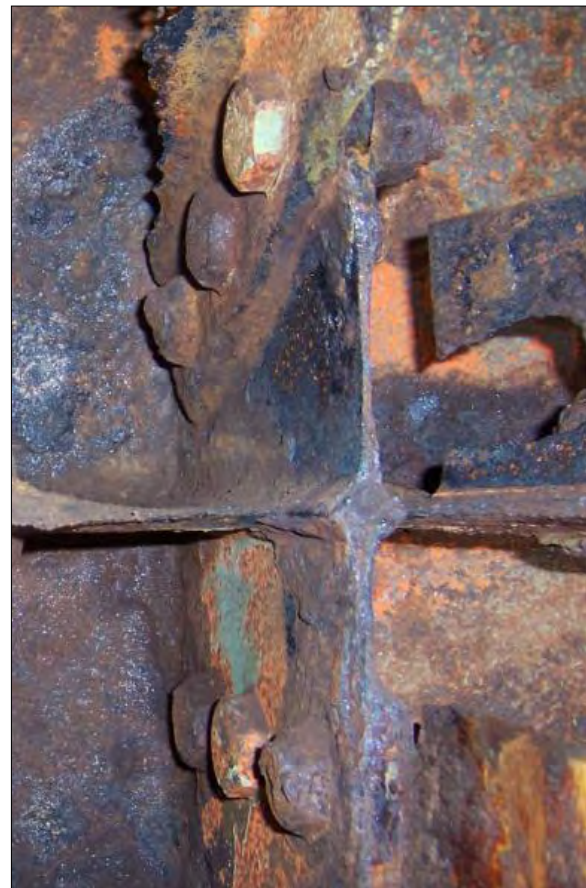
Figure BR6: Knife-Edge. Heavy Section Loss at Stiffener & Gusset Plate
