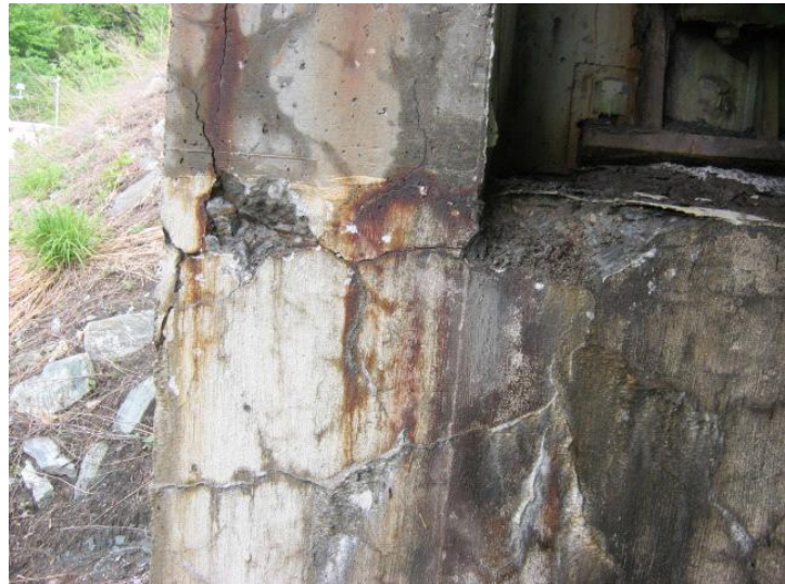
Bridge abutment showing cracks and spalls
