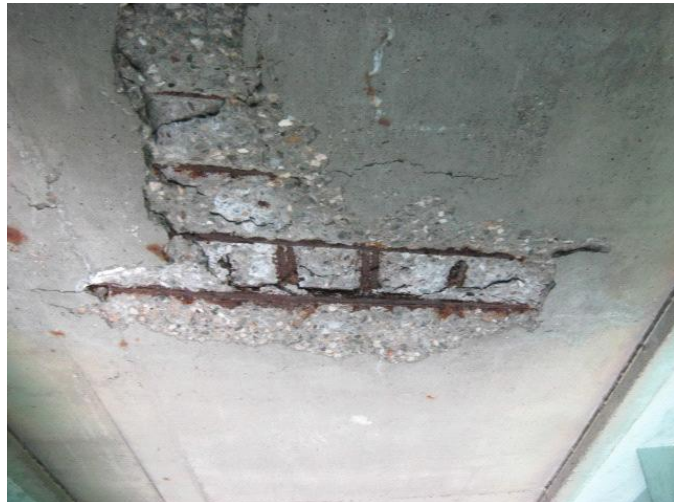
Large spall in the bridge span
