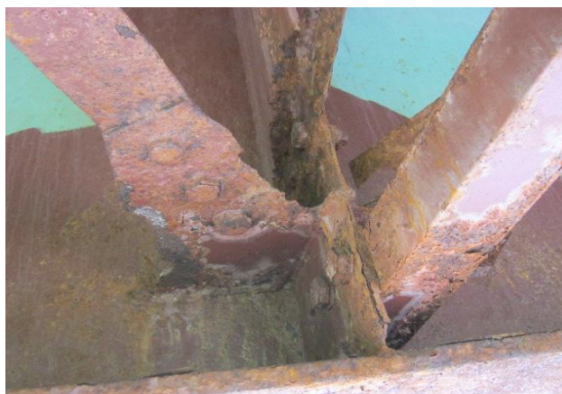
Rust and scale under relief joint
