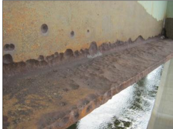
Figure BR7: Bottom Flange Pitting
