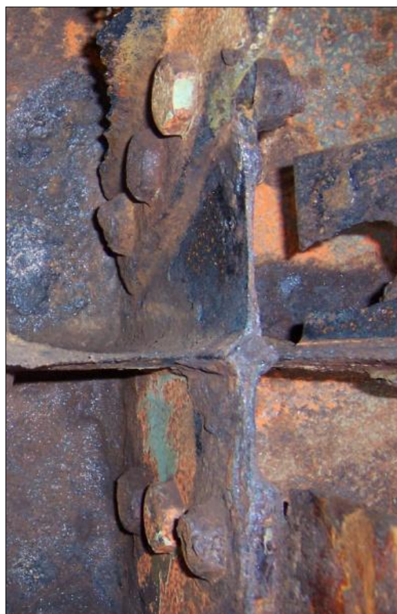
Figure BR6: Knife-Edge. Heavy Section Loss at Stiffener & Gusset Plate
