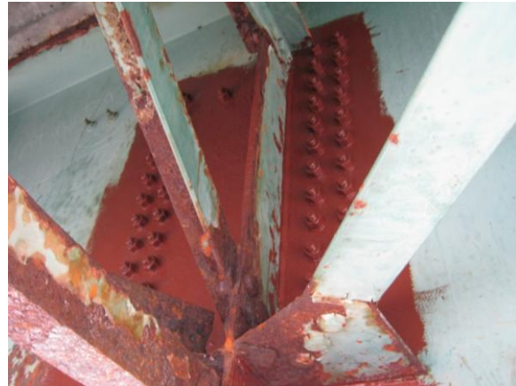
Figure BR10: Web Crack Bolted Plate Repair by NHDOT BBM (inside face)
