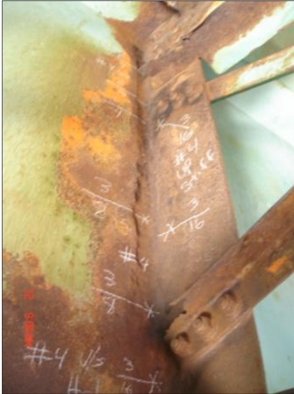
Figure BR12: Heavy Pitting on Web at Transverse Stiffener
