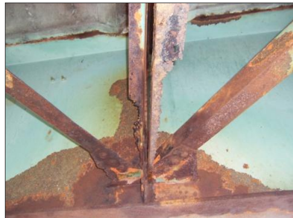
Figure BR11: Heavy Section Loss Under Deck Relief Joint
