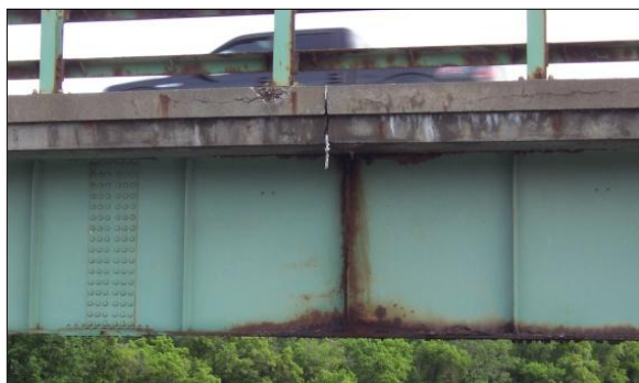
Figure BR5: Typical Corrosion at Deck Expansion Joint
