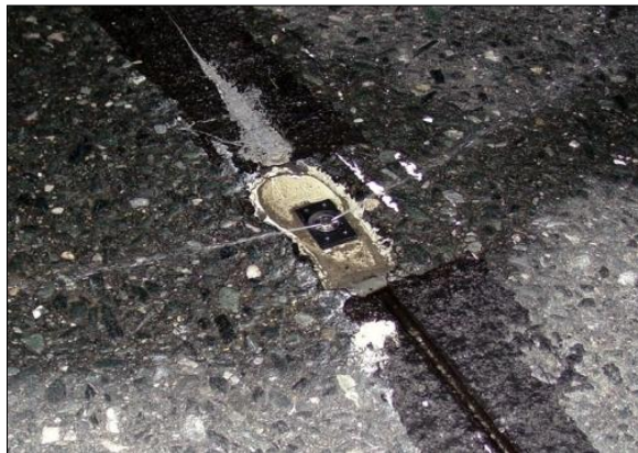
Figure BR2: FAST Anti-Icing System Nozzle Installed in SB Bridge Pavement
