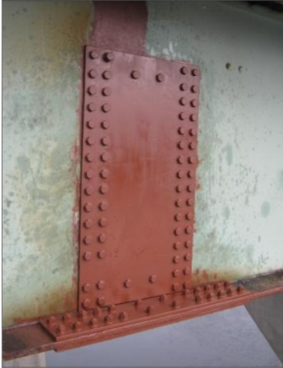
Figure BR9: Web Crack Bolted Plate Repair by NHDOT BBM (outside face)
