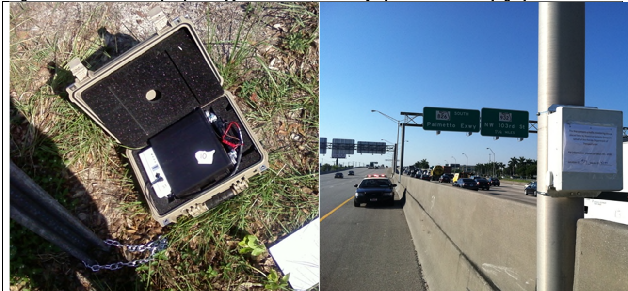
Figure 1: BlueFax Device (left) and Typical Post-Mounted Deployment on SR-826 (right)
