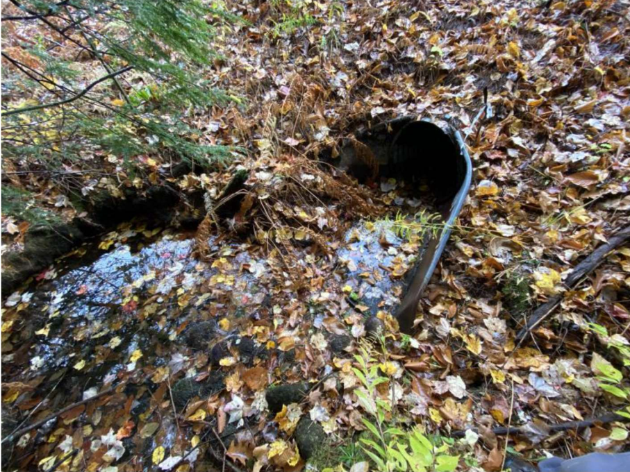
Impact Locations G and H: Looking towards the inlet of the 24" CMP at approx. Sta. 1336 SB in Wetland #s 20 and 26.
