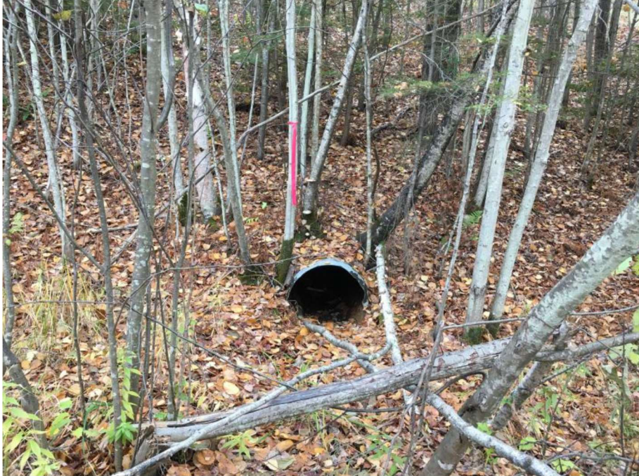
Impact Location X: Looking towards the outlet of the 24" CMP at approx. Sta. 1470 SB Median in Wetland # 155.
