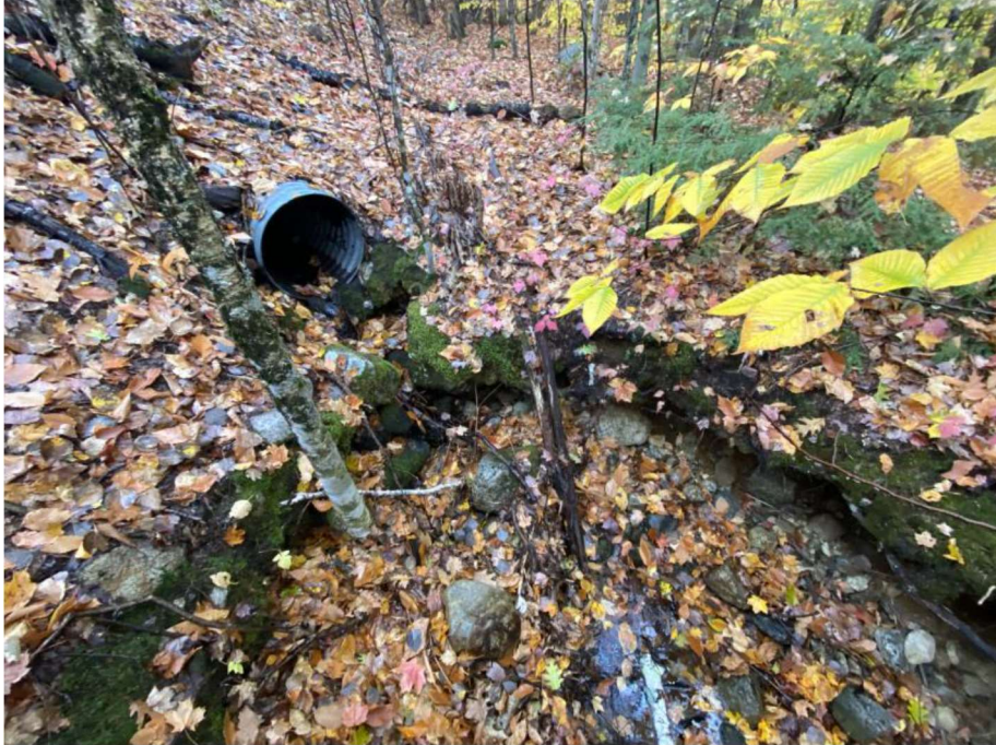
Impact Locations D, E and F: Looking towards the outlet of the 24" CMP at approx. Sta. 1336 SB Median in Wetland #s 27, 26 and 28.
