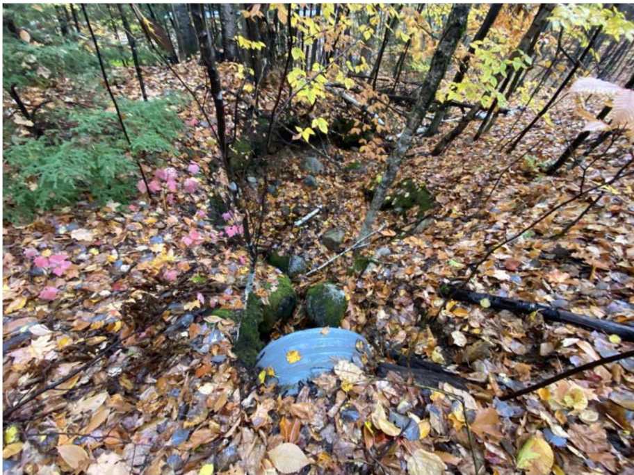
Impact Locations D, E and F: Looking away from the outlet of the 24" CMP at approx. Sta. 1336 SB Median in Wetland #s 27, 26 and 28.
