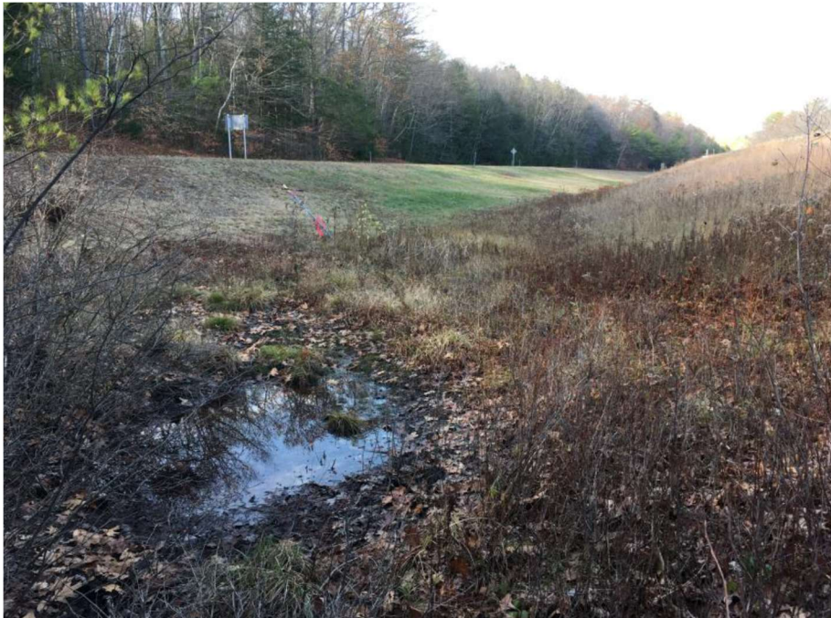
Impact Location W: Looking away from the inlet of the 24" CMP at approx. Sta. 1465 SB in the median between the mainline and Exit 10 SB Off-Ramp in Wetland # 149.
