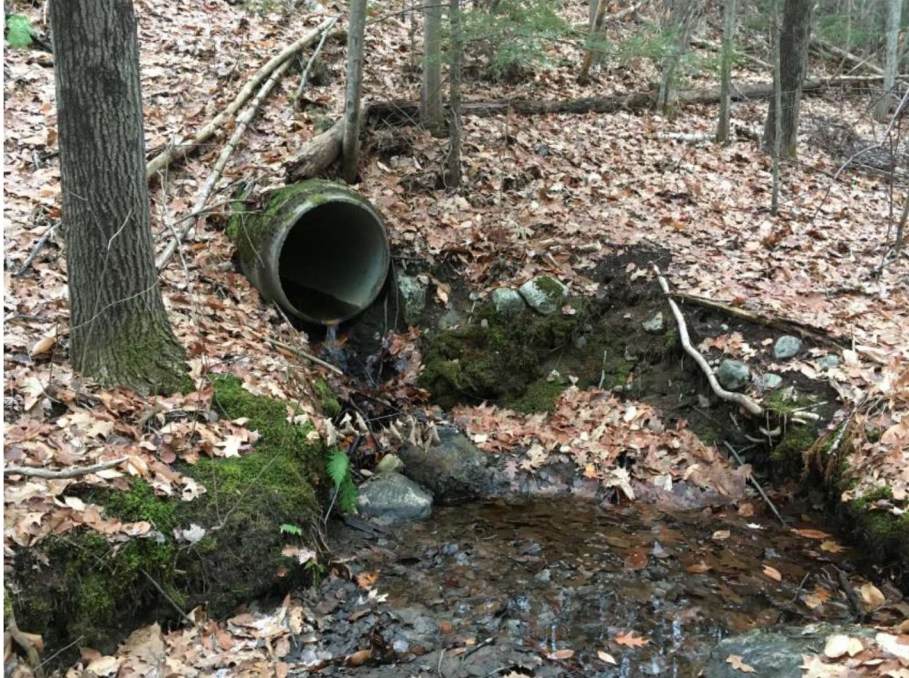
Impact Location J: Looking towards the outlet of the 30" RCP at approx. Sta. 1437 NB in Wetland # 117.
