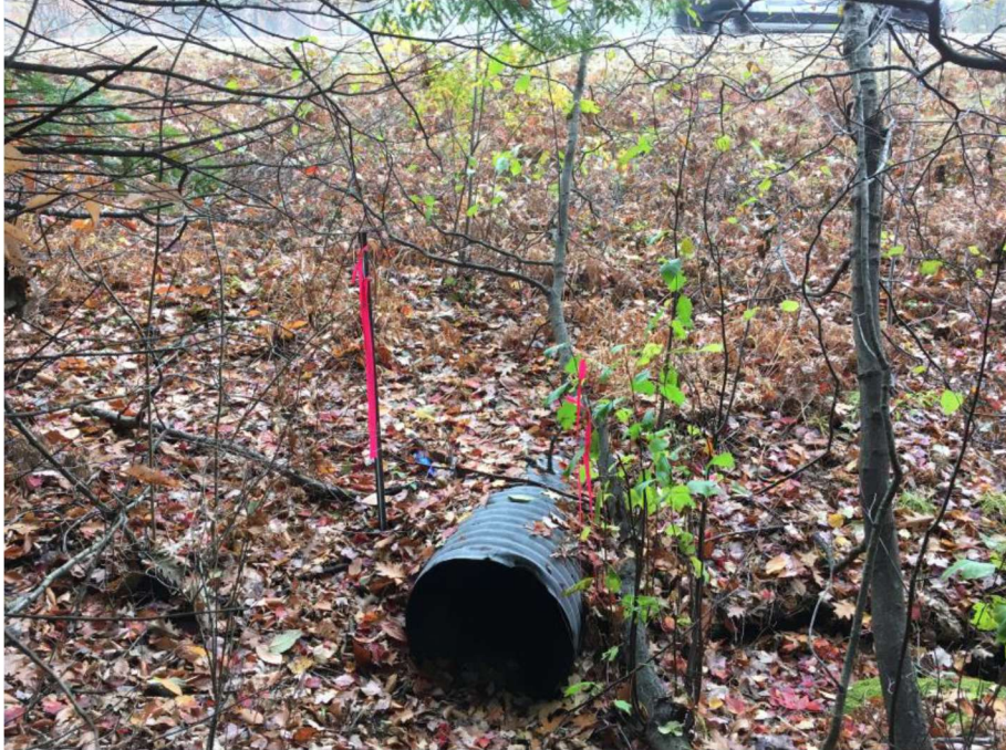
Impact Location Y: Looking towards the inlet of the 24" CMP at approx. Sta. 607 SB Off-Ramp at Exit 10 in Wetland # 156.
