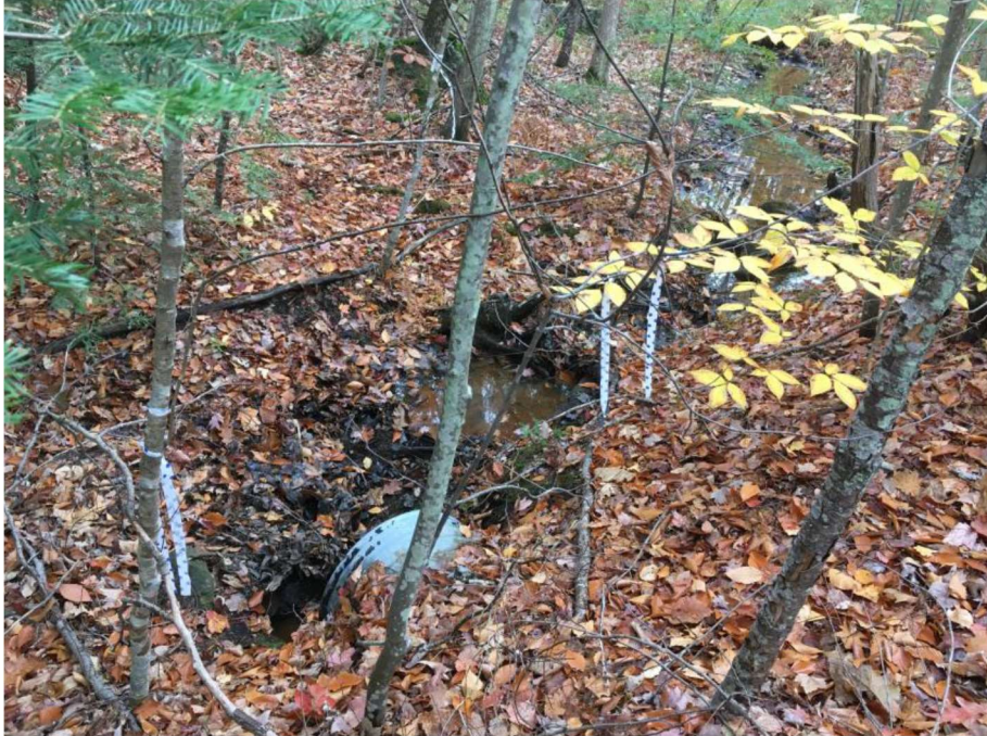
Impact Location AM: Looking away from the outlet of the 24" CMP at approx. Sta. 1546 NB Median in Wetland # 203.
