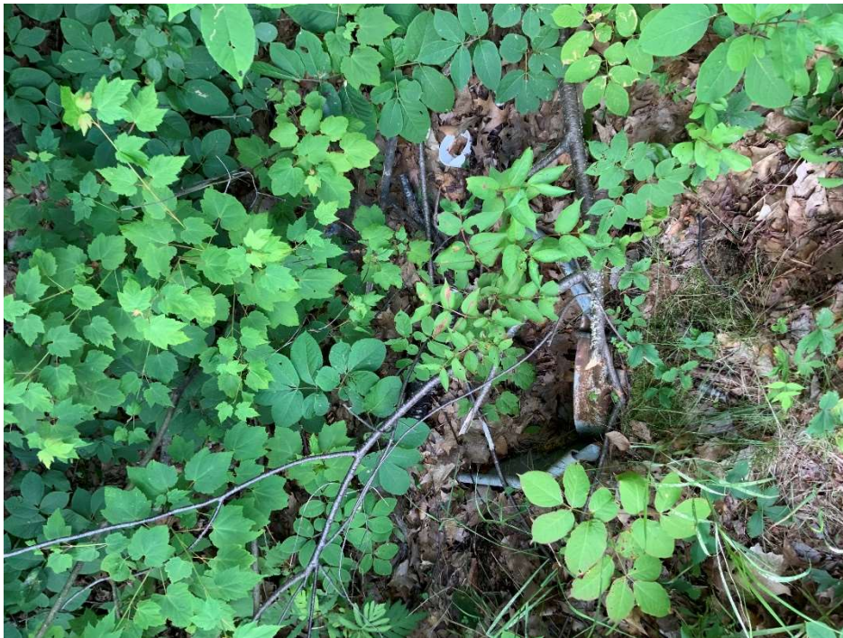
Impact Location A: Looking down at the inlet of the 15" CMP at approx. Sta. 1328 SB in Wetland # 13.
