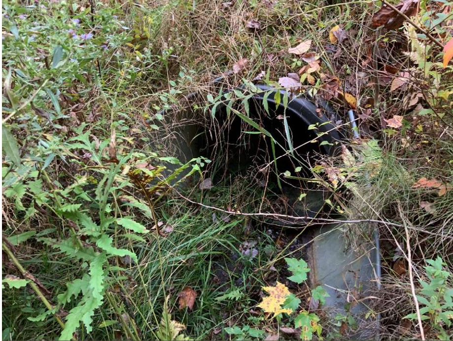
Impact Location K: Looking towards the inlet of the 24" SPP at approx. Sta. 1442 NB in Wetland # 119.
