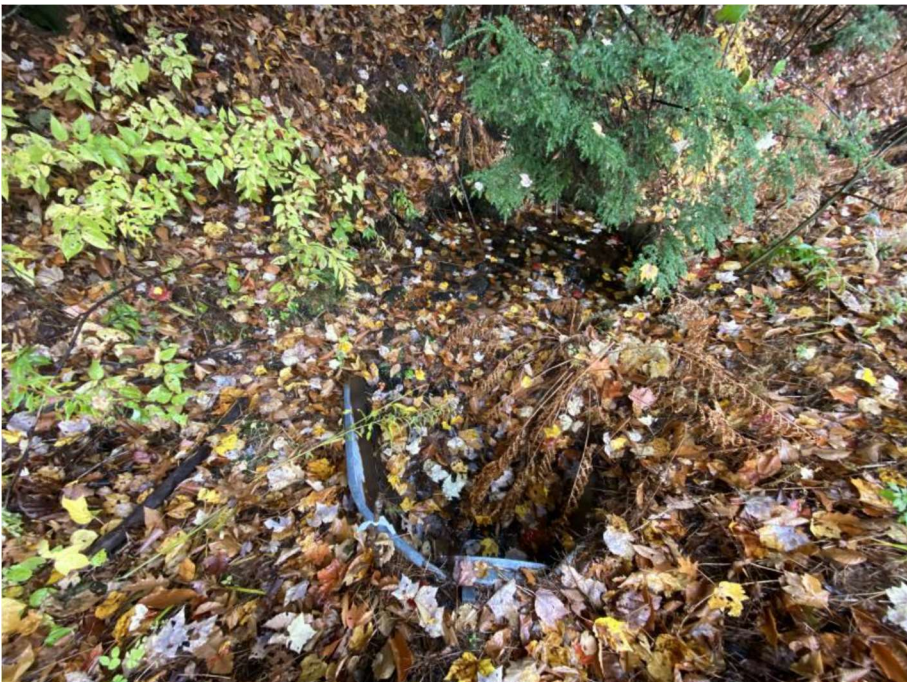
Impact Locations G and H: Looking away from the inlet of the 24" CMP at approx. Sta. 1336 SB in Wetland #s 20 and 26.
