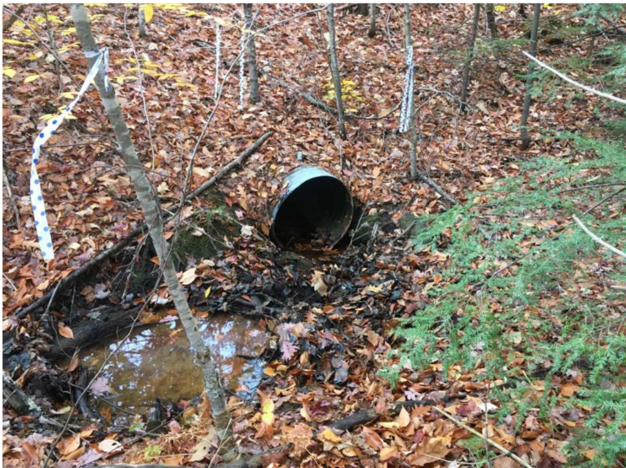
Impact Location AM: Looking towards the outlet of the 24" CMP at approx. Sta. 1546 NB Median in Wetland # 203.
