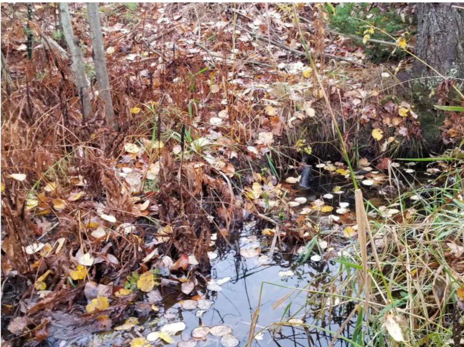
Impact Locations T, U and V: Looking towards the outlet of the 36" CMP at approx. Sta. 308 NB Off-Ramp at Exit 10 in Wetland #s 135, 138 and 140.
