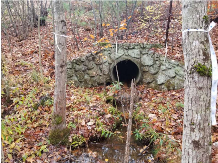
Impact Locations O, P and Q: Looking towards the outlet of the 30" RCP at approx. Sta. 1452 NB in Wetland #s 124, 125 and 126.
