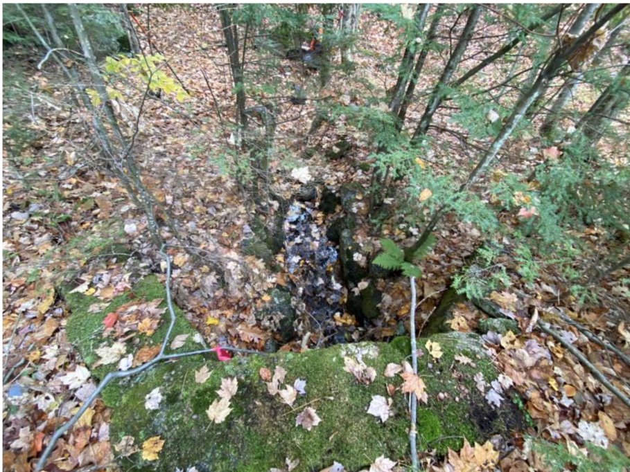
Impact Locations B and C: Looking away from the outlet of the 15" CMP at approx. Sta. 1328 SB Median in Wetland #s 14 and 15.
