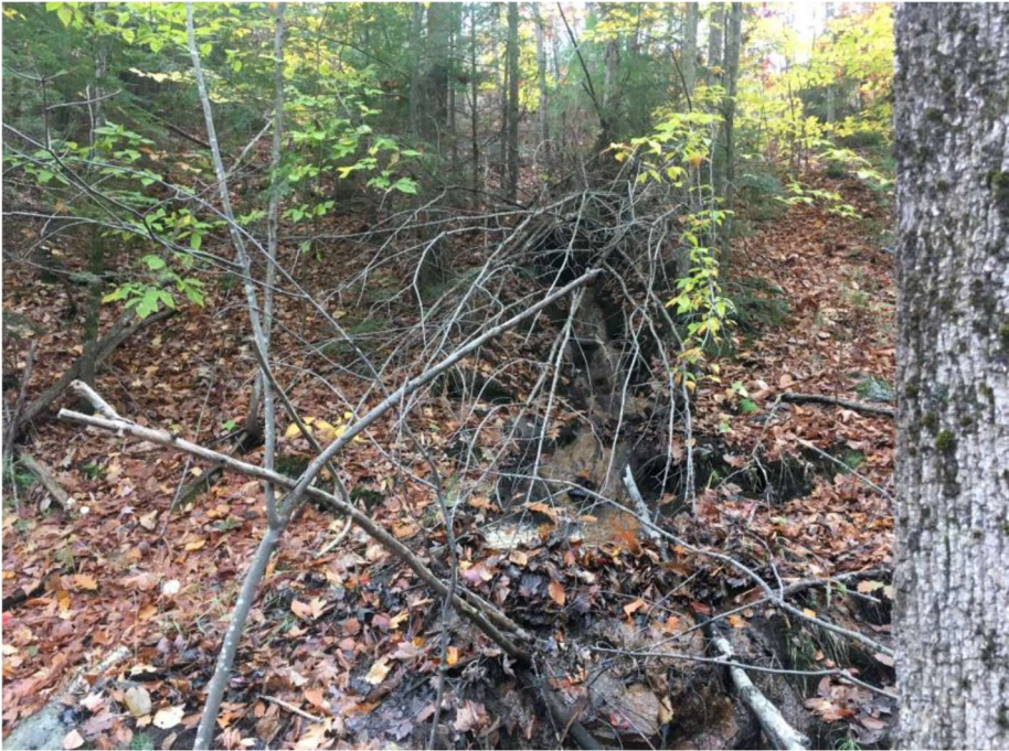
Impact Location AL: Looking towards the outlet of the 24" CMP at approx. Sta. 1546 NB in Wetland # 203.
