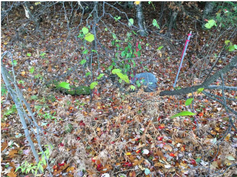
Impact Location Y: Looking away from the inlet of the 24" CMP at approx. Sta. 607 SB Off-Ramp at Exit 10 in Wetland # 156.
