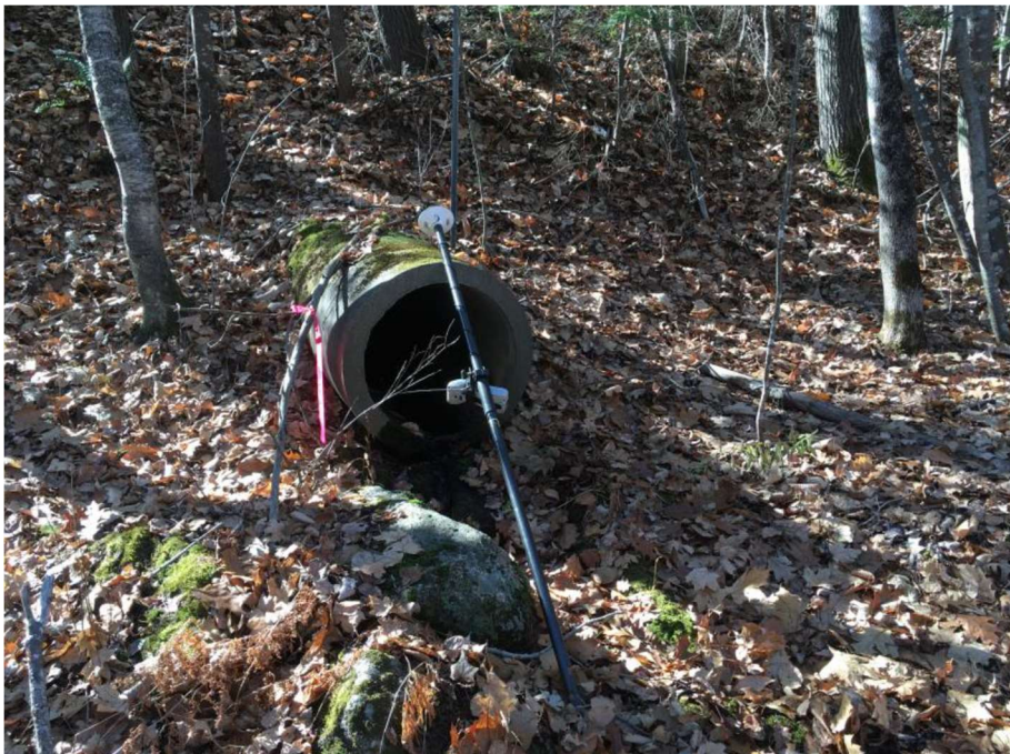
Impact Location AO: Looking towards the inlet of the 24" RCP at approx. Sta. 1542 SB in Wetland # 200.
