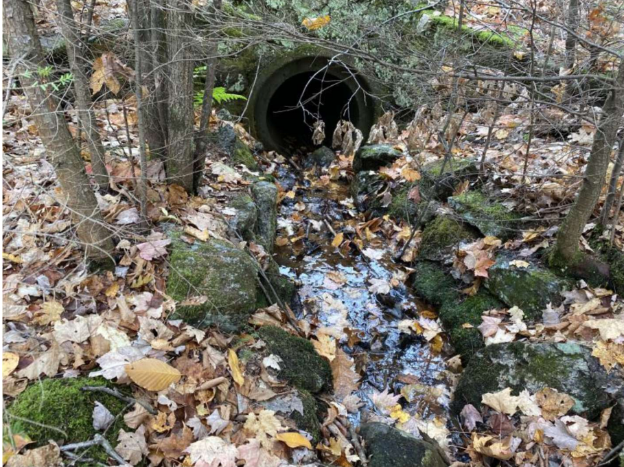
Impact Locations B and C: Looking towards the outlet of the 15" CMP at approx. Sta. 1328 SB Median in Wetland #s 14 and 15.
