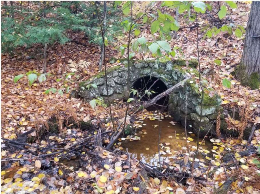
Impact Locations R and S: Looking towards the inlet of the 36" CMP at approx. Sta. 1463 NB Median in Wetland #s 137 and 138.
