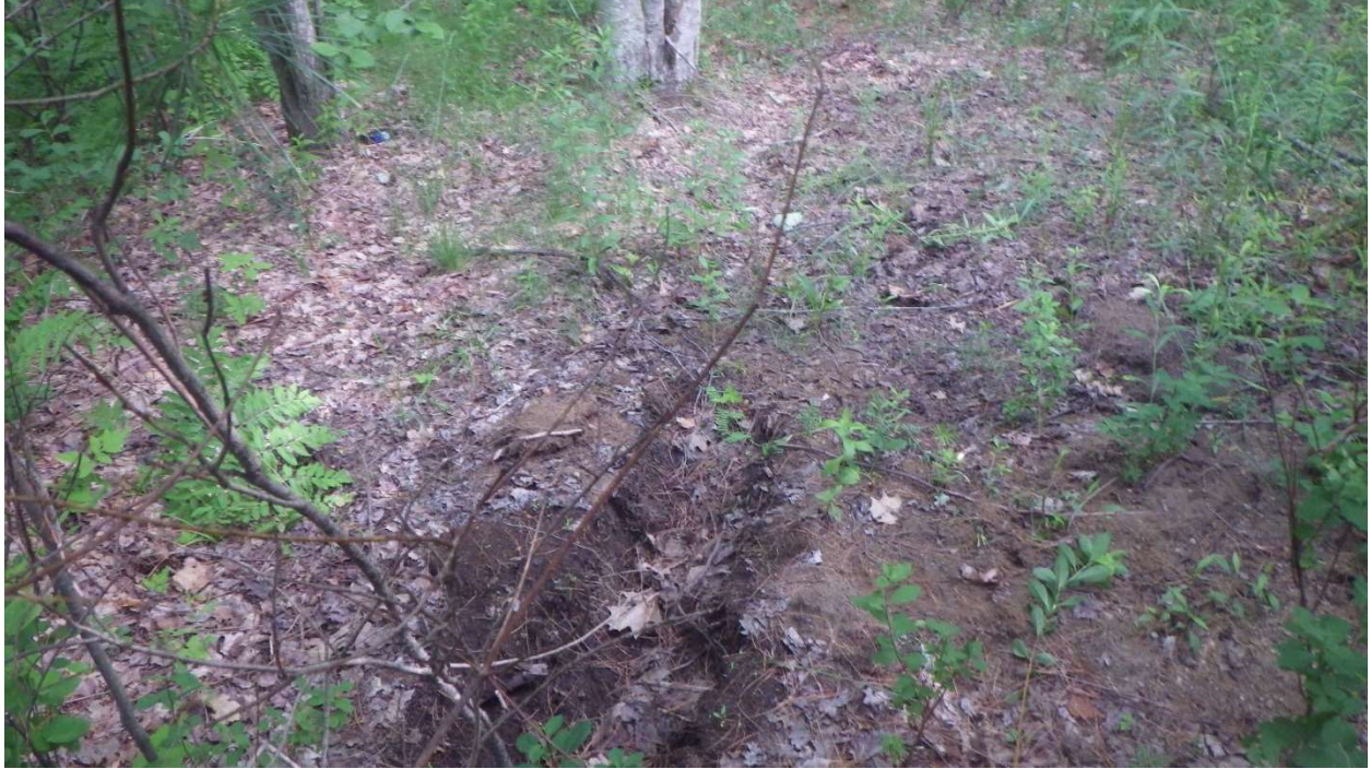
Impact Location N: Looking away from the outlet of 12" CMP at approx. Sta. 1450 NB in Wetland #123.
