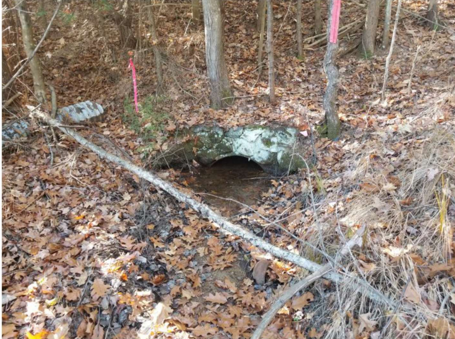
Impact Location I: Looking towards the inlet of the 30" CMP at approx. Sta. 1401 SB Median in Wetland # 90.
