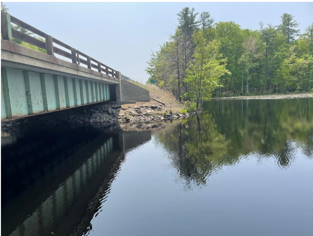
Photo 16: SW Bridge Quadrant from NW Bridge Quadrant facing South (May 2023) IMPACT AREA: A / TC / TD
