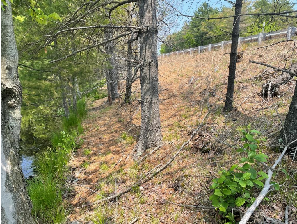
Photo 17: NW Bridge Quadrant Existing Causeway Slope (May 2023) IMPACT AREA: TF / TG / D
