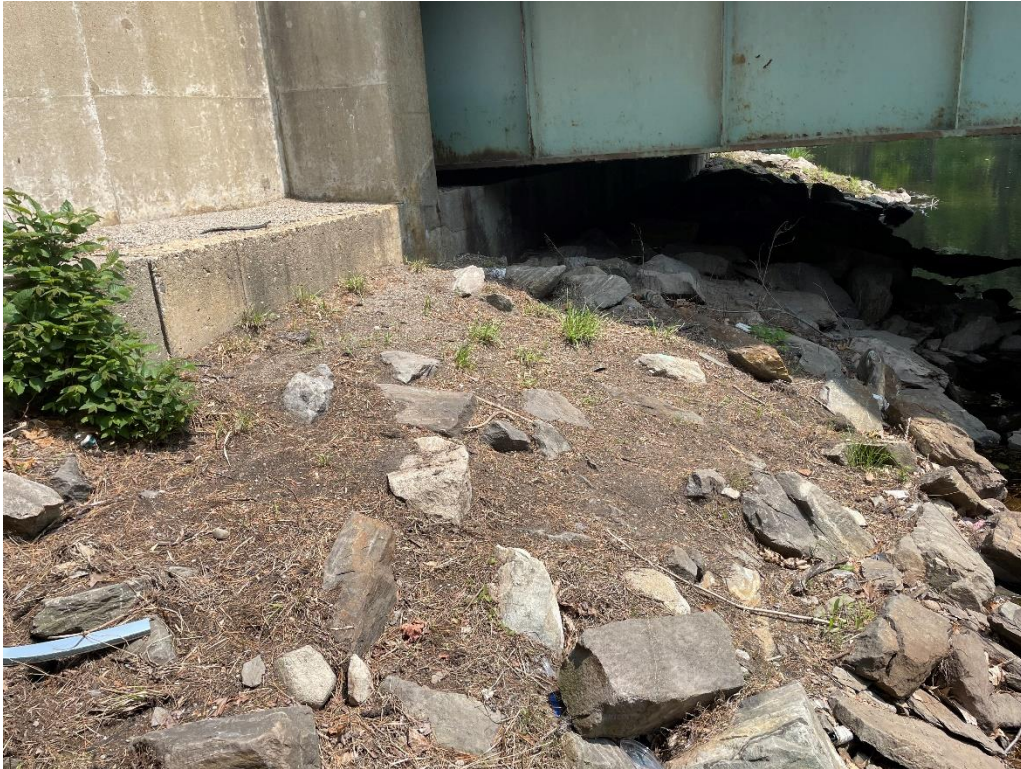
Photo 15: Northern Bridge Abutment NW Bridge Quadrant facing East (May 2023) IMPACT AREA: D
