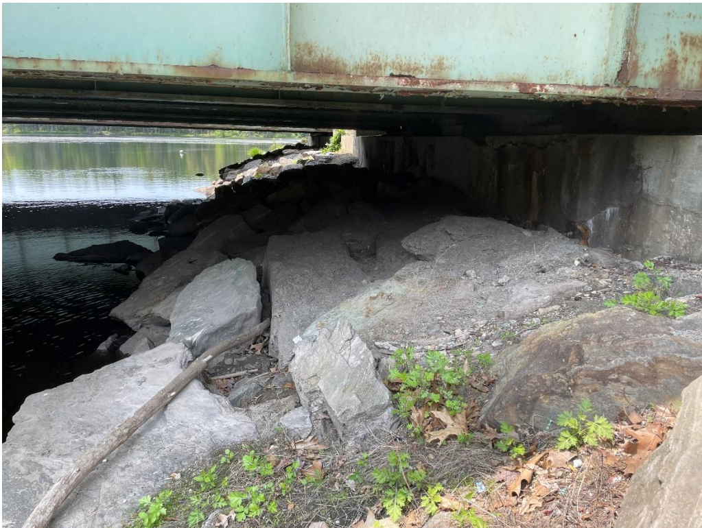
Photo 14: Northern Bridge Abutment NE Bridge Quadrant facing West (May 2023) IMPACT AREA: D
