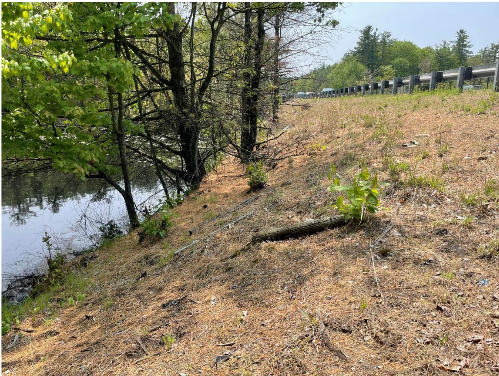
Photo 12: NE Bridge Quadrant Causeway Slope (May 2023) IMPACT AREA: C/ D
