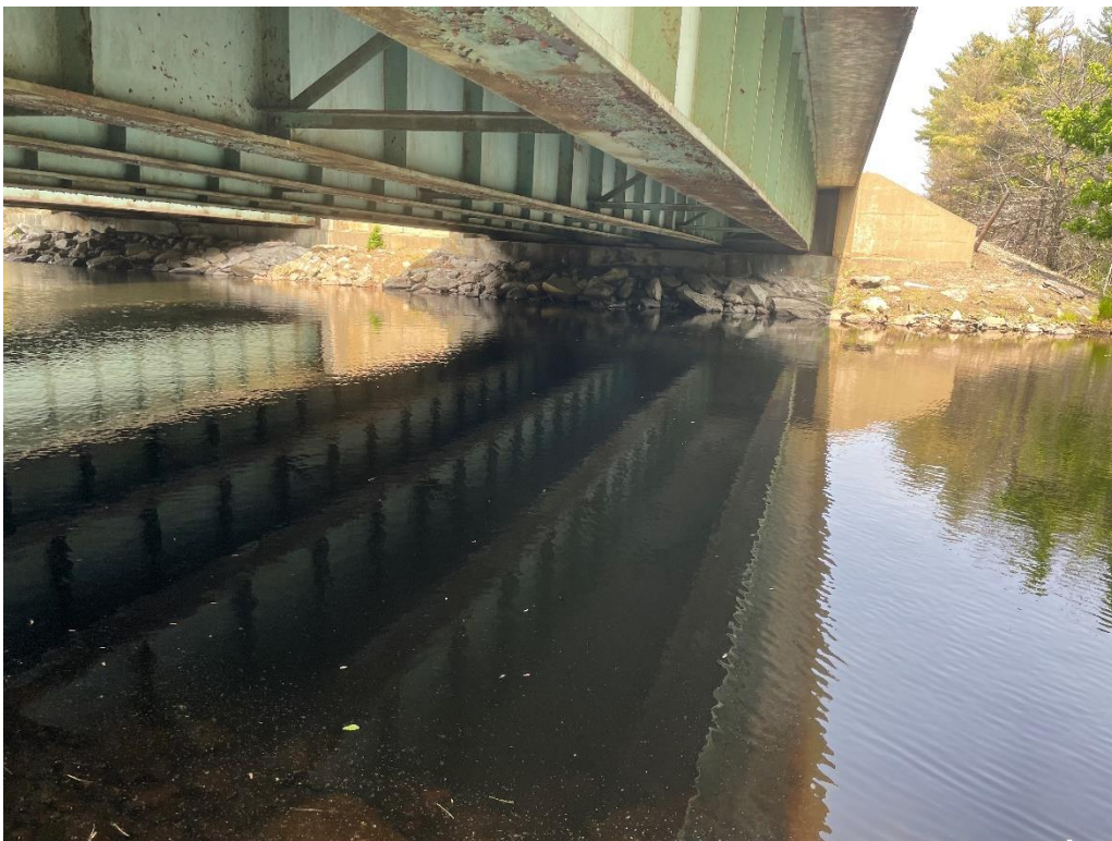
Photo 8: Pennichuck Brook Crossing facing North from SE Bridge Quadrant (May 2023) IMPACT AREA: C / D / TD
