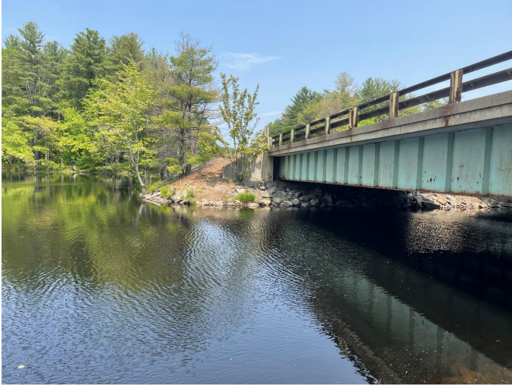
Photo 9: Pennichuck Brook Crossing facing North from SW Bridge Quadrant (May 2023) IMPACT AREA: D / E/ TD / TF
