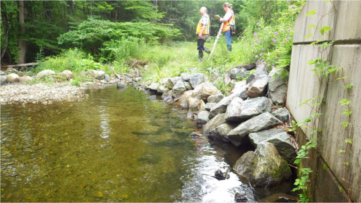
8. Existing rip rap, outlet side bank right (2021)
