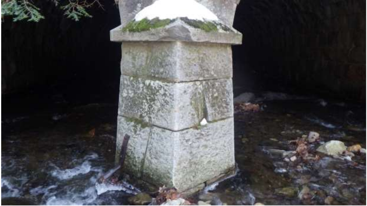
Figure 27. Looking west at center pier with pointed ends on spandrel wall at eastern end (inlet) from upstream
