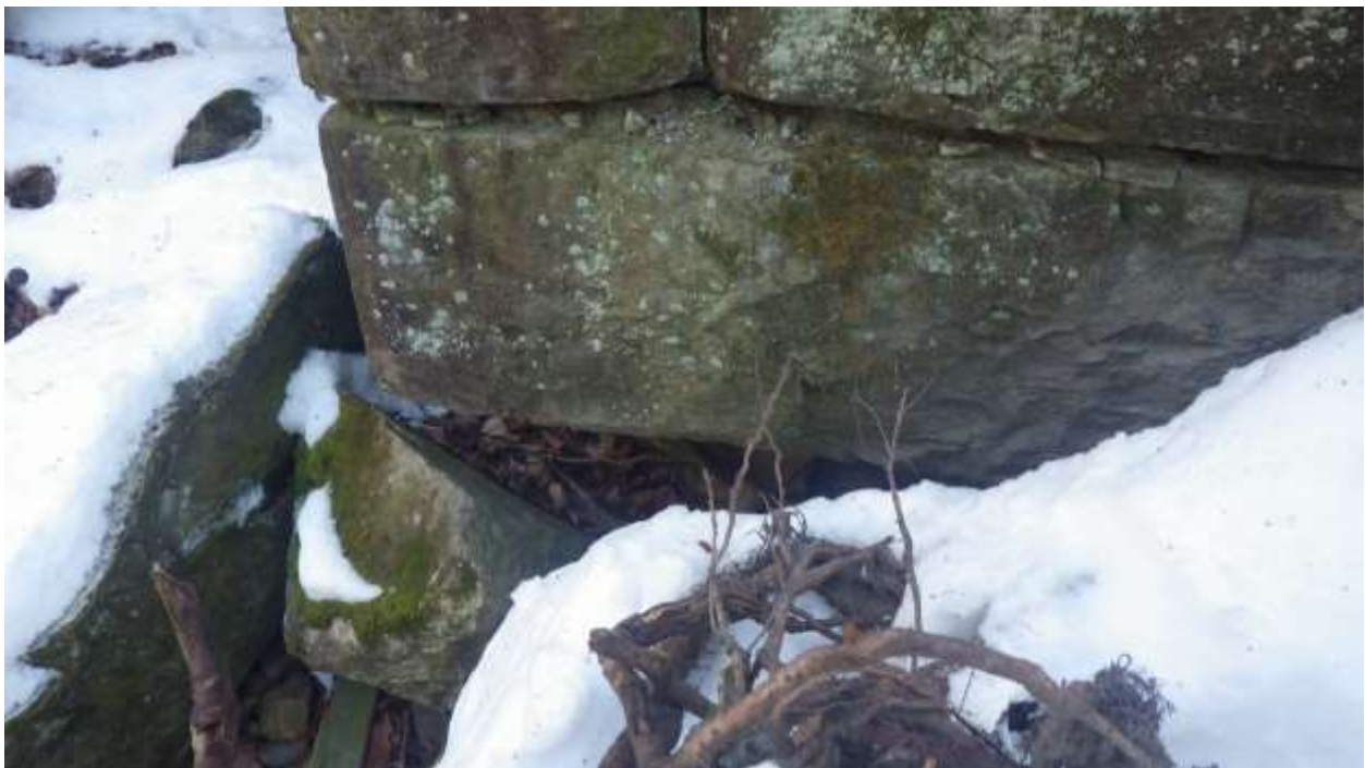
Figure 14. Looking east at stone displacement at base of southwest wingwall
