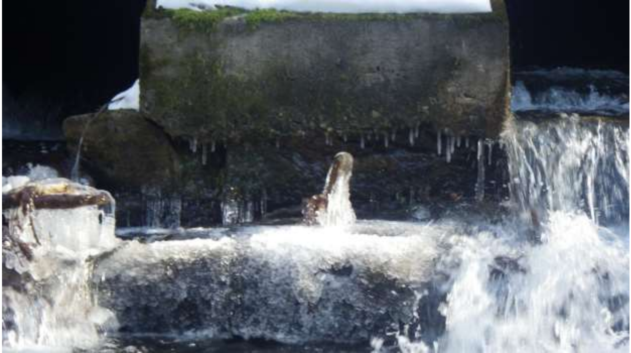
Figure 7. Looking east at the base of outlet center buttress support from downstream
