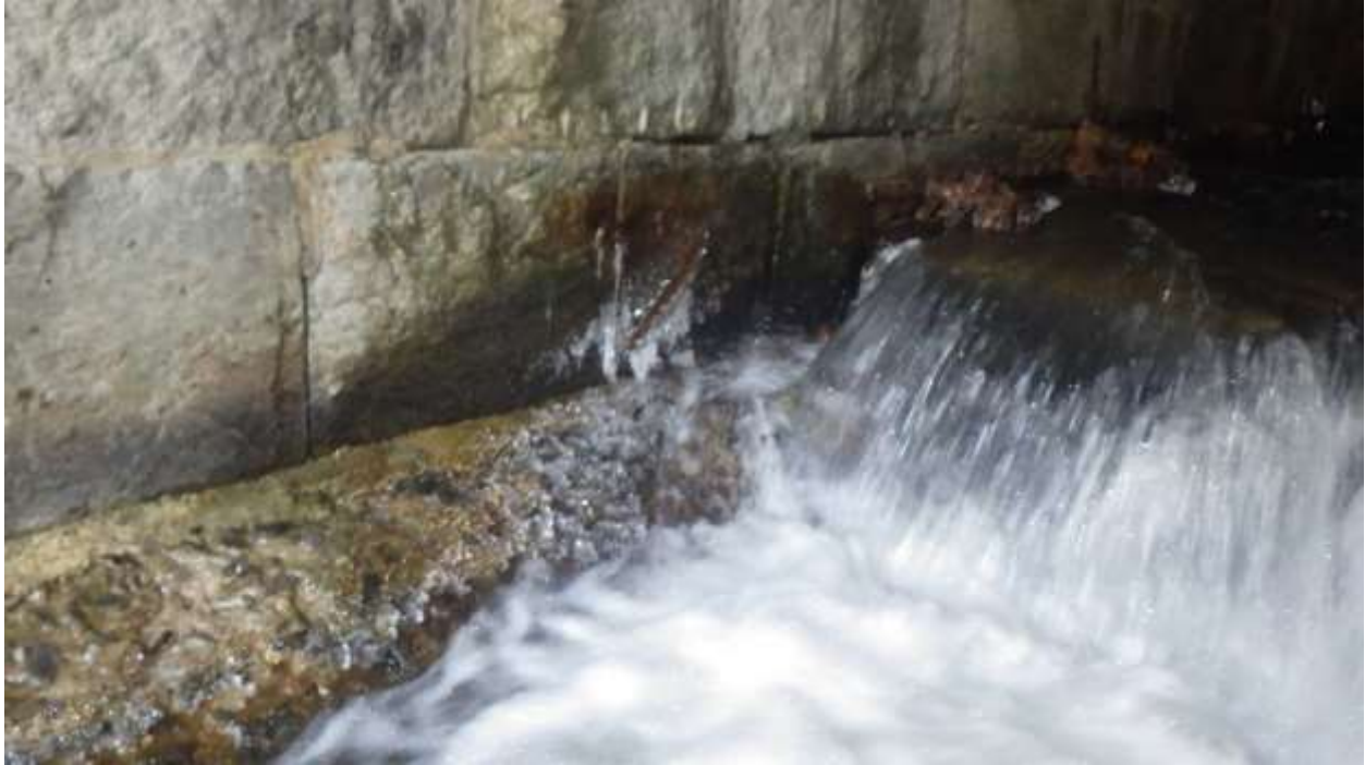
Figure 19. View of northern sidewall of the north barrel showing where the stone floor washed away and undermining of the concrete toe wall installed in 2014
