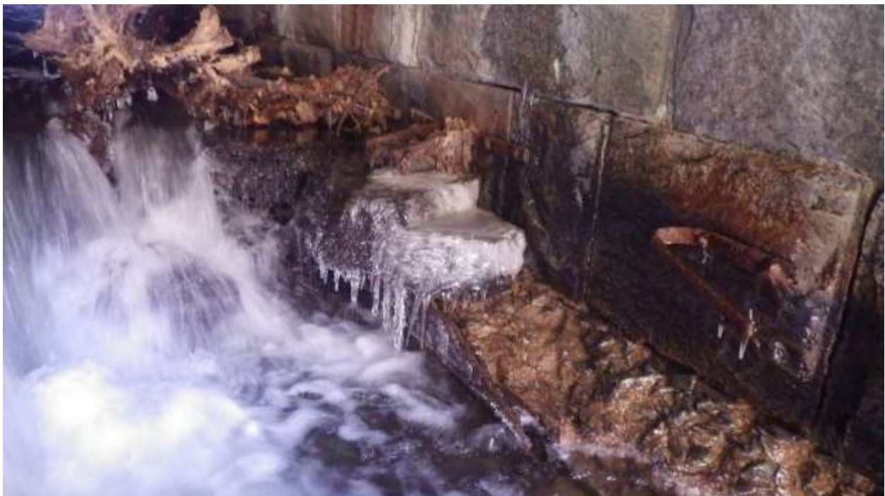
Figure 18. View of the southern sidewall of the north barrel showing where the stone floor has washed away and undermining of the concrete toe wall installed in 2014
