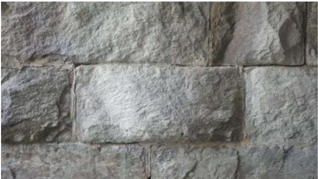
Figure 20. View of typical stone used throughout the structure measuring 1'8" tall and 4' long, looking at the northern sidewall of the north barrel
