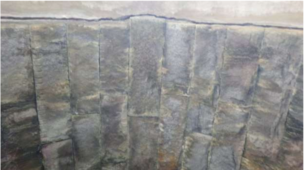
Figure 16. View of the keystone at the western end (outlet) of the north barrel
