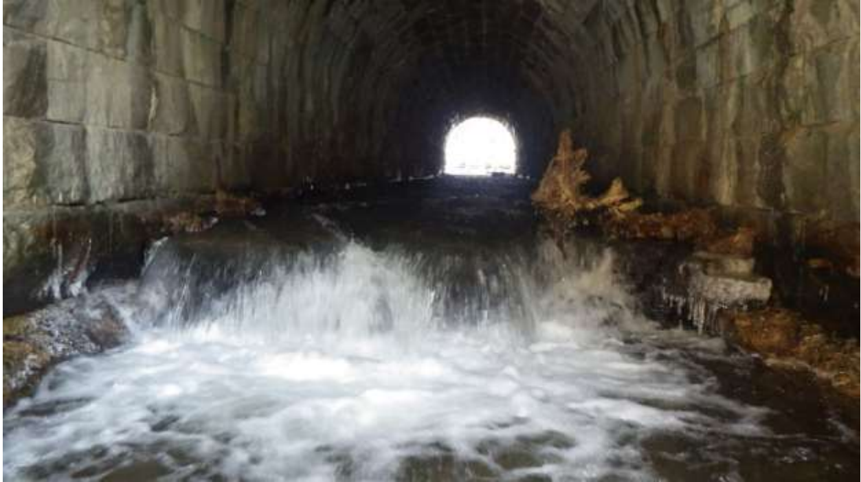
Figure 17. Looking east through the north barrel at the 3' drop located 30' into the structure where the stone floor washed away and revealed the original concrete floor
