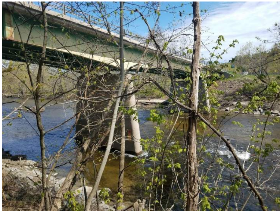
Photo 2: View of Bridge 072/127 from the southeast quadrant on the West Bank Side
