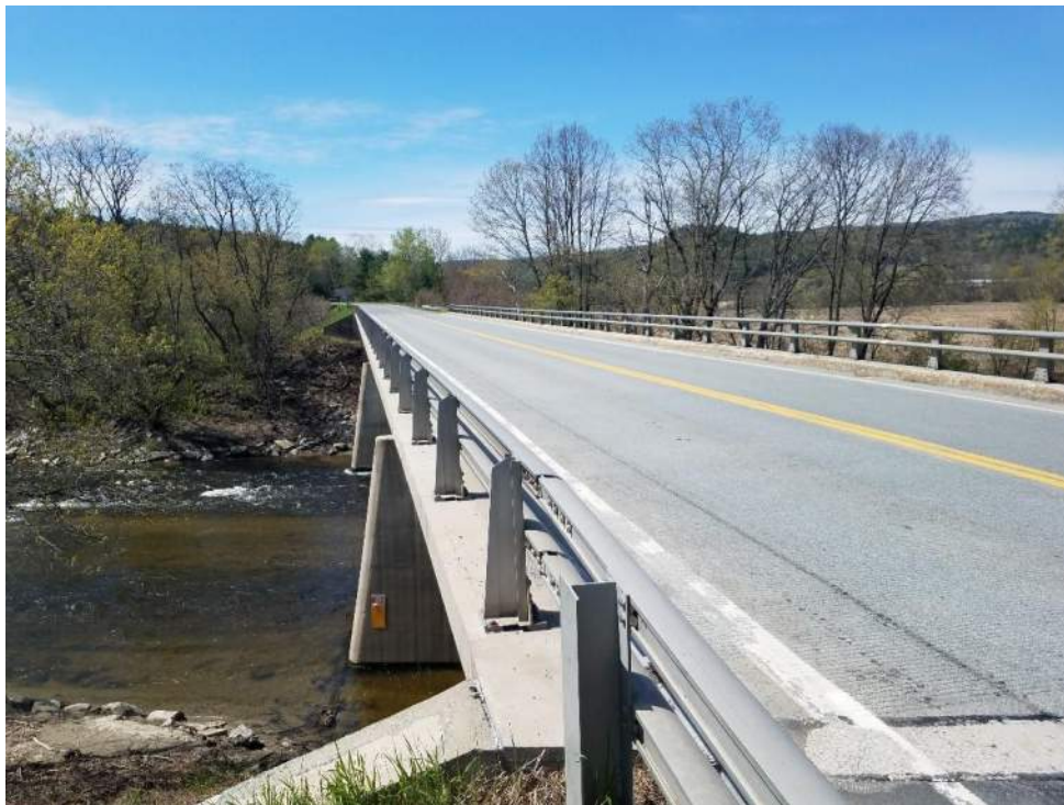
Photo 6: View of Bridge 072/127 from the northeast quadrant on the East Side Bank
