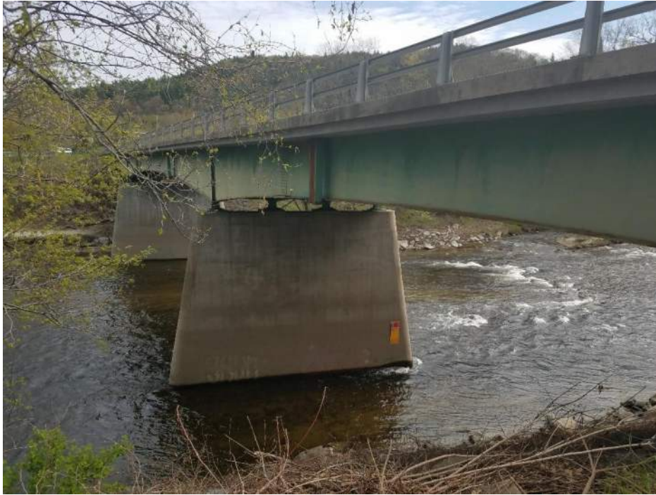
Photo 1: View of Bridge 072/127 from the southwest quadrant on the West Bank Side
