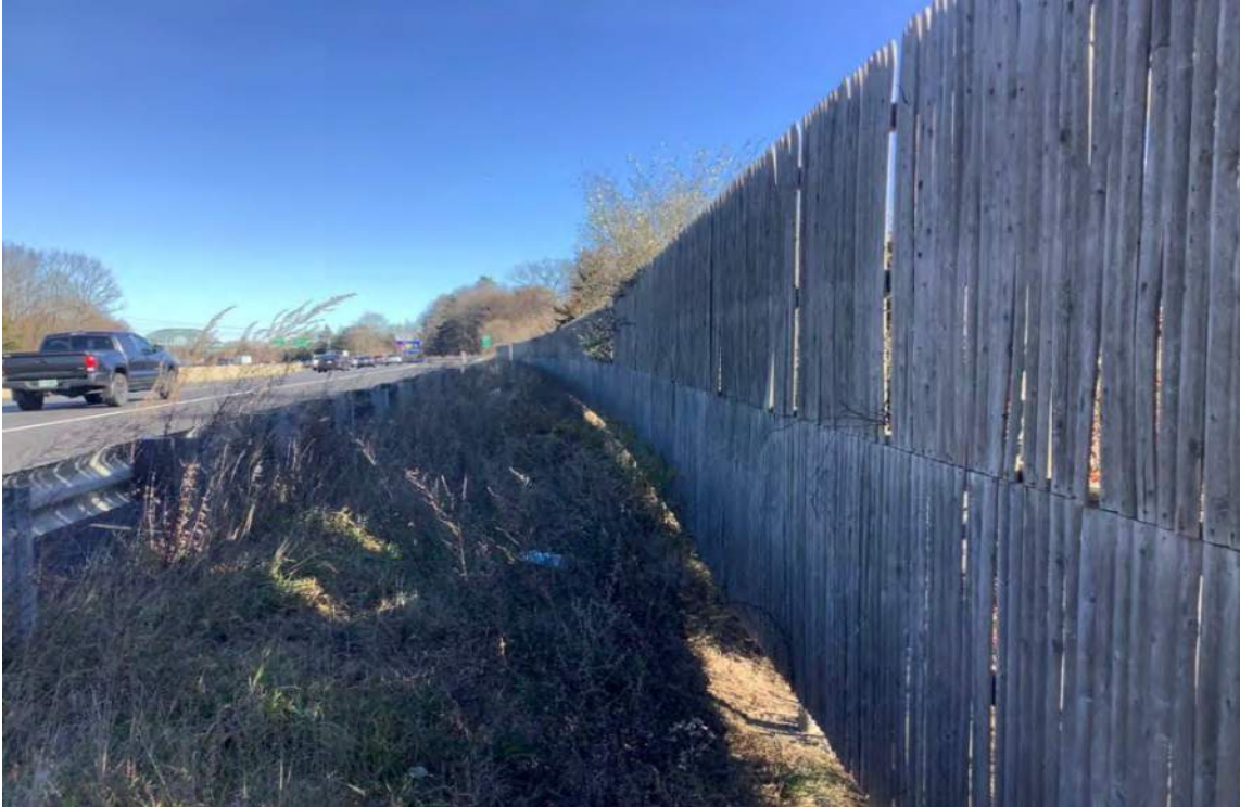
Photo 7: View northeast of the existing wooden fence near the New Franklin School.
