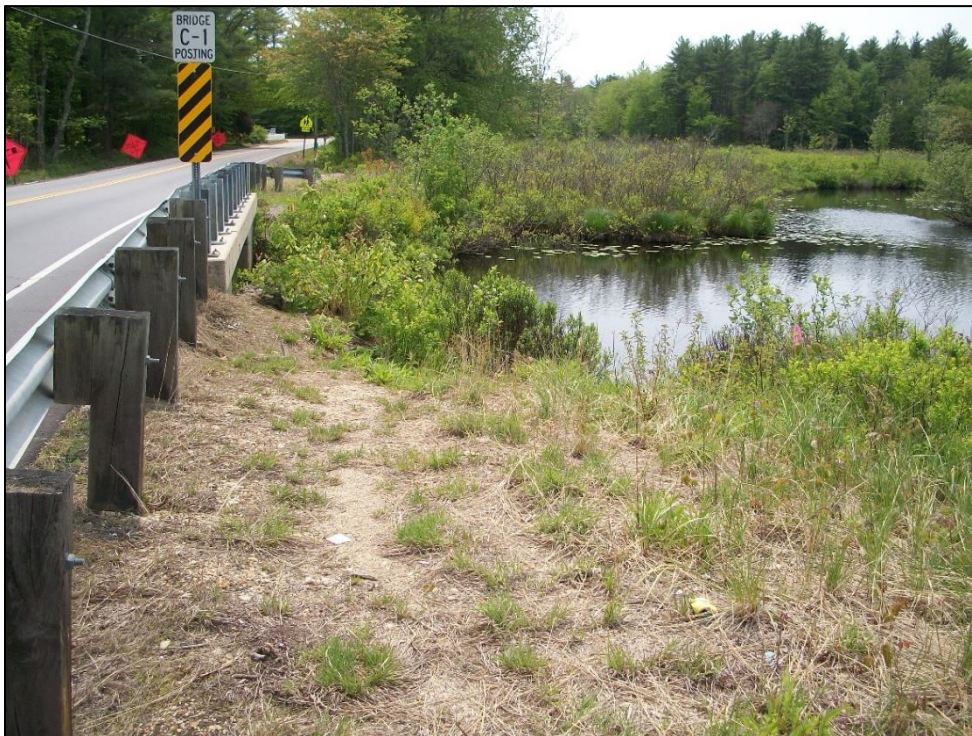
Photo 4. View south of Bridge No. 141/127, looking toward west/downstream side of bridge. Photo taken on 5/31/2019.
