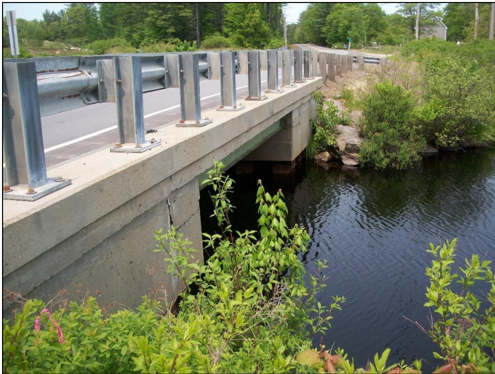
Photo 2. View northwest of Bridge No. 141/127, looking toward northeast bridge quadrant. Photo taken on 5/31/2019.
