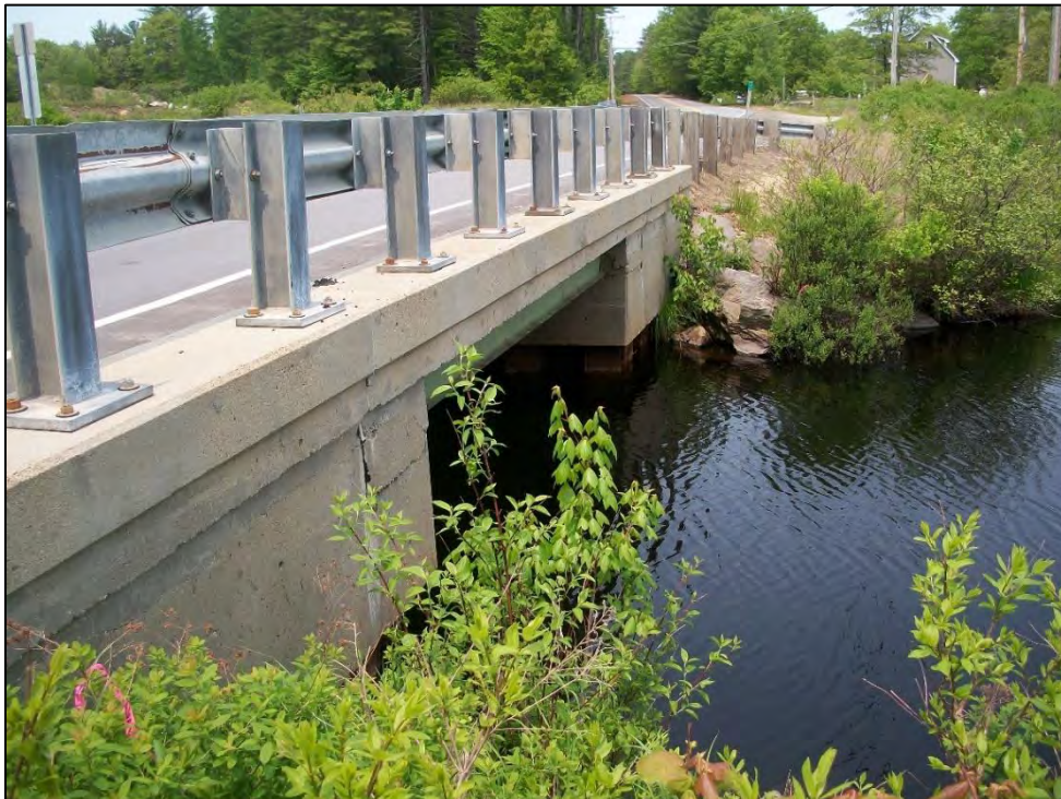
Photo 2. View northwest of Bridge No. 141/127, looking toward Impact Areas C and F (east/upstream side of bridge). Photo taken on 5/31/2019.
