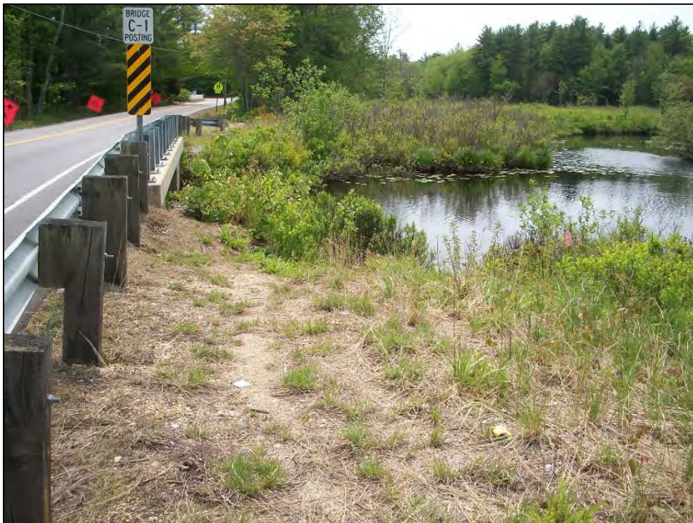
Photo 4. View south of Bridge No. 141/127, looking toward Impact Areas G, H, I, J, K, and L (west/downstream side of bridge). Photo taken on 5/31/2019.
