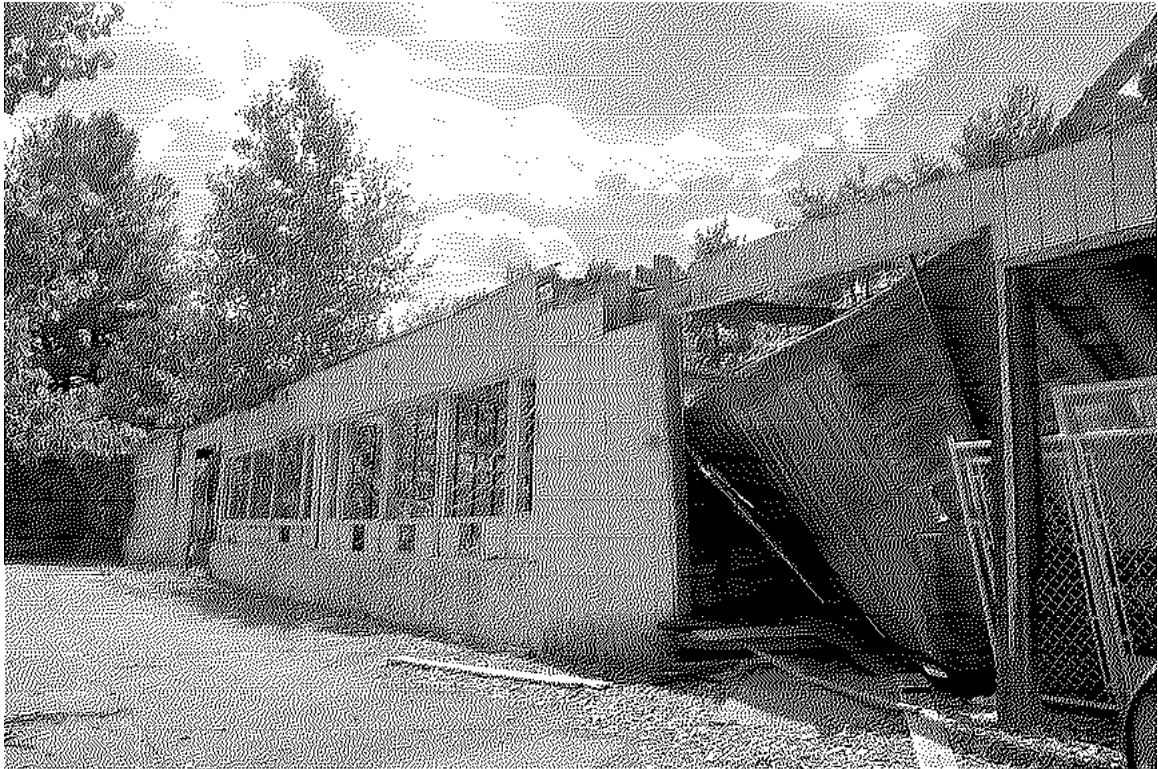
Photo 03: Equipment Shed, 22 Pillsbury Rd., roof collapsed (LON-WO, Woodmont Orchard Historic District)
