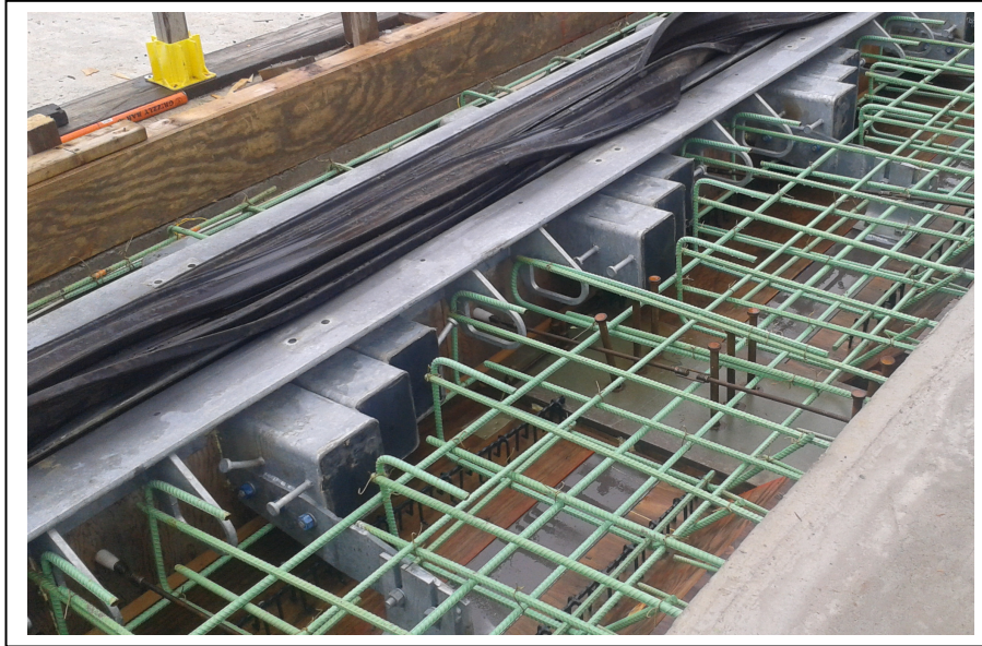
Modular Expansion Joint Reinforcing
