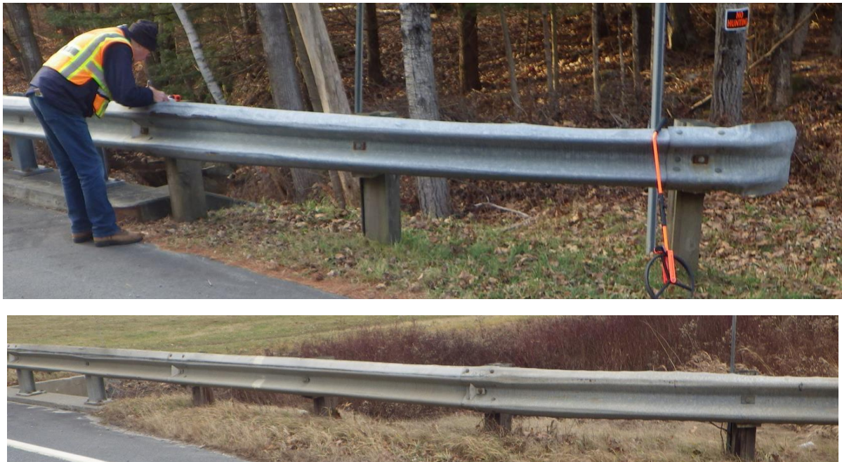
Figure 2 – Examples of W-Beam Bridge Rail in Need of Transition
