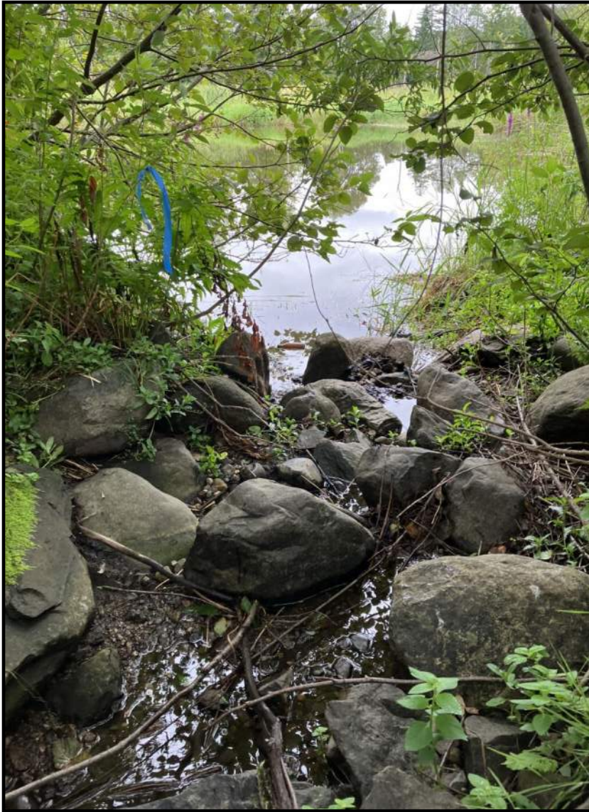
Photo 5: Looking downstream at apparent riprap stacked as channel outlets into emergent wetland/Fire Pond.
