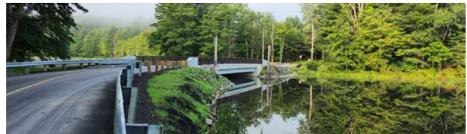
MassDOT hired CHA to replace the Champeaux Rd. Bridge over Long Pond in Sturbridge, MA. The bridge required total replacement due to structural deficiencies. Our innovative design featured an integral abutment bridge supported by micropiles.
