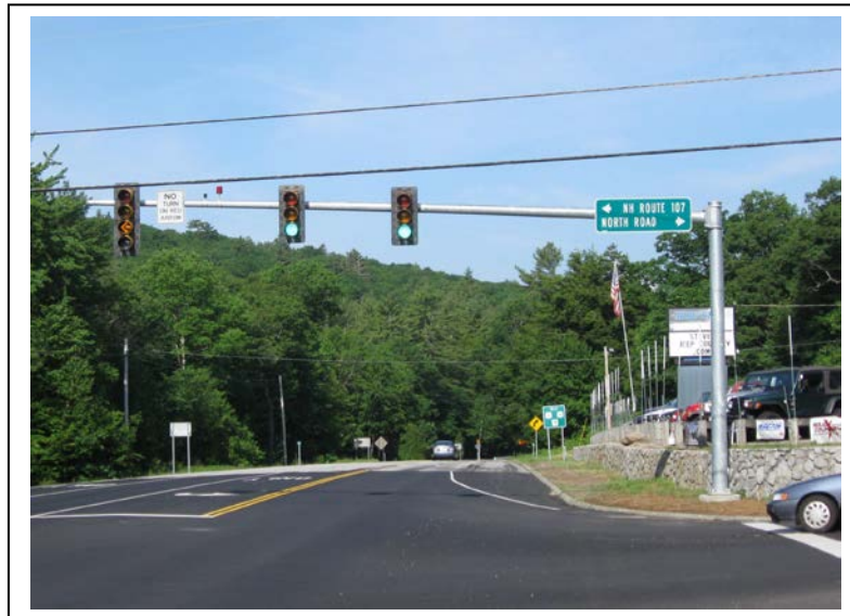
Typical NHDOT Traffic Signal Support (Mast Arm)
