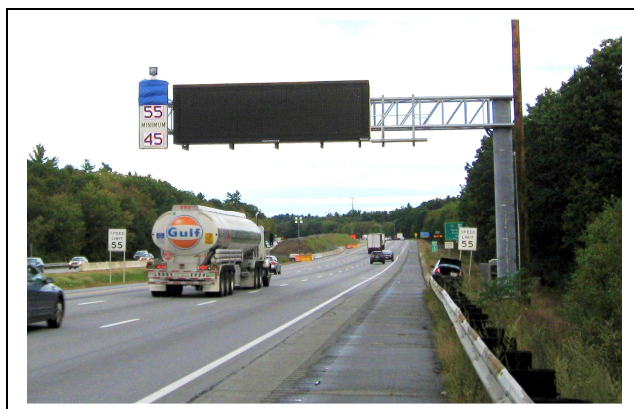
Typical NHDOT DMS Overhead Structure
