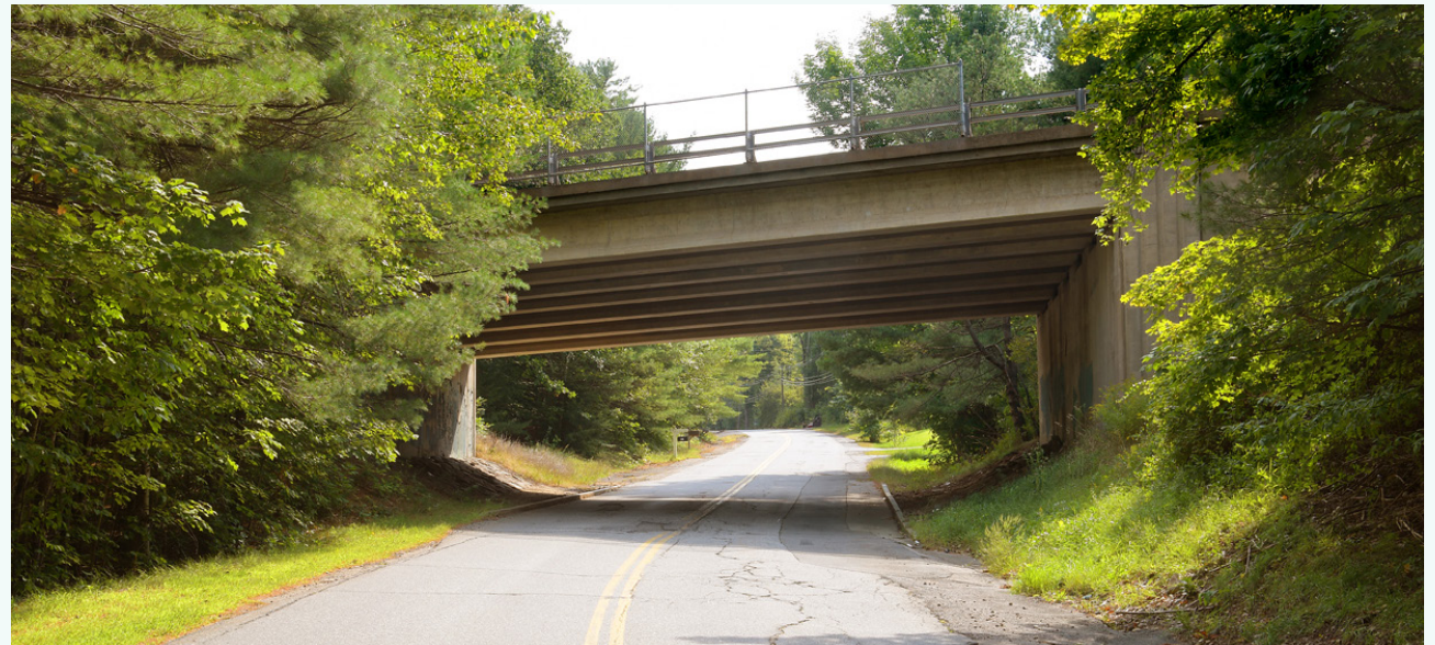
2021 view of US Route 3-NH Route 11 Bridge over Mile Hill Road, north elevation, facing south (Preservation Company)
