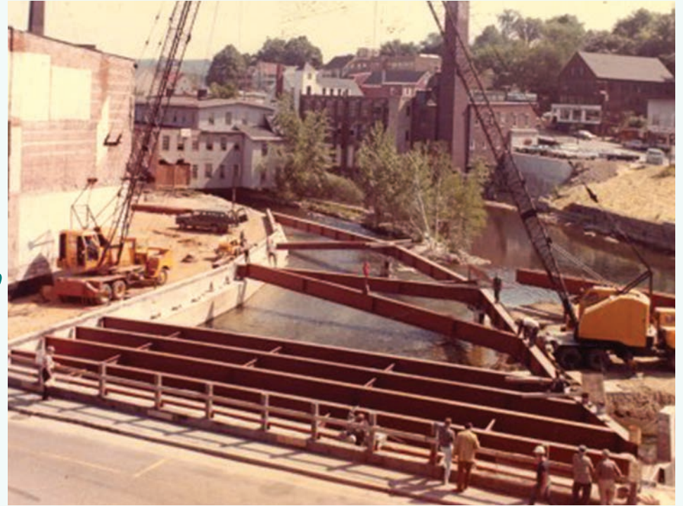
Beacon Street East under construction in 1969, facing northeast, with old Main Street Bridge in foreground (Laconia Public Library)
