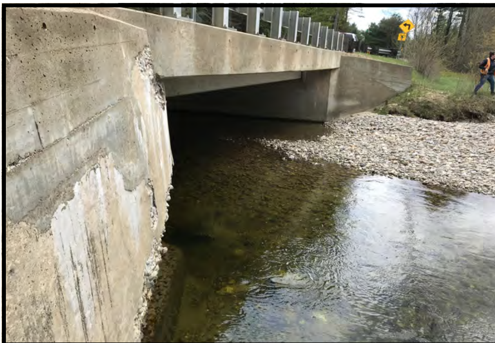
PHOTO 26: This is a view of the outlet of the crossing structure at site 7.
