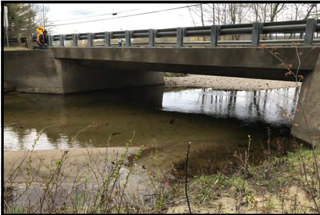
PHOTO 25: This is a view of the inlet of the crossing structure at site 7.
