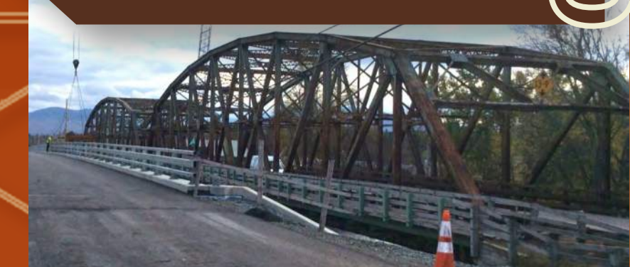
Construction view showing the new steel girder bridge (left) and the Parker truss bridge prior to demolition, 2020.
