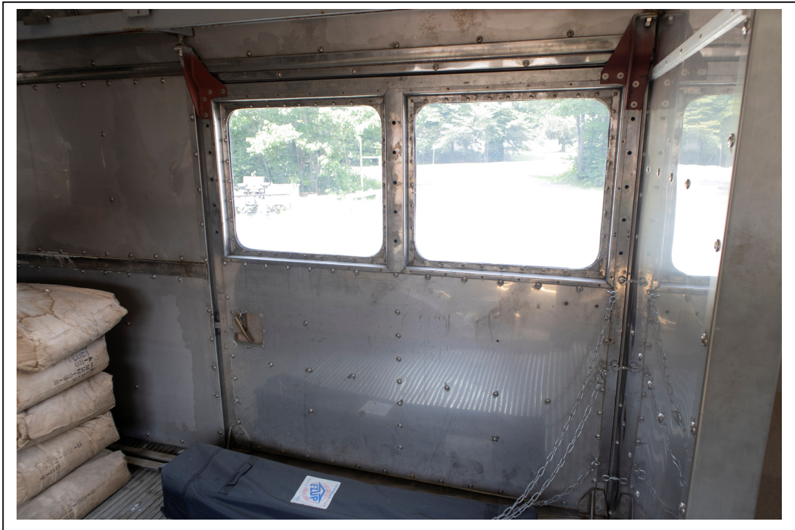
Photo 20. Car A, baggage compartment, view looking north at sliding baggage door (Carly Adler, photographer 7/20/23; HRI Neg. #23056 D2:3).
