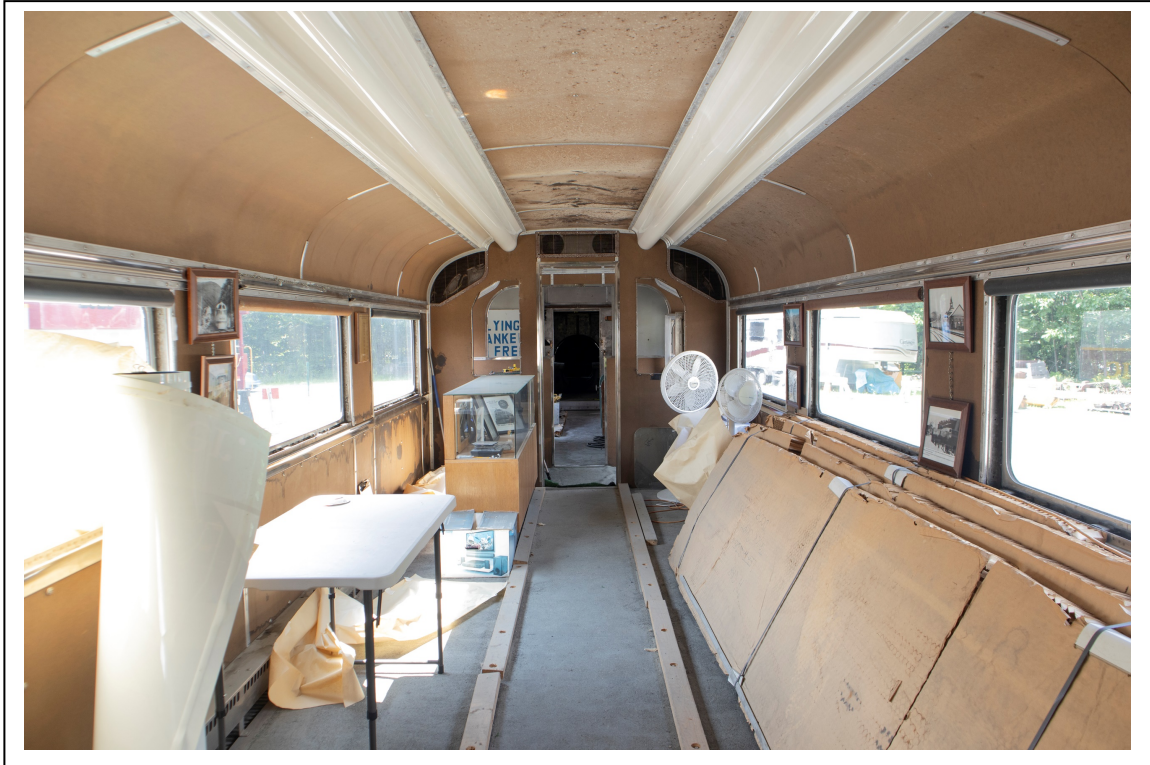
Photo 22. Car A, passenger compartment, view looking southeast toward rear of train (Carly Adler, photographer 7/20/23; HRI Neg. #23056 D2:55).
