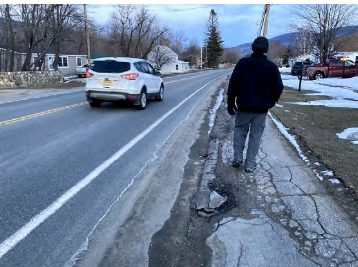
Sidewalk with cracks, loose pavement, holes, no elevation, etc.
