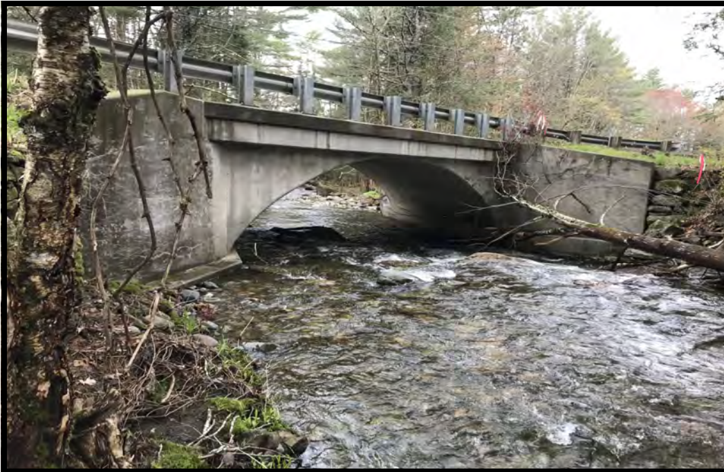
PHOTO 13: This is a view of the inlet of the crossing structure at site 4.
