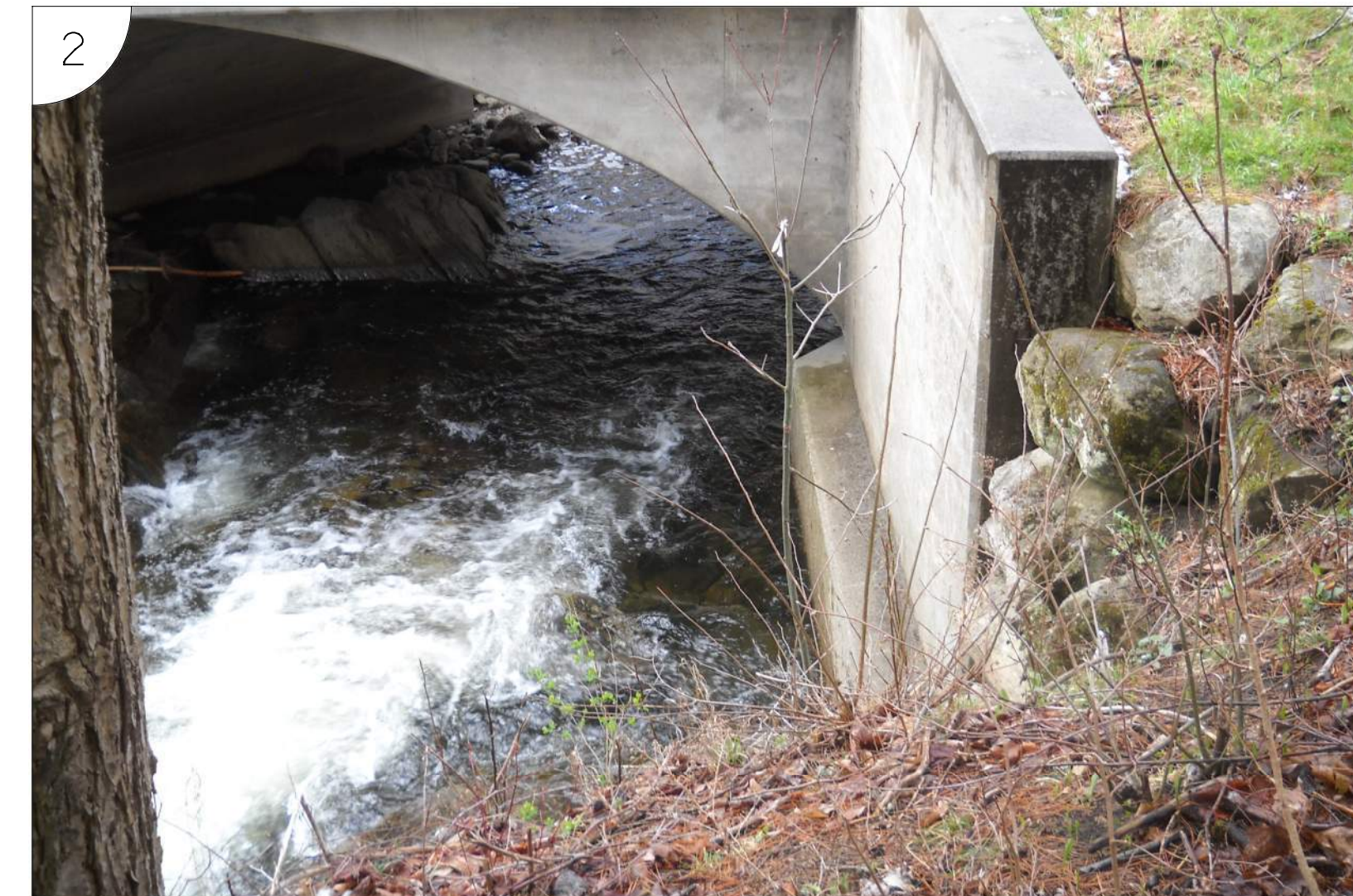
SCOUR AREA LOOKING WEST
