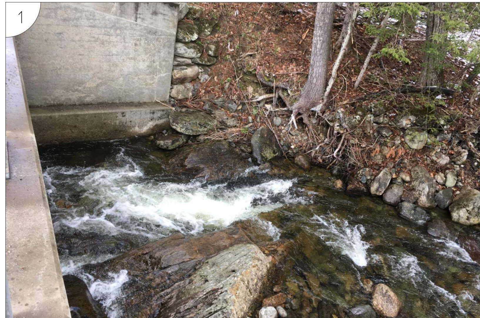
SCOUR AREA LOOKING NORTH
