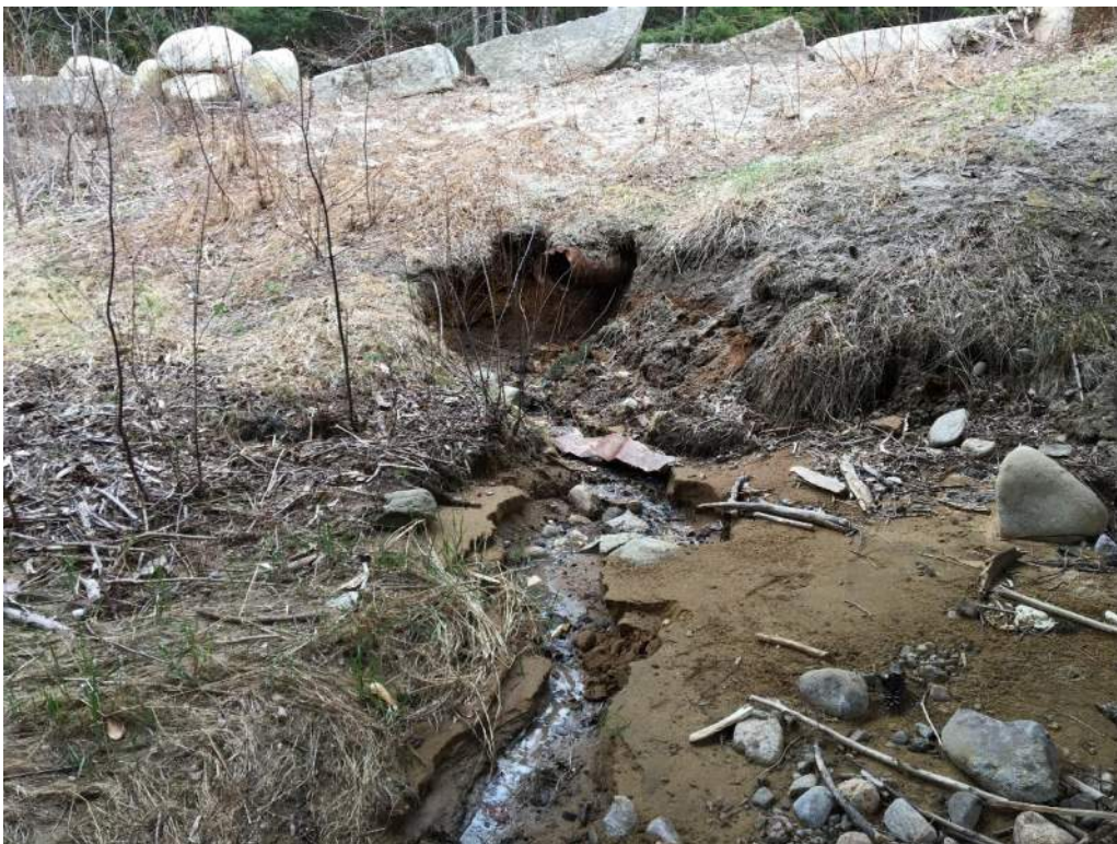
Photo 9: IMPACT AREA: E – Bank behind southern bridge pier showing erosion/scour from existing drainage outfall (05/06/2020) Photo Direction: SE
