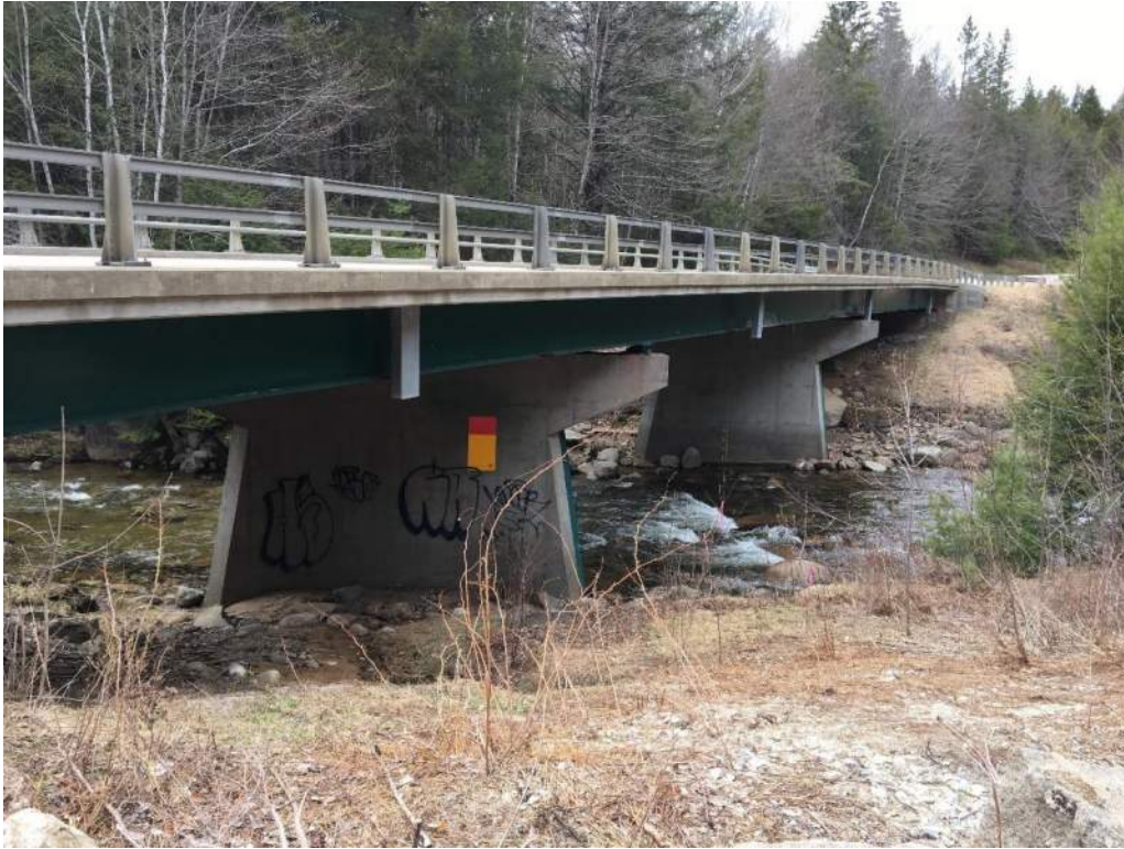
Photo 10: IMPACT AREA: E & G Bridge No. 061/091 carrying NH Route 113A over the Swift River (05/06/2020) Photo Direction: NE
