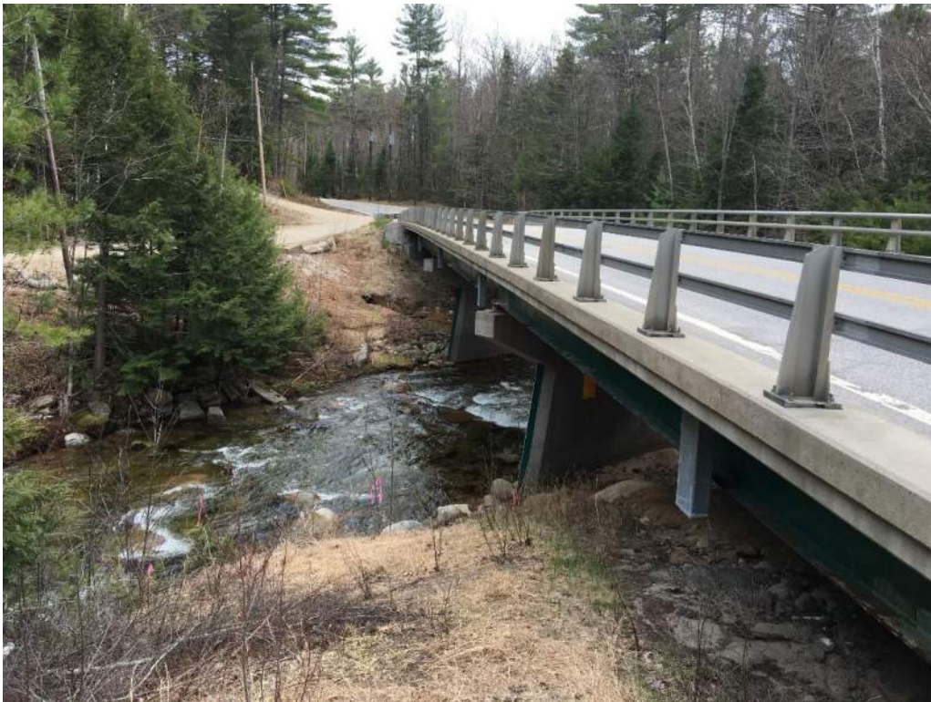
Photo 3: IMPACT AREA: G & E – Waterfront Buffer – NE bridge quadrant (G) in foreground / SE Bridge quadrant (E) opposite side of Swift River (05/06/2020) Photo Direction: S
