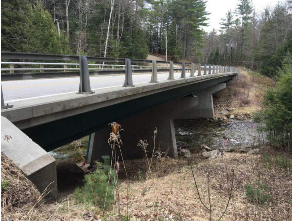
Photo 4: IMPACT AREA: G & E – Waterfront Buffer - Bank behind northern bridge pier (05/06/2020) Photo Direction: W
