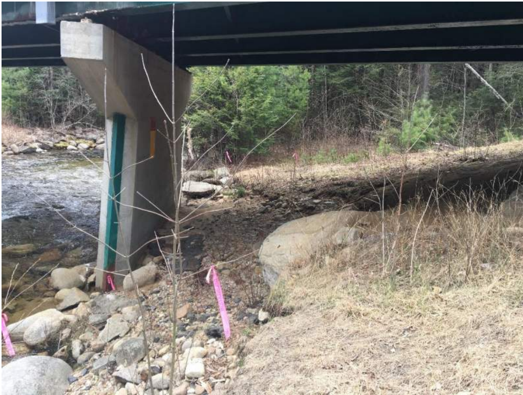
Photo 1: IMPACT AREA: G – Waterfront Buffer - Northern bridge pier facing downstream (05/06/2020) Photo Direction: W
