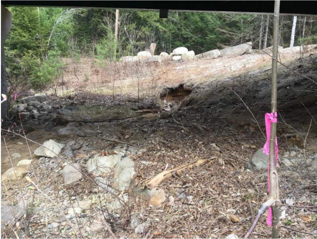
Photo 8: IMPACT AREA: A/E/B – Bank behind southern bridge pier and existing drainage outfall (05/06/2020) Photo Direction: E
