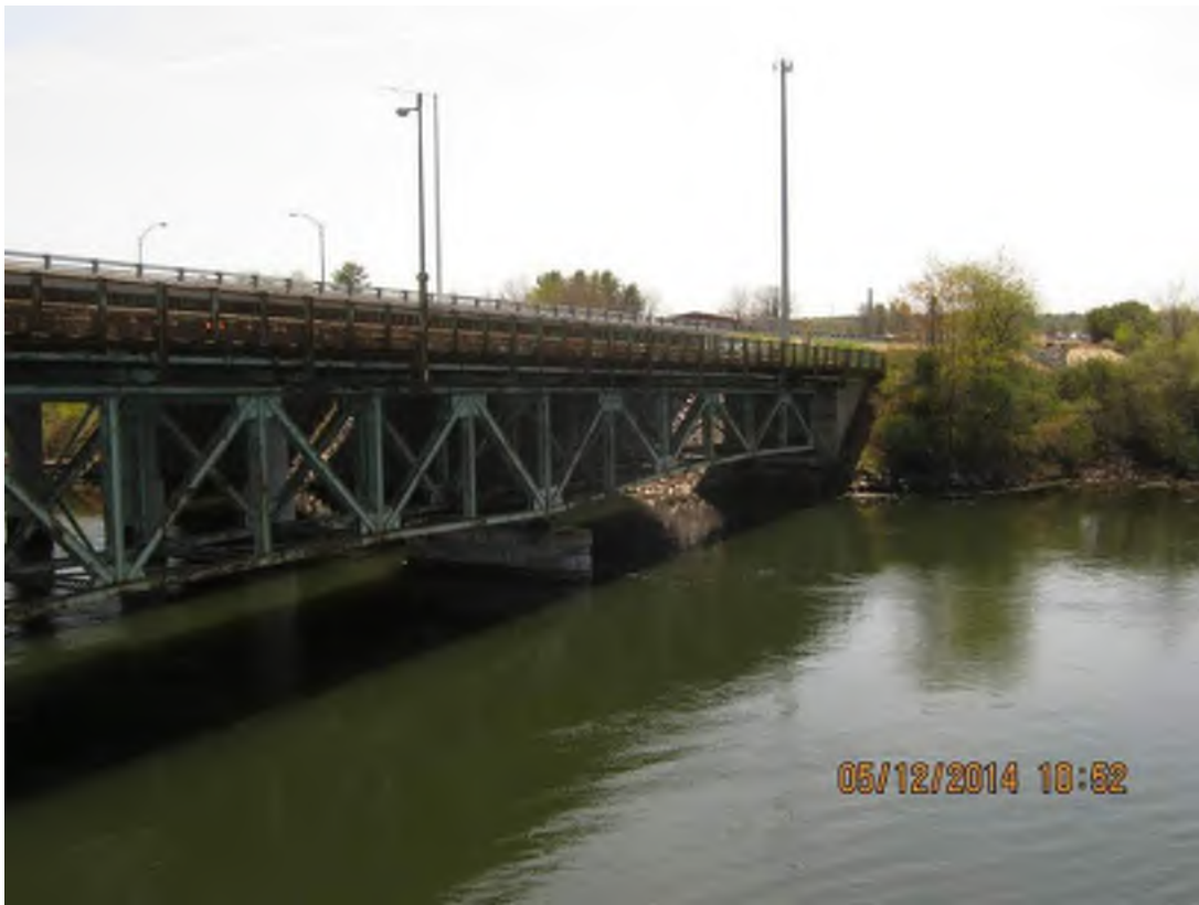
Photo 19: View south of the General Sullivan Bridge in Newington in the vicinity of one proposed temporary causeway (to right of bridge in the photo).
