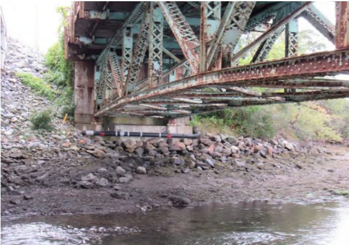
Photo 14: View south of the underside of the General Sullivan Bridge along the Newington shoreline.
