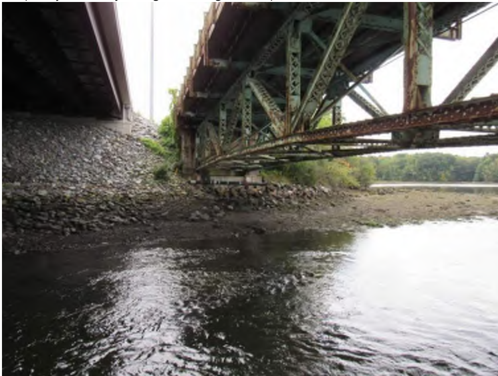
Photo 20: View south below the GSB in Newington in vicinity of one proposed temporary causeway (to right of bridge in the photo).
