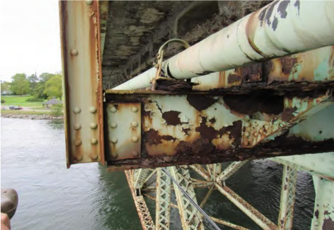
Photo 13: View north of corrosion and deterioration of the General Sullivan Bridge superstructure.
