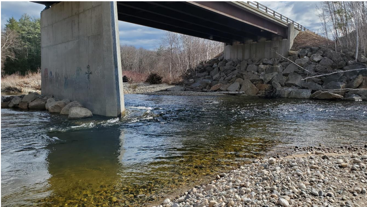
Figure 2. View of Pier I (the subject of this scour repair project). View is looking south.
