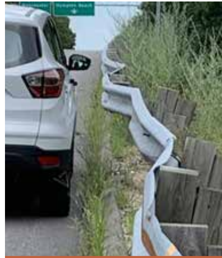
The Turnpikes Bureau also repaired or replaced 35 locations of damaged guardrail/terminals utilizing Statewide Contract, Betterment Funds, and the Operating Budget.
