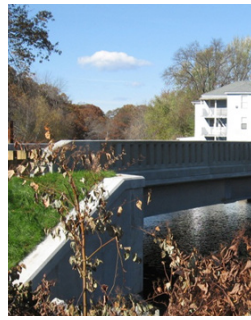
CHA designed the replacement of the bridge carrying Route 122 over the Blackstone River in Northbridge, MA using accelerated bridge construction techniques (ABC). The design also included an innovative excavation support solution to accommodate construction staging and utility constraints.
