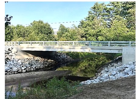
Two bridges on Stage Road in Gilmanton were bundled, creating design and construction efficiencies.
